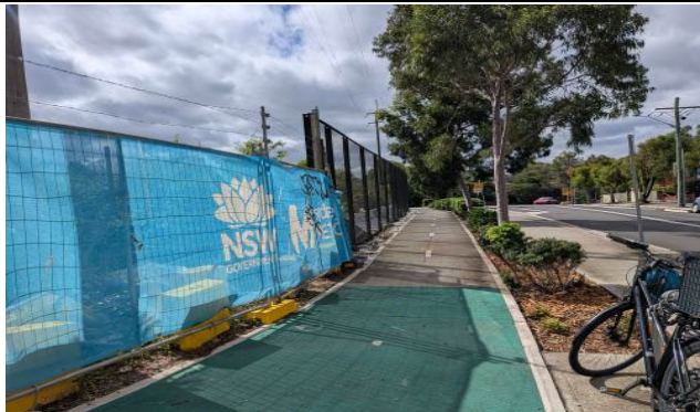
Figure 5 – Dulwich Hill - Steel barrier works planning ongoing, Martinus to avoid all impacts to TEC/PCT in this area as per recent discussions with SM and ER. Contractor Environment Manager to discuss the potential issues with the design and construction teams.
