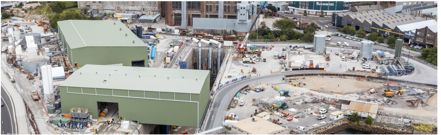
Two acoustic sheds have been removed from The Bays following the completion of tunnelling for CTP.
