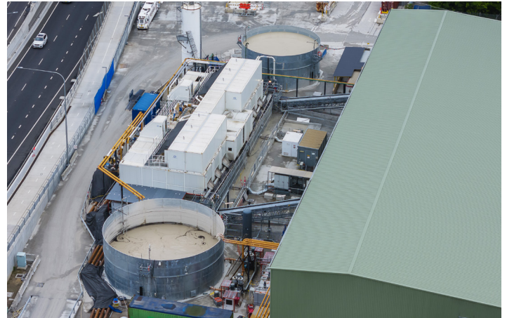
Aerial photo of the ETP TBM slurry treatment plant at The Bays site.
