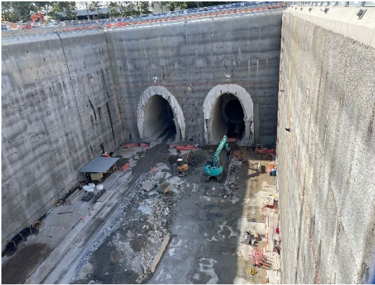
Figure 1.7 Station Box (SOP).
