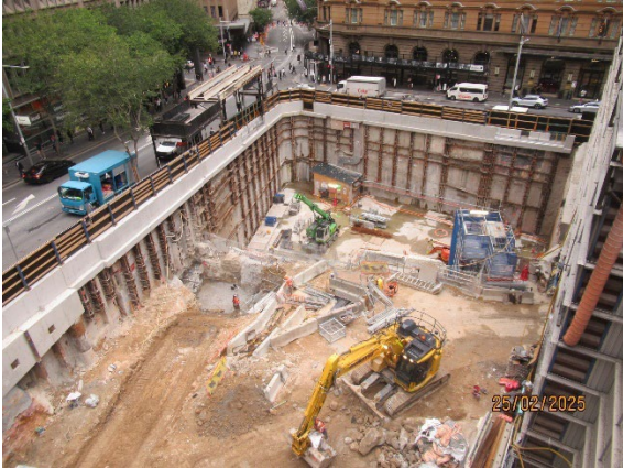
Figure 3.1 Hunter Street East: Works in the SW corner of the site including footing for the steel deck.
