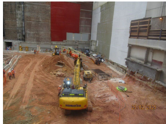
Figure 3.4 Hunter Street West: Water proofing works evident on adjacent building walls. Removal of spoil.
