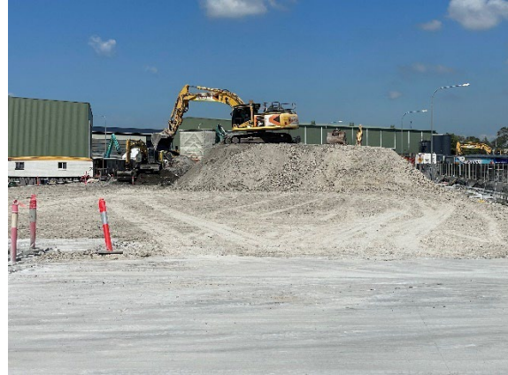
Figure 1.2 Crushed rock from the station box being used as backfill material to fill the void from the spoil shed slab. (The Bays).
