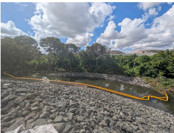
Figure 2.13 – Clyde MSF West: Northern Duck Creek Embankment Works –involving vegetation removal and rock scour placement.
