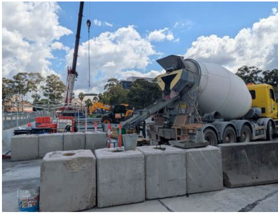
Figure 2.5 - SOP Site: Concrete truck set-up for delivery via drop pipe at SOP Station Box.
