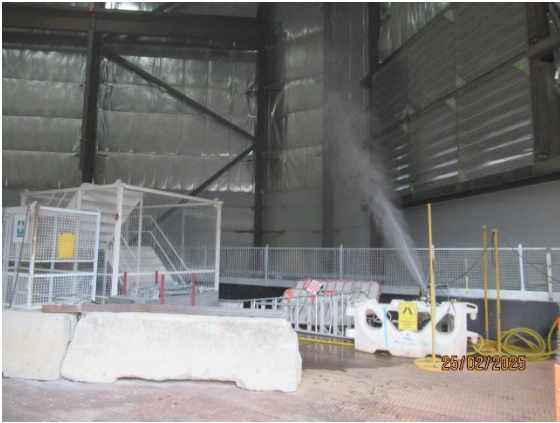
Figure 3.7 Pyrmont West: Mister in operation inside the acoustic shed.
