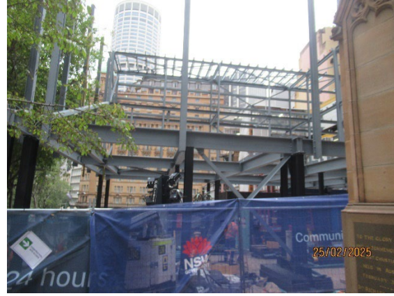
Figure 3.2 Hunter Street East: Installation of a metal frame for the crib sheds.
