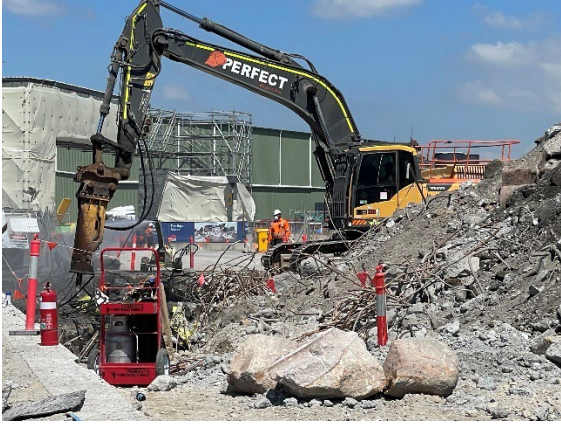
Figure 1.1 Removal of the final sections of the Spoil shed slab (The Bays).
