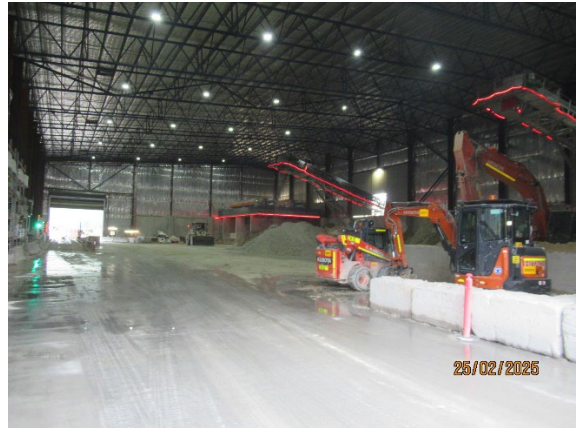
Figure 3.10 The Bays: Spoil management inside the acoustic shed.
