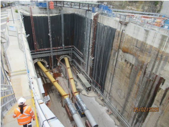
Figure 3.9 The Bays: Ventilation for the two TBMs in the tunnels.
