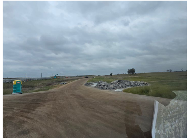
Portion 4 – Concrete storage and unbunded washout area. PLM arranged for a temporary bund to be installed, and it was suggested that storage be in a more suitable location.
