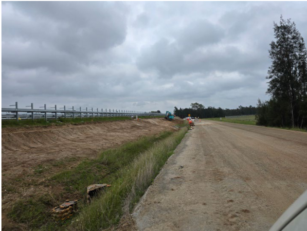
Luddenham to M4 – CST works had commenced. Additional ESC was required prior to upcoming rain.
