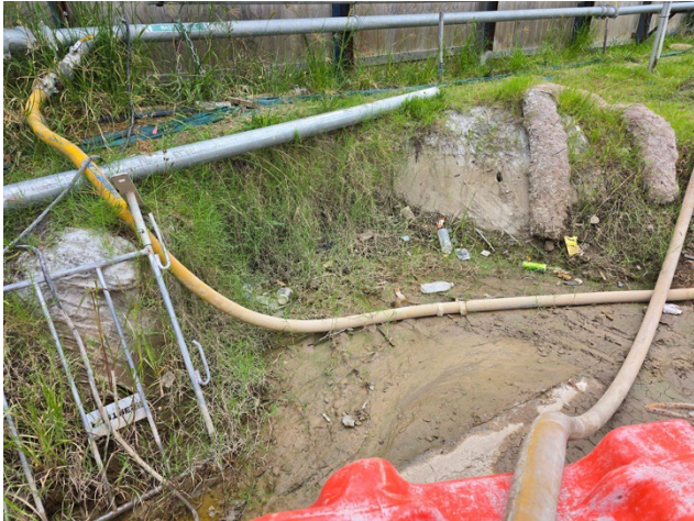
CMSF – It was noted that a pump sump filled with sediment and required cleaning.
