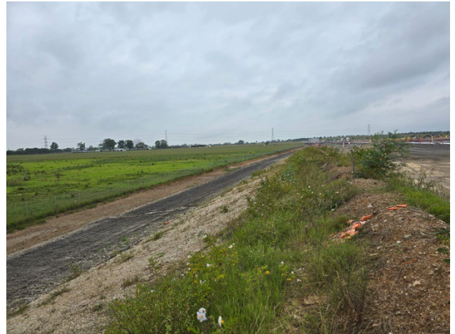
SMF – It was noted that weed spraying had occurred at the SMF, however some areas require additional spraying.
