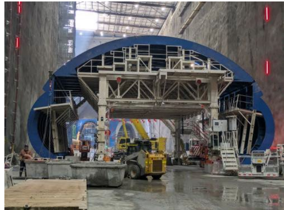
Figure 2.6 – Westmead Site: Euroform formwork assembly in the base of station box continuing.
