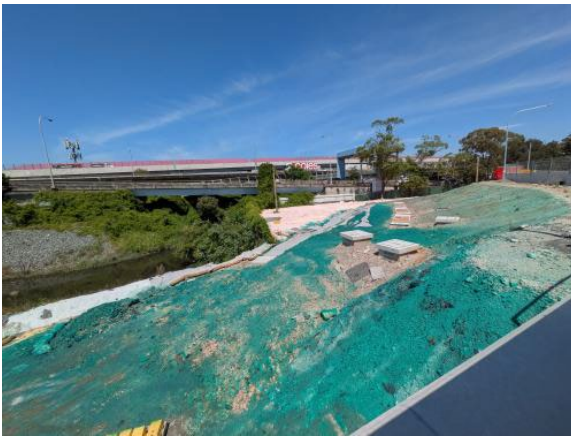
Figure 2.11 – Clyde MSF West: Finishing works and landscaping remains in Area 5, with polymer applied prior to Xmas Shutdown.
