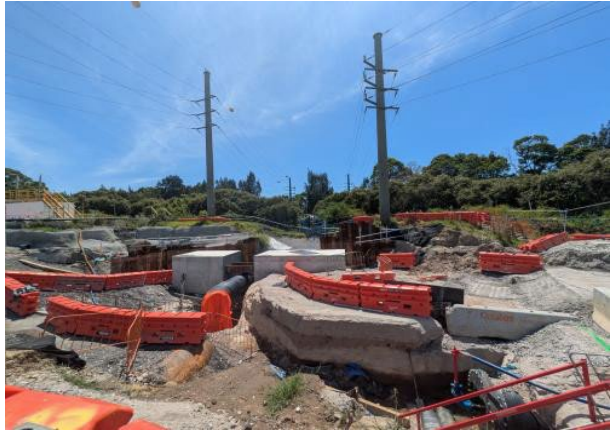
Figure 2.16 – Clyde MSF East: Sydney Water WM2 preparatory works for tie in and commissioning underway.
