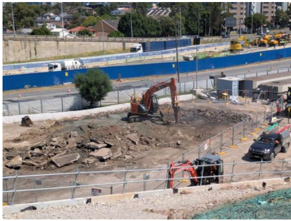
Figure 2.12 – Clyde MSF West: Hardstand breakout for future piling works for flood relief culvert. Dust suppression observed.
