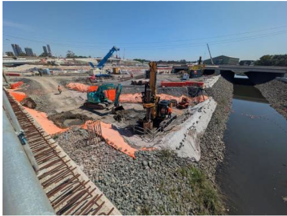
Figure 2.10 - Clyde MSF West Site: Piling works - near Duck Creek low flow channel.
