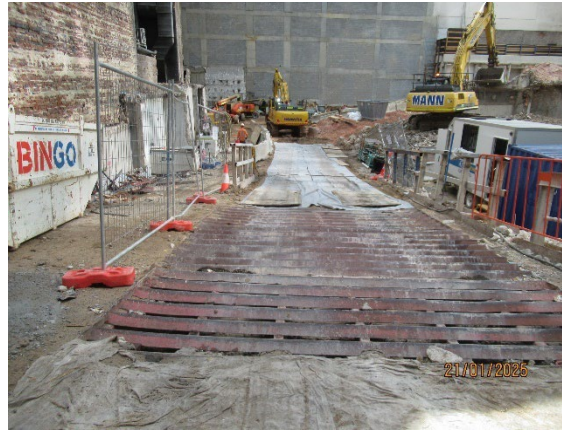
Figure 3.8 Hunter Street West: Access from Hunter Street with rumble grid. Ground stabilised with geofabric.
