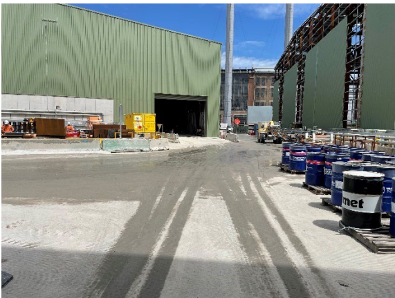
Figure 3.9 The Bays: Ongoing Water carts being used to wet down roads for dust suppression.
