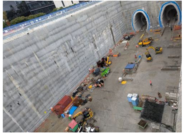
Figure 2.4 – SOP Site: Cross passage excavation works completed and spoil removed from previous spoil storage area within Station Box.
