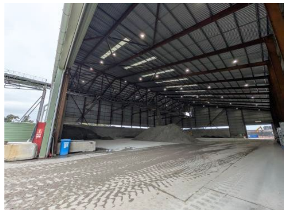
Figure 2.8 – Rosehill Site: Spoil stockpiling within shed and spoil movements internally only (to MSF).
