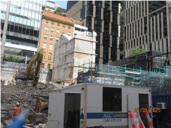
Figure 3.7 Hunter St West: Removal of buildings and spoil from around Skinner's Hotel.
