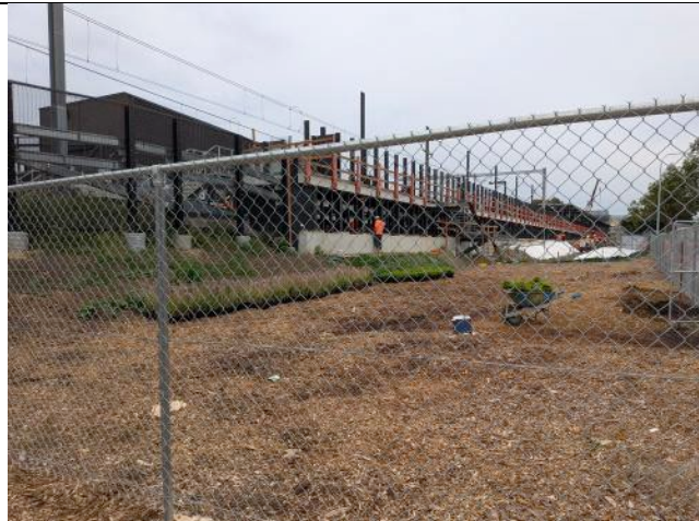
Figure 7 – Bankstown Station - Non-JHLOR works related to stormwater upgrade in the vicinity of Bankstown Station nearing completion (Council works), landscaping in progress.
