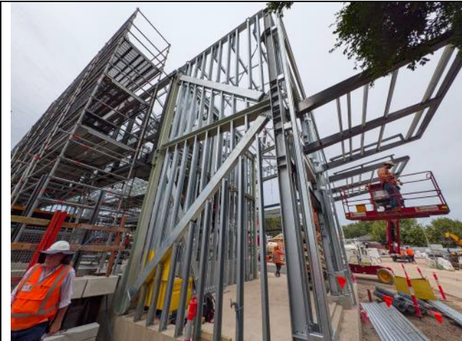
Figure 9 - Bankstown Station - Steel installation works for the Sydney Metro building area nearing completion.
