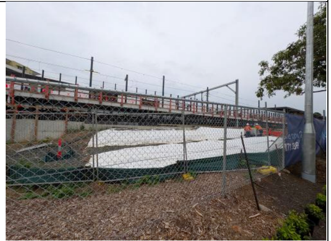
Figure 8 – Bankstown Station - Culvert backfilling completed, geofabric on the embankments and silt fence in low points in place.
