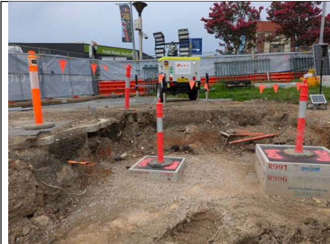
Figure 13 – Bankstown Station - Backfilling of the areas around Metro Building and combined services routes installation ongoing.
