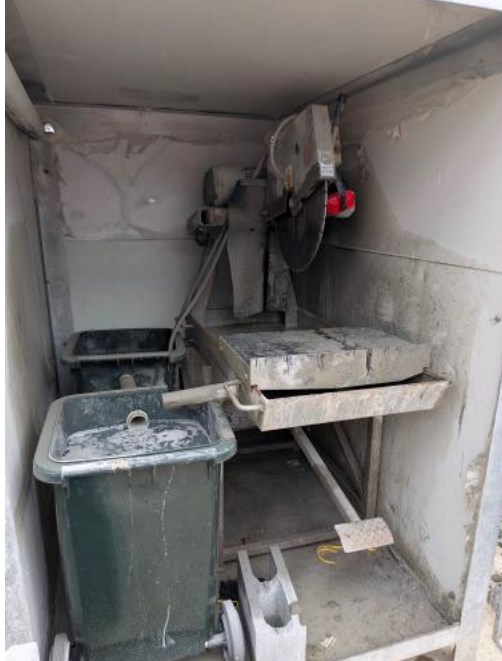
Figure 11 - Bankstown Station - Brickwork and block work ongoing. Concrete cutting station was established on site to capture concrete cutting slurry and minimise concrete saw noise - good practice.
