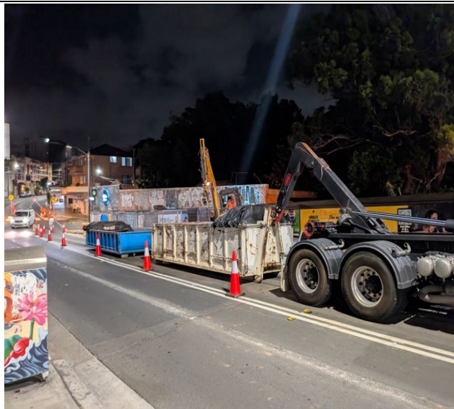
Figure 5 – Illawarra Road, Marrickville – Footpath excavation in progress, spoil being transferred to skip bins.
