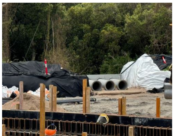
Figure 2.14 – Clyde MSF East Site: Biobasin outlet in the process of being constructed.
