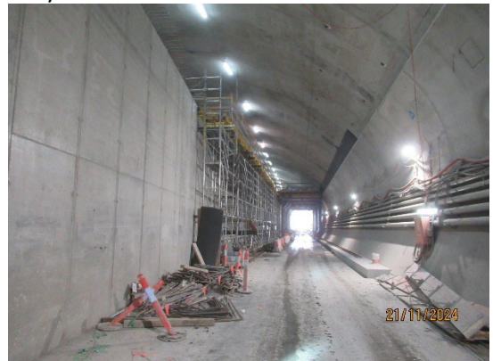
Figure 1.4 Cavern and plenum (Burwood North).
