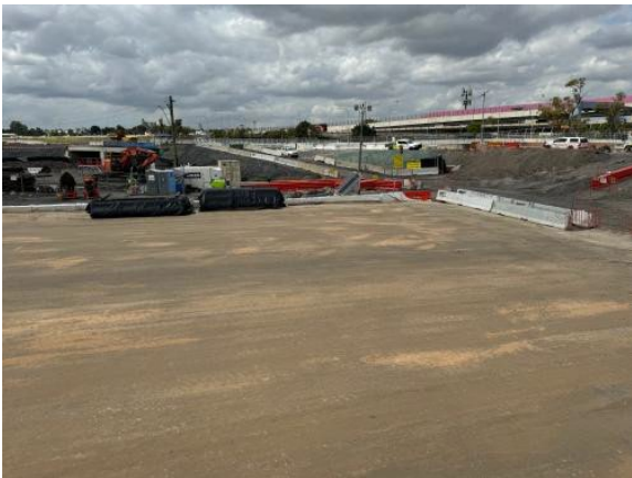
Figure 2.11 – Clyde MSF West Site: Geo synthetic liner to be placed across the LTP . GLC reports Contamination Site Auditor in attendance to observe proposed process.
