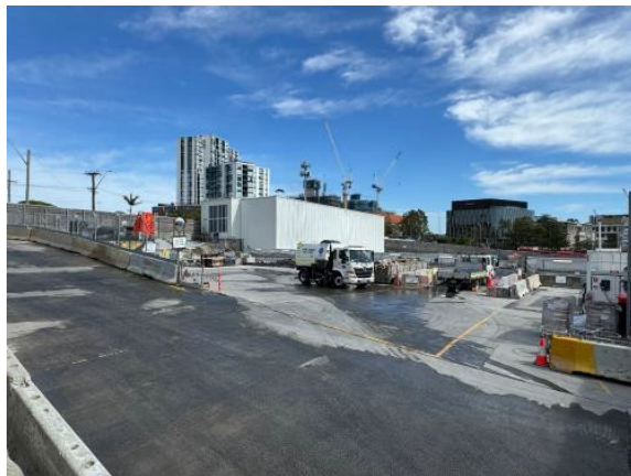
Figure 2.8 – Westmead Site: Internal site access wet down on a very hot day, to mitigate dust (29degrees at 9am).
