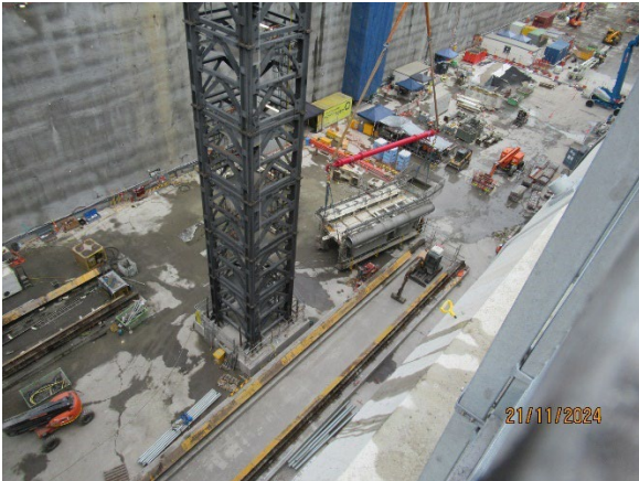
Figure 1.7 Lift out of TBM plant from the station box using the tower crane (SOP).
