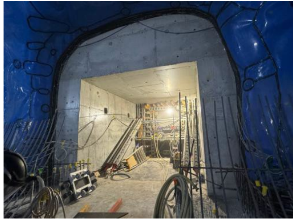
Figure 2.4 – Westmead Site: Ongoing FRP for Stub Tunnel invert slab and Cross Passages walls.
