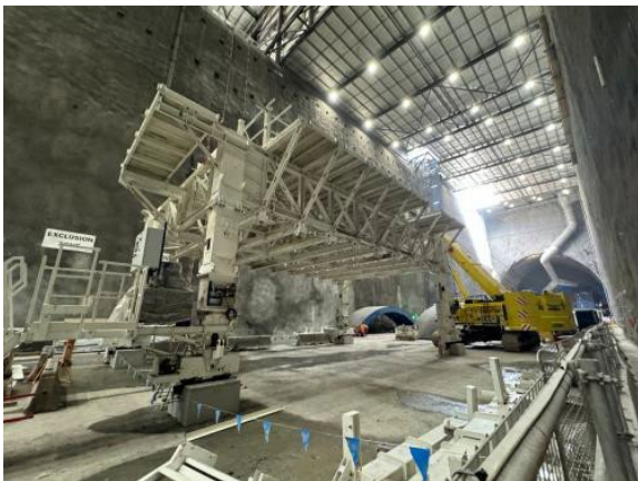
Figure 2.7 – Westmead Site: Ongoing build of the Euroform Formwork gantry. Curved form sections still to be added.
