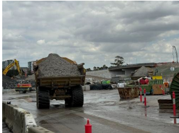
Figure 2.10 – Rosehill Site: Spoil movement kept internal at the moment, with re-use of tunnel spoil amongst works at the MSF.
