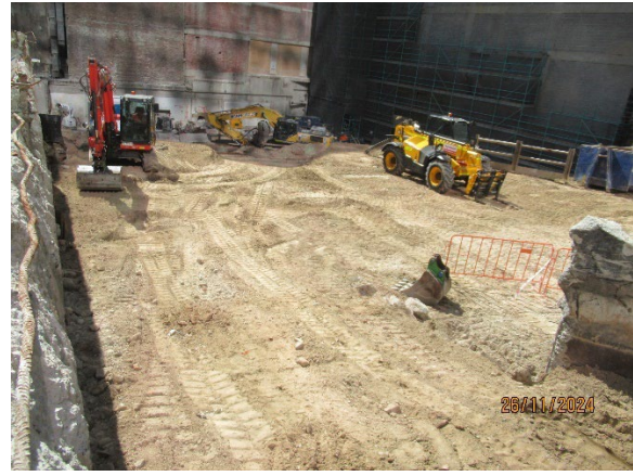
Figure 3.8 Hunter Street West: Demolition and other works recommenced after completion of Archaeological Excavations adjacent the former De Mestre Place.
