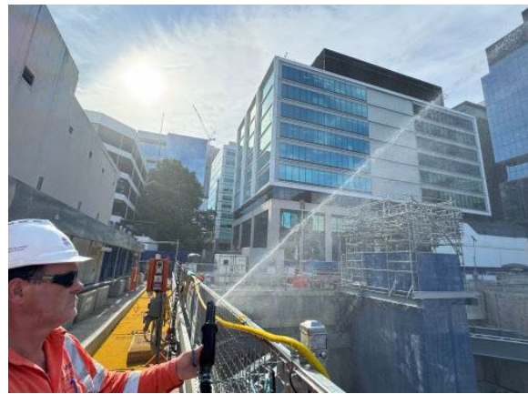
Figure 2.2- Parramatta Site: Dust management at Station Box from the numerous misters / sprinklers in use.
