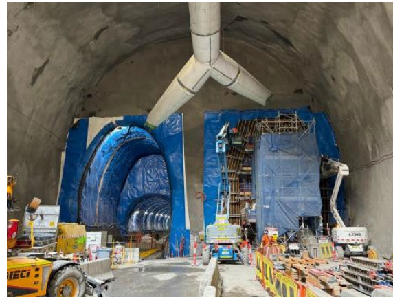
Figure 2.6 – Westmead Site: Nozzle formwork and pours ongoing at the western end of the Station Box.
