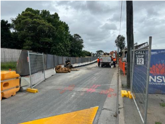
Figure 2.9 – Clyde MSF: Unwin St Southbound works within work area bordered by noise blankets.
