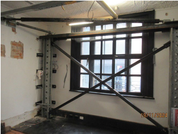
Figure 3.7 Hunter St West: Temporary Structural support and crack monitoring/wall support across crack at Skinner's Hotel.
