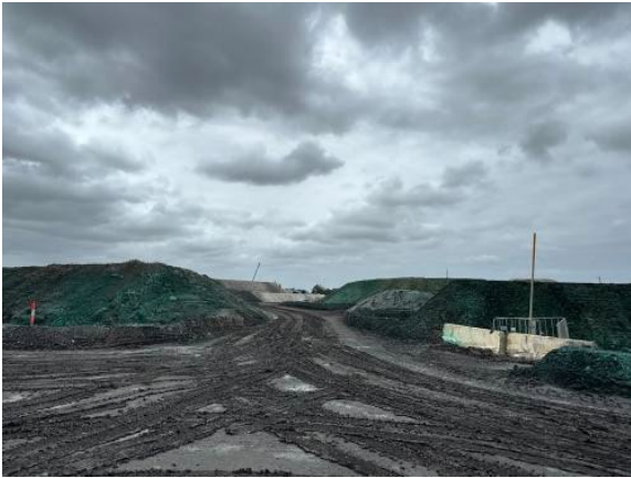
Figure 2.9 – Clyde MSF East: Spraying of stockpiles had commenced in preparation for Christmas Site Shutdown.
