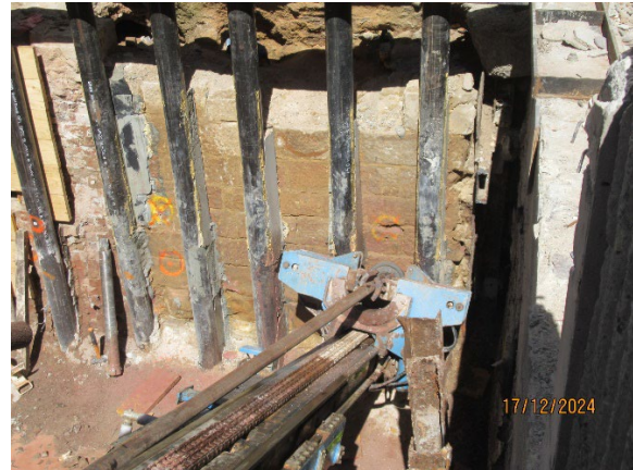
Figure 3.8 Hunter Street West: Rock Anchors being placed in Heritage wall adjacent George Street after recoding by heritage consultants.
