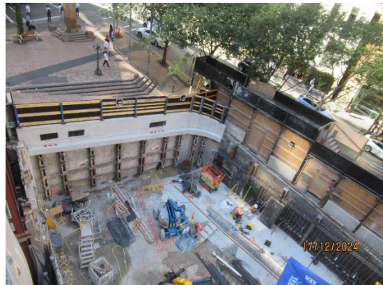
Figure 3.6 Hunter Street East: Barrier and A class hoarding installed adjacent Richard Johnson Square.
