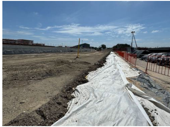
Figure 2.6 – Clyde MSF: GSL placement over Load Transfer Platform material. GLC reports Site Auditor has re-visited activity to witness layers and process.
