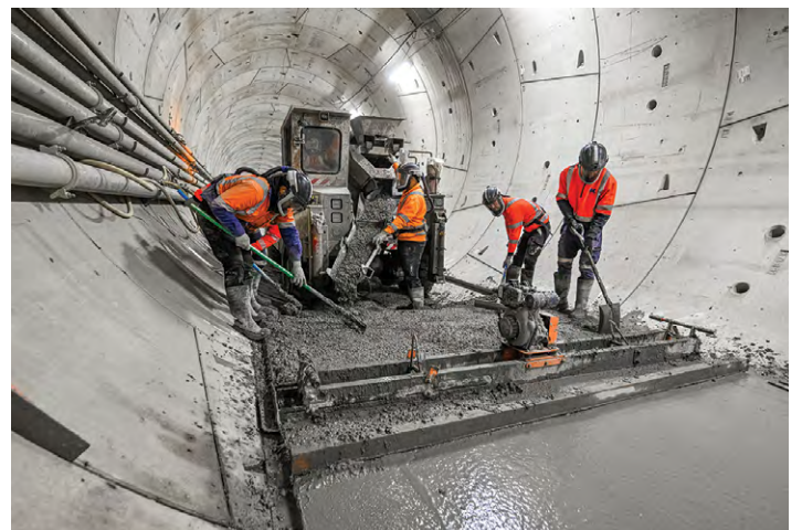
A concrete floor being poured in a tunnel north of the Orchard Hills Station site.
