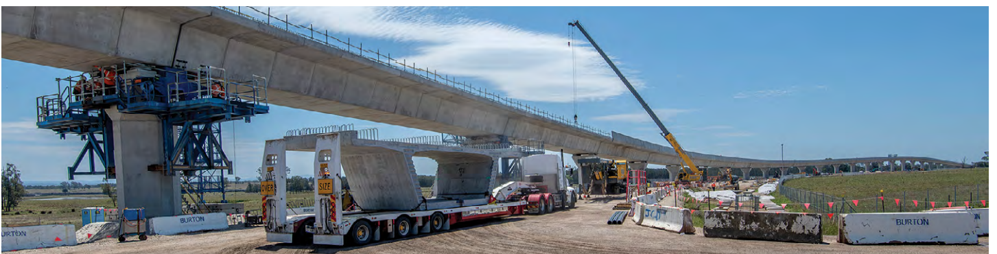
The SCAW team has successfully delivered and erected all 1101 precast segments for the viaducts.
