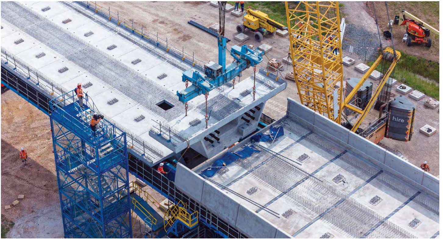
The placement of the final segment to complete the viaduct installation for the project.
