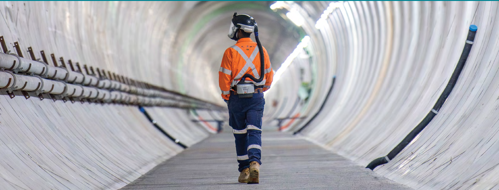
A section of the completed twin tunnels between the Airport Terminal and the Bringelly Services Facility.
