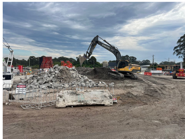
Claremont Meadows: Ramp material is being removed via the shaft and loaded out
