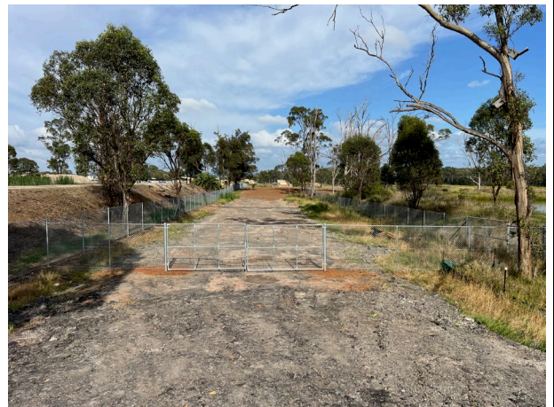
Bringelly: The back laydown area has been handed back to Sydney Metro
