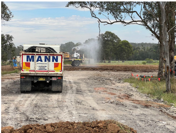
Bringelly: The ACM stockpile was spread and inspected prior to being hydromulched
