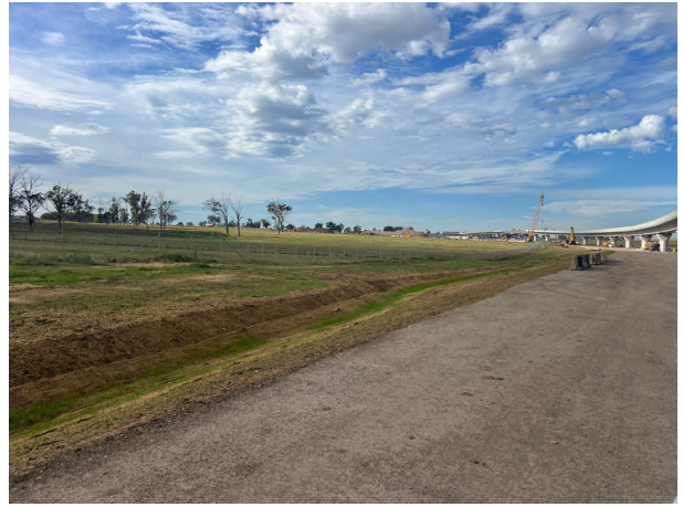
Luddenham North: The perimeter drainage line has been stabilised with jute mat and hydromulch
