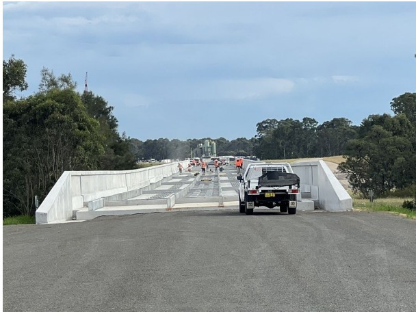
Blaxland's Creek: Additional grinding works occurred on the bridge with a vacuum used to contain the dust
