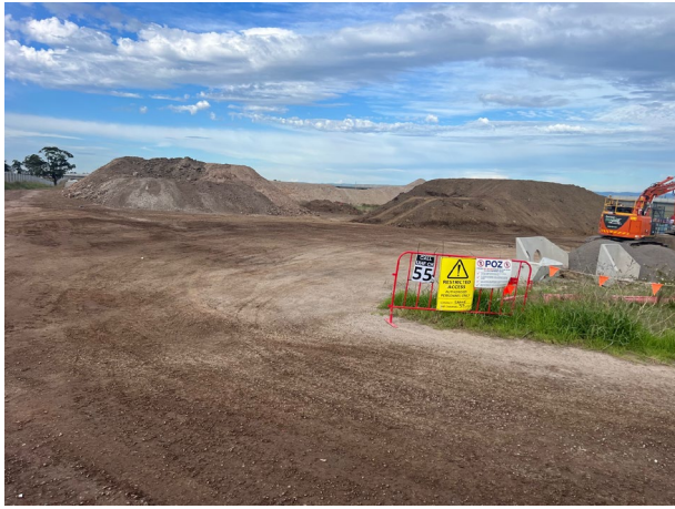
Luddenham North: VENM and topsoil are being stockpiled to be reused on the project
