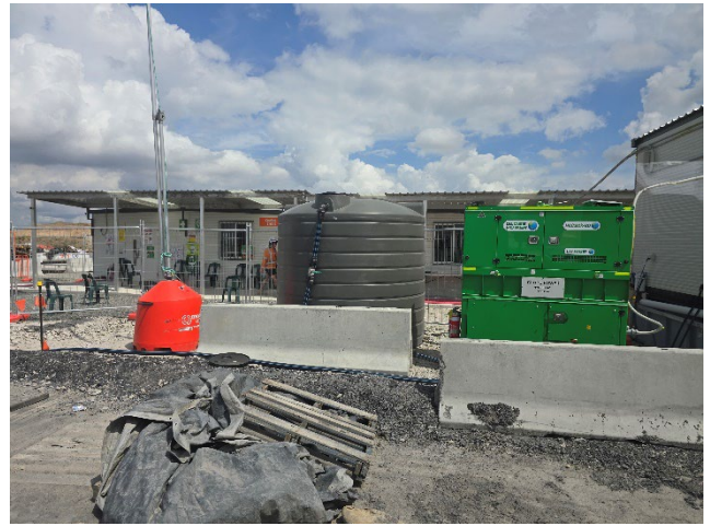
SMF – Noted hybrid generators are being used onsite
