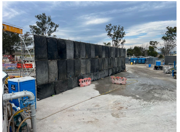
Bringelly: The noise wall was in place to allow for OOHW concrete pours
