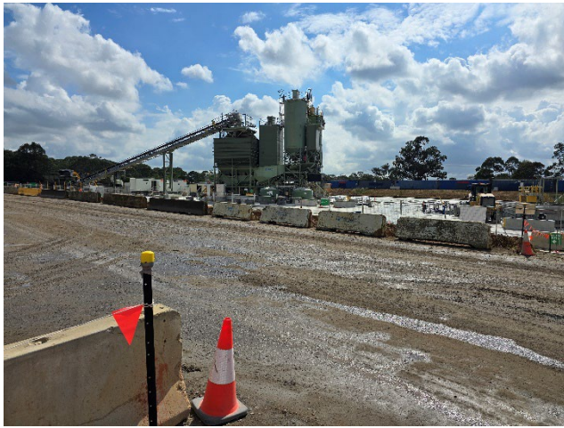
ORH – Concrete batch plant
