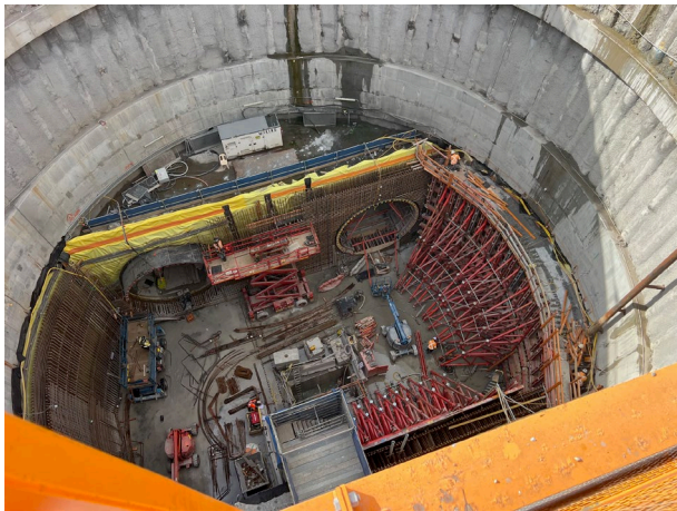
Bringelly: Three main concrete pours remain for the completion of this shaft
