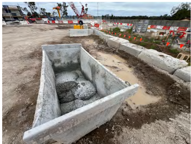
Bringelly: The concrete washout area was no longer required; it was suggested a bin remain on site in case unforeseen concrete works occur.
