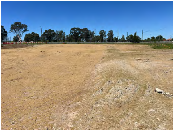
Claremont Meadows: Equipment is being progressively lifted out of the tunnel shaft.
