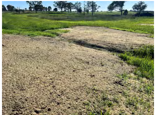
Defence: Minor disturbed areas were stabilised via hydromulch prior to the shutdown.
