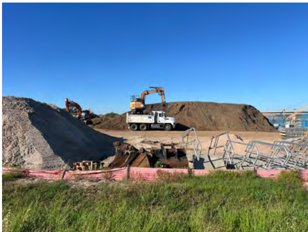
Luddenham North: The stockpiles were shaped and sprayed with polymer prior to shutdown.
