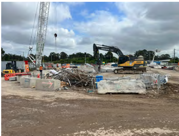
Claremont Meadows: Material from the tunnel was separated into recyclable and waste stockpiles.
