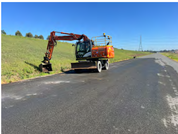
Patons Lane: Rework was observed to be tidy and controlled along the Patons Lane batter.
