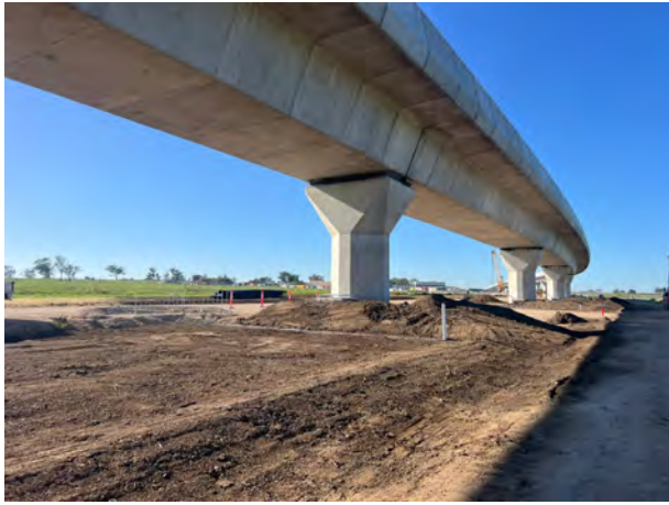
Luddenham North: Topsoil was applied underneath the viaduct in preparation for hydromulch.
