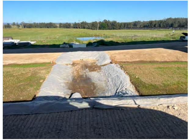
Luddenham North: The cross drainage was in appropriate condition for the shutdown.
