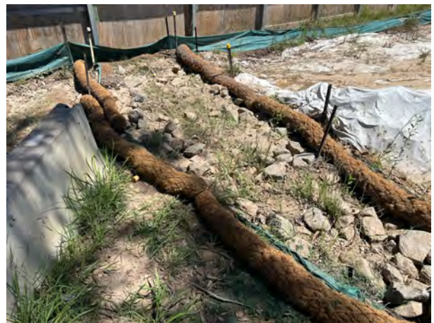
Claremont Meadows: ERSED controls were refreshed prior to the shutdown.
