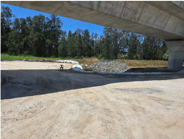
Portion 3 – ESC prior to discharge under via duct adjacent to Cosgroves Creek.
