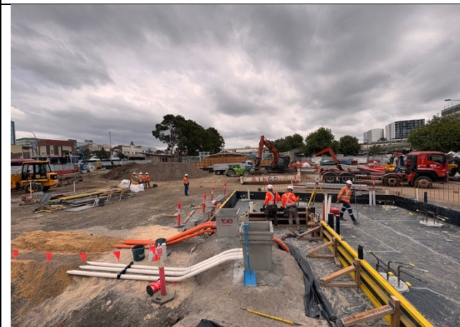
Figure 9 – Metro Service Building works including services installation and formwork in progress followed by concrete pours
