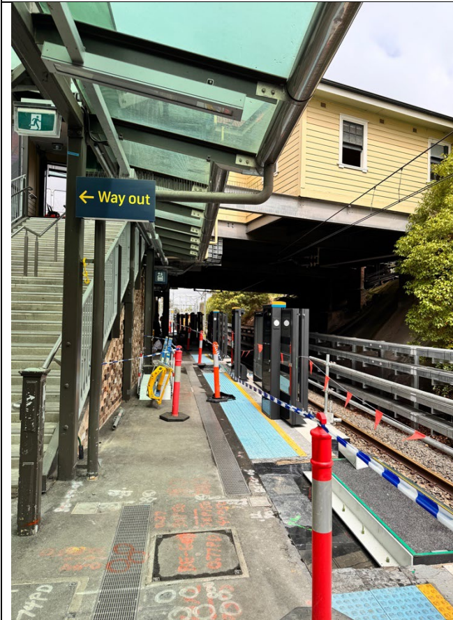
Figure 13 – Belmore Station – Platform Screen Doors and Mechanical Gap Fillers being installed on the platforms
