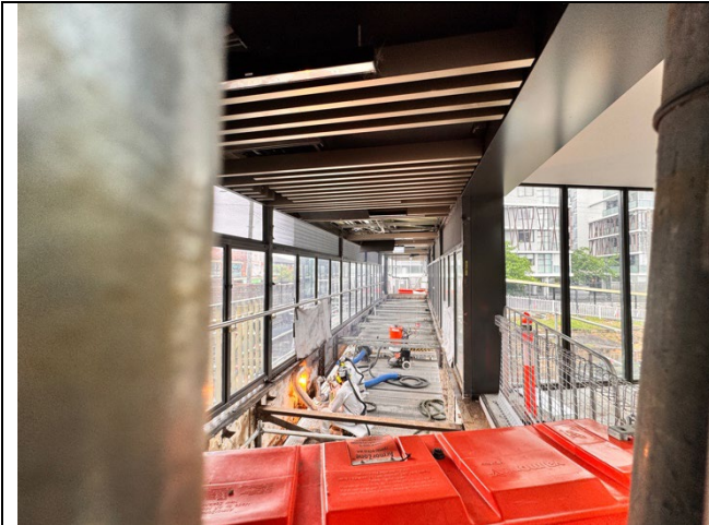
Figure 11 – Canterbury Station - Lead paint removal in progress using laser and vacuum extraction
