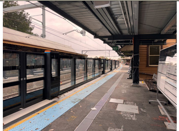
Figure 2: Marrickville Station – Platform Screen Doors installed
