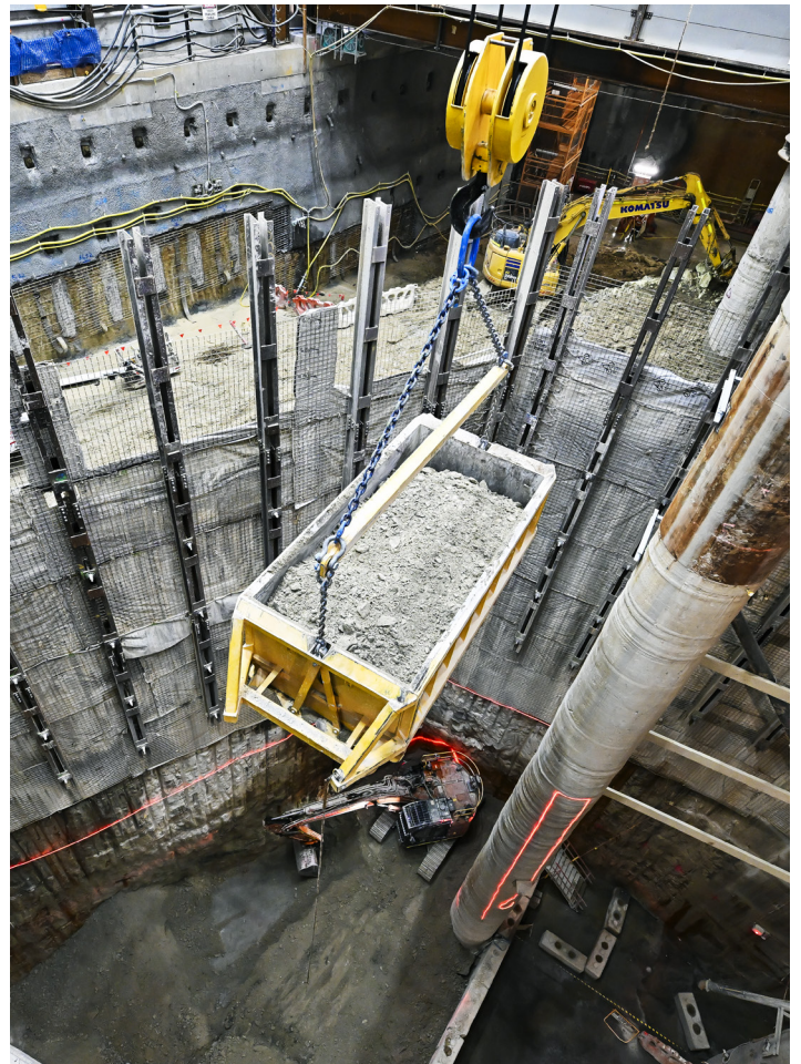
Excavated material is removed from the cavern and loaded into trucks to be taken offsite.
