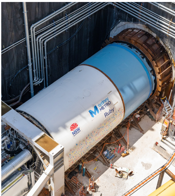
TBM Ruby launched from The Bays Station site and is now on its way to Pymont.
