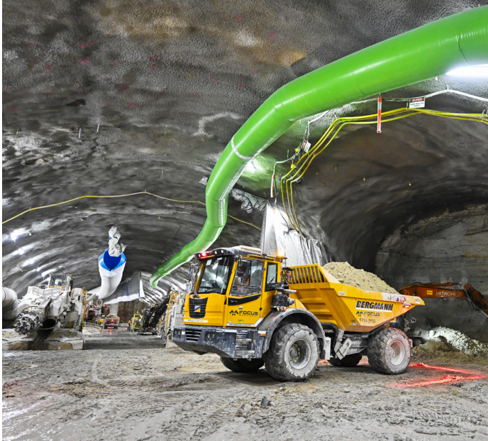
A total of 312,000 tonnes of spoil will be excavated in the cavern and associated tunnels at Pymont Station.
