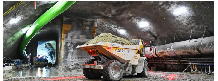
The station cavern will be 18 metres high, 24 metres wide and 170 metres long.
