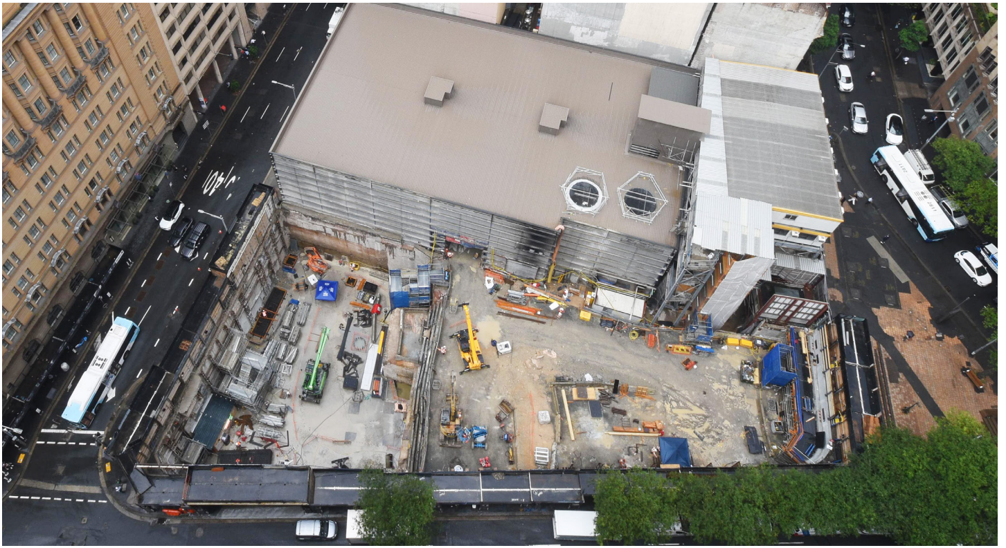
Site establishment works for shaft excavation are continuing at the Hunter Street East site.
