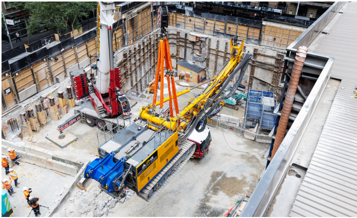
A 400 tonne crane lifts a large piling rig into the shaft during a complex engineering exercise at the Hunter Street East site.
