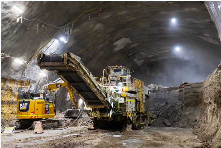
The Hunter Street Station cavern is 28 metres wide, 20 metres high and will be 180 metres long.
