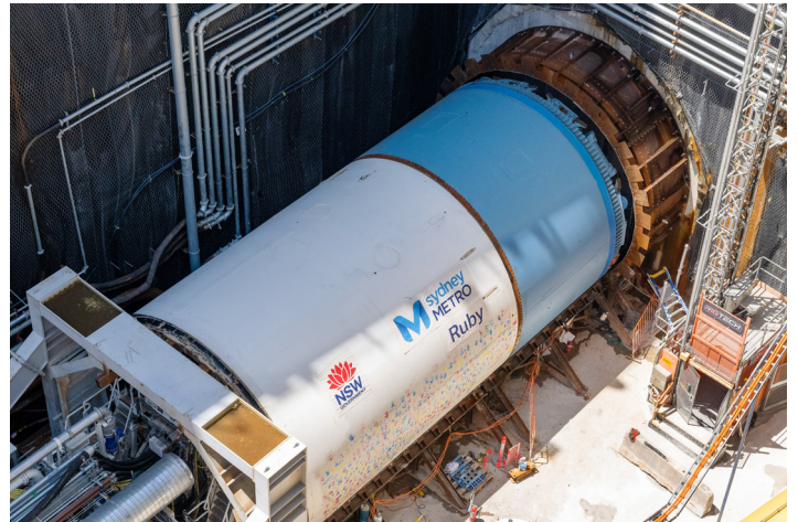
TBM Ruby launched from The Bays Station site and is now on its way to Pyrmont.
