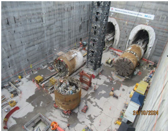
Figure 1.7 TBM in the station box. Disassembly activities using the tower crane (SOP).
