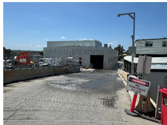
Figure 2.8 – Westmead Site: Sprinklers on driveway to manage dust and cleanliness of truck wheels.
