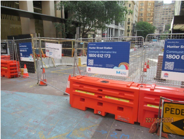
Figure 3.7 Hunter St West: Signage for road closure of Hunter Street. Hoarding under construction.
