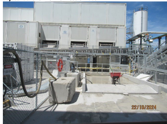
Figure 3.10 The Bays: Slurry Treatment Plant.
