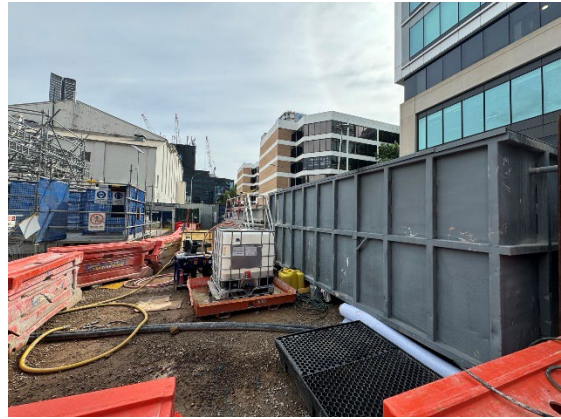
Figure 2.4 – Parramatta Site: Settlement tank adjacent to Station Box, to assist with removing sediment load before pumping to WTP.
