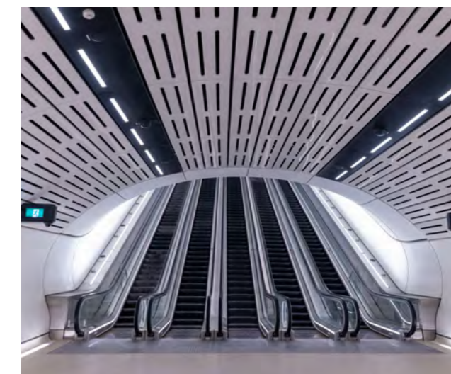
Image: The internal acoustic insulation at Victoria Cross station is made from up to 80 per cent recycled PET plastic packaging such as drinking water bottles.
