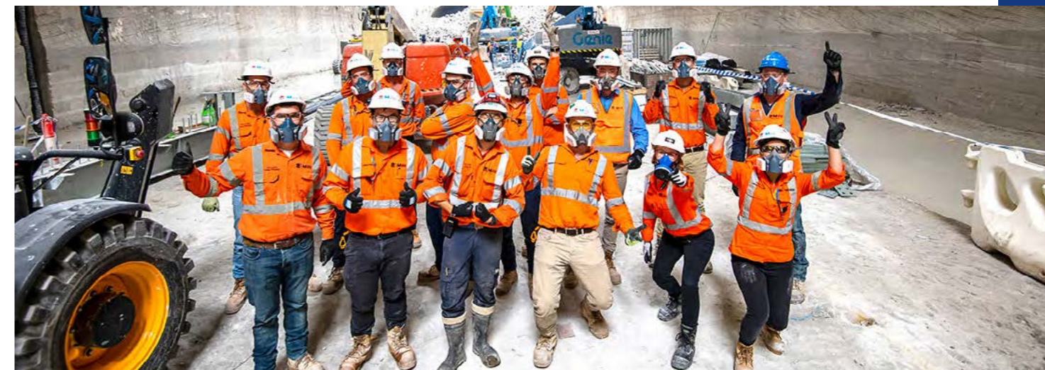
Image: Masks are a must when working below ground. Central team in the metro box, February 2021.
