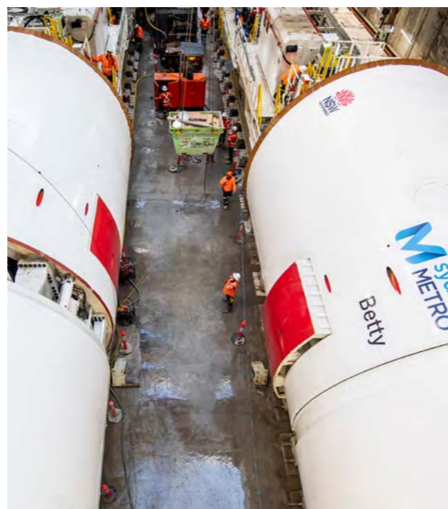
Image: TBM Betty has begun its journey from Rosehill to Sydney Olympic Park, the first part of twin nine-kilometre tunnels from Sydney Olympic Park to Westmead.
