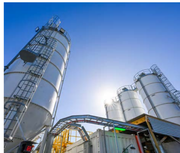
Image: The purpose-built water treatment plant at Rosehill that supplies all Tunnel Boring Machine operations with treated groundwater.
