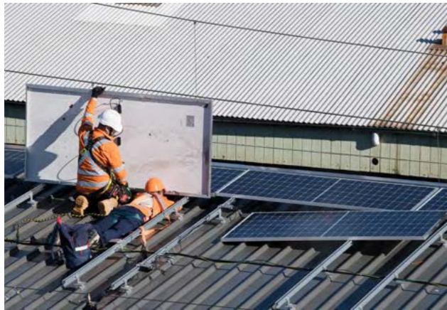
Image: The renewable energy generated from the 664 solar panels at Central Station will power lights across three platforms and will lower the electricity demand at the station by 10 per cent.
