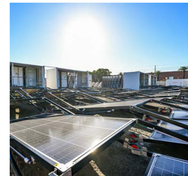
Image: A rapidly deployed mobile solar farm powers the Tunnelling Infrastructure Academy at Rosehill.
