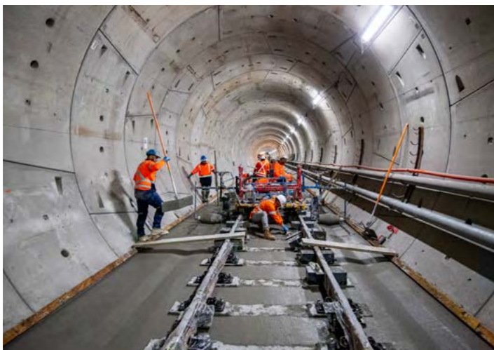
Image: A concrete pour inside the tunnel between Chatswood and Crows Nest.
