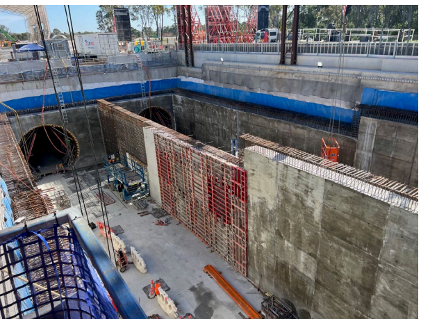
Orchard Hills – Works continue in the dive, with a partition wall being constructed
