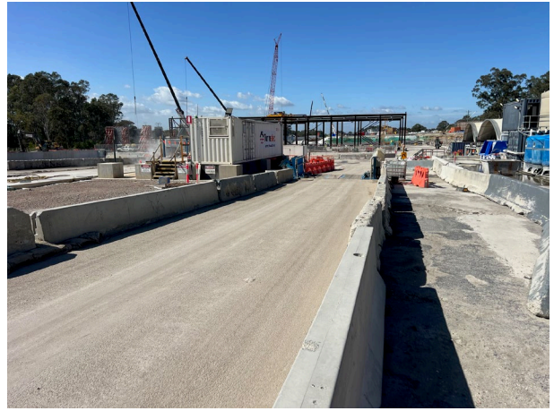
Orchard Hills – The wheel wash was decommissioned, mud tracking will need to be monitored and removed via alternative means
