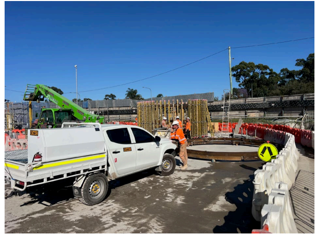
Claremont Meadows – The NW corner is now being used for construction forms, concrete pumping has been relocated to the other side of the shaft
