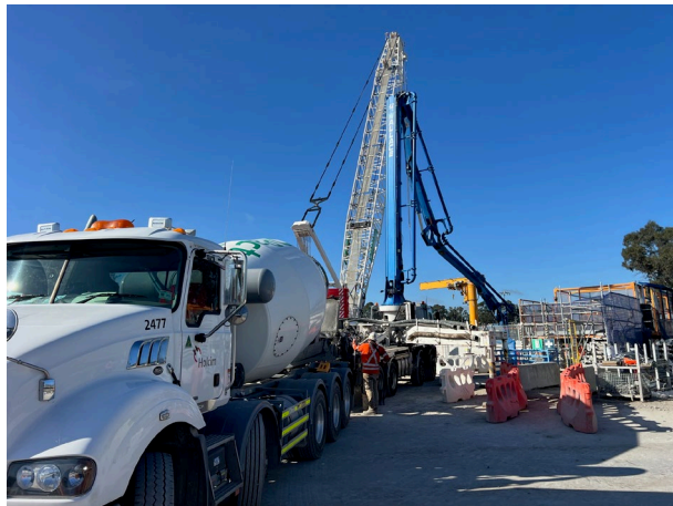
Claremont Meadows – Concrete pours continued down the shaft, washout facilities were present
