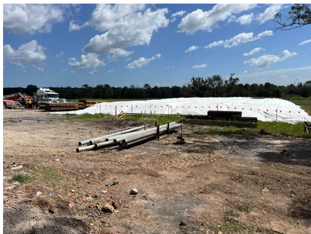
Bringelly – The ACM stockpile has been approved to be respread over the existing laydown area
