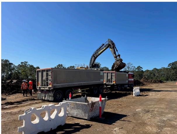
Orchard Hills – Topsoil was loaded out from the site, the S143 process has been implemented
