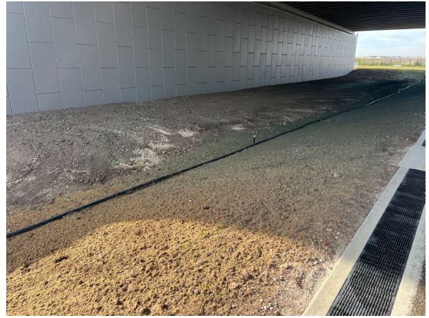
M12 Bridge – The revegetation under the M12 bridge is showing limited signs of success, the ER has requested that the contractor discuss this with Sydney Metro
