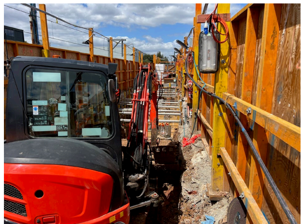
Platform 1/2 - Water was held in the excavation on platform 1/2 and was pumped to a water cart for disposal
