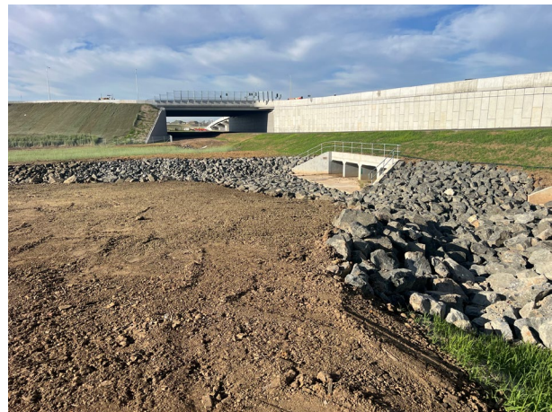
M12 Bridge - The main culvert has been finalised and the surrounding catchment stabilised
