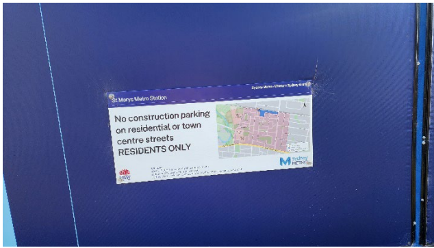
STM – Site parking signs
