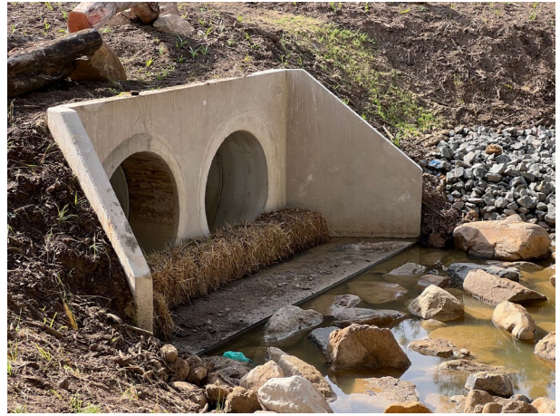
Defence - Hay bales have been placed across the culvert in Unnamed Creek.
