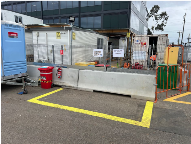
Compound - A dedicated refuelling area has been provided following recent spills
