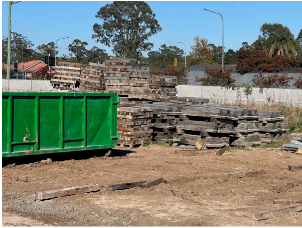
Claremont Meadows – Waste timbers from the site storage area are to be given to organisations who will reuse or repurpose them
