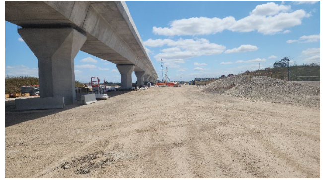
LUD – Laydown areas were maintained. A minor oil spill was observed and cleaned during the inspection
