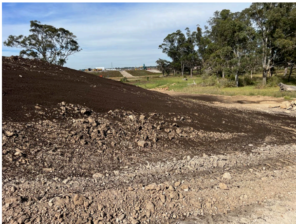
PS105 - Organic rich material is being applied to PS105 as per the requirements of the RAP
