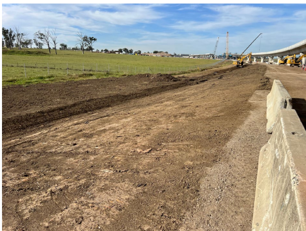
Luddenham North - The batters are being shaped with topsoil in preparation for the application of hydromulch
