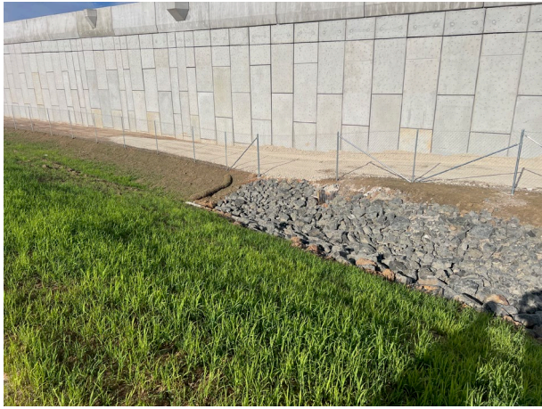
M12 Bridge – The drainage line adjacent to the M12 is in good condition with scour protection
