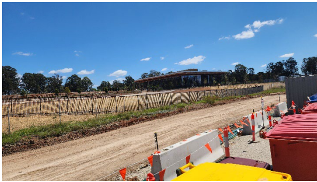
BFD – backfilling of the clean water diversion and preparation for new road access
