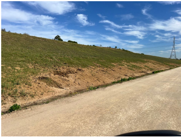
Patons Lane - Areas of failed revegetation remain along the batters adjacent to Patons Lane
