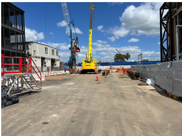
Compound – The hardstand area had a fine layer of dust, the contractor stated that a sweeper is used to clean this at the end of each day. ER requested records
