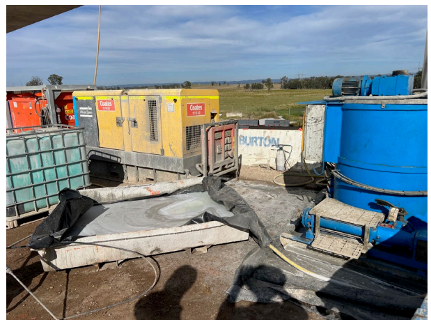
Luddenham North – Grout has spilt outside of the containment structures. ER requested a cleanup and evidence of additional containment
