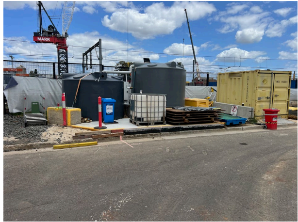
Compound – The water recycling area was clean with all materials properly stored
