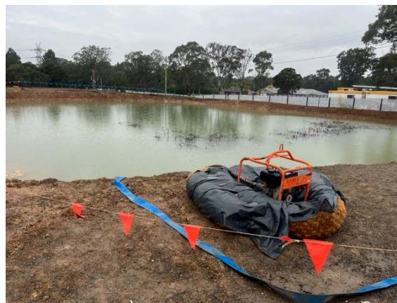
Photo 24: SE Sediment Basin – Water collected from across the site is pumped via rock-lined channels to the M7 Sediment Basin prior to discharge to Blaxland Creek via the EPL licenced discharge point. NB: There was no access to the M7 sediment basin during the audit due to wet weather WHS restrictions.
