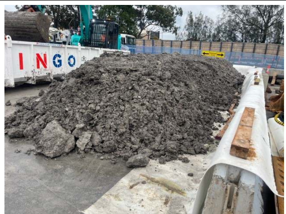
Photo 8: Stockpiled VENM excavated for station box sump in designated bay. No tracking or sediment on surrounding hardstand observed.
