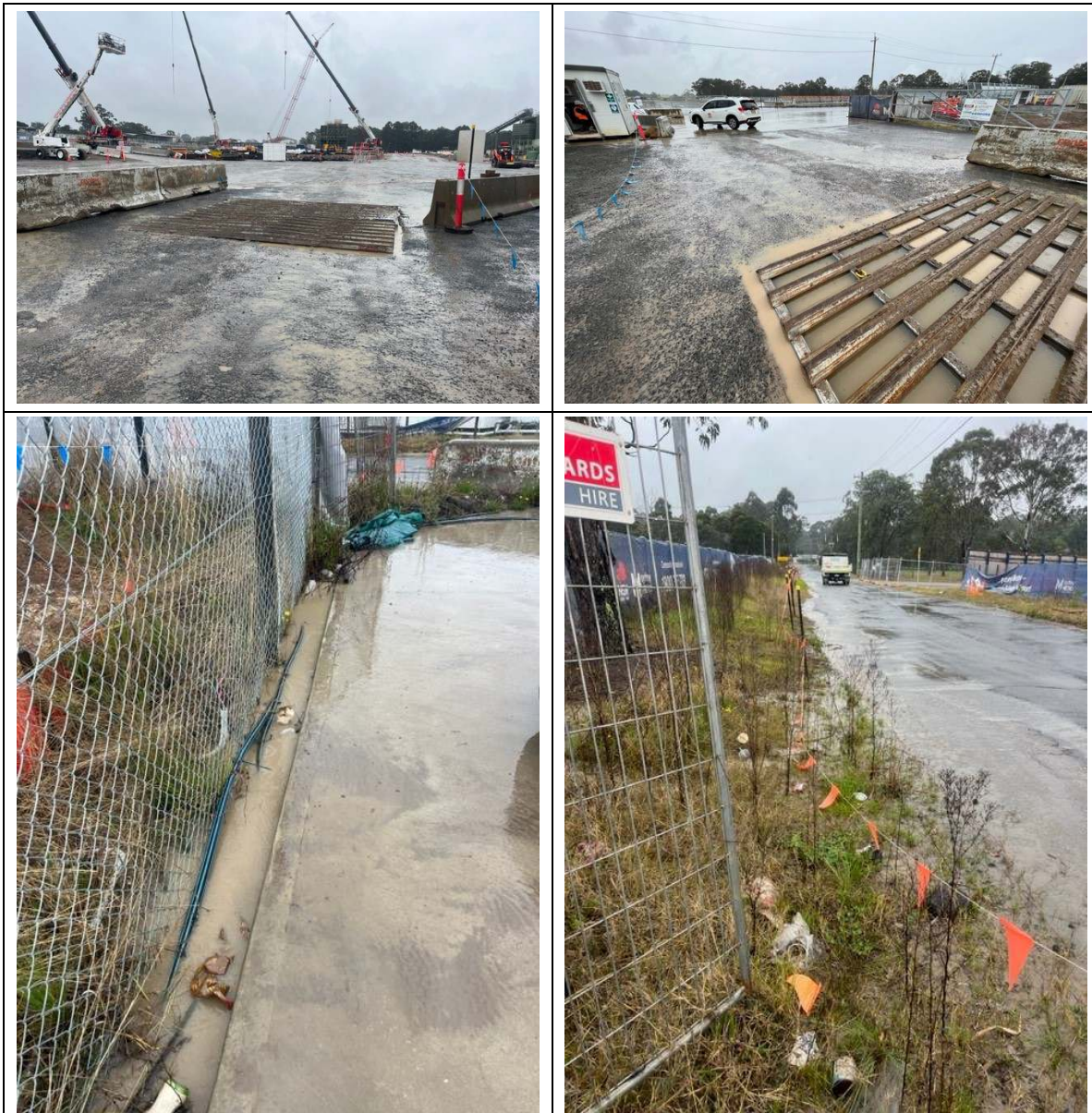
Photos 25-28: The cattle grid at the Heavy Vehicle access onto Lansdowne Road was filled with sediment-laden water, which was flowing through deteriorated controls onto the nature strip and down the road. Stormwater inlets were not observed due to no kerb and gutter. Refer to Attachment 1, Condition 128 for recommendations.
