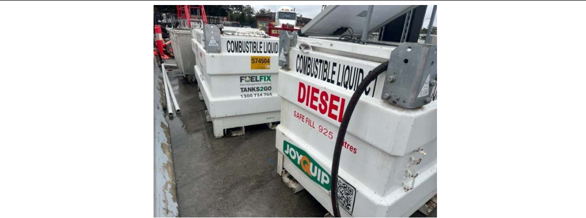
Photo 7: Compliant diesel storage (labelled and self-bunded) for tower cranes
