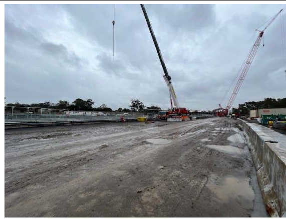
Photo 20: Internal haul roads were muddy and further stabilisation measures should be applied to reduce the risk of tracking (it is noted that works were on hold at the time of the audit due to wet weather)
