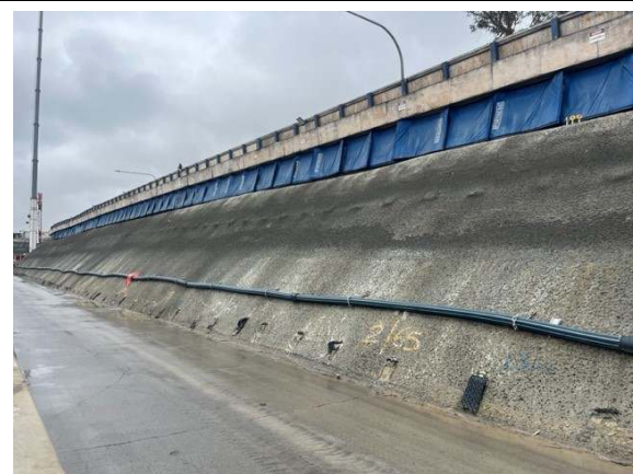
Photo 9: Noise blankets installed at top of batter on hoarding to reduce noise impact to surrounding residents.
