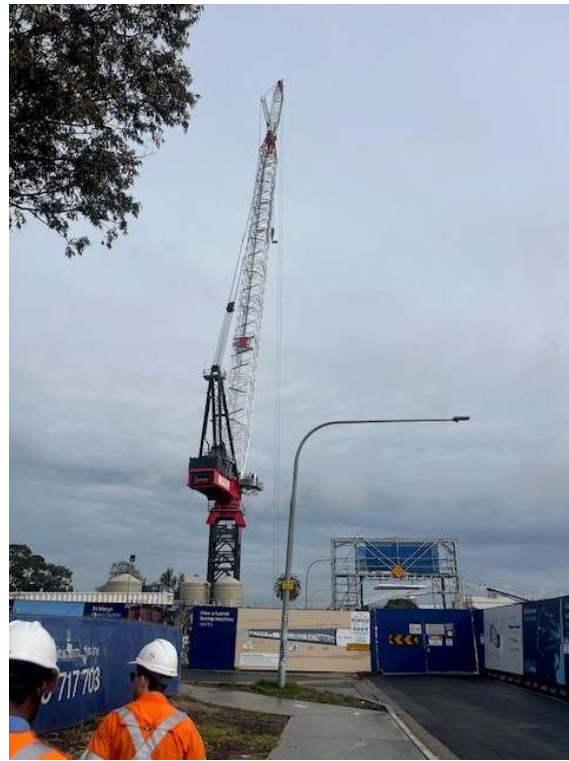
Photo 1: A tower crane had been set-up at St Mary's. As a result of a noise assessment, shrouding for the crane had been ordered to reduce potential impacts to surrounding residents
