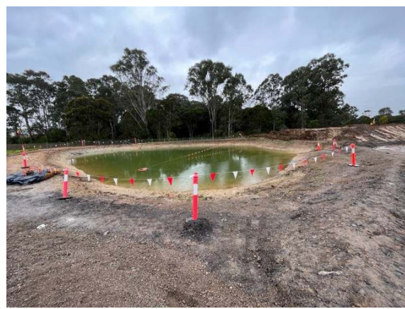
Photo 22: Northern sediment basin – Water reused for dust suppression or trucked to the St. Mary’s WTP
