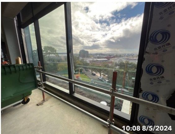
Photo 20 Level 3 Planter Box
