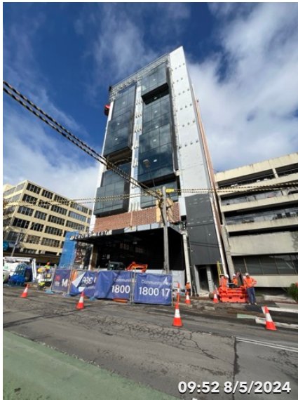
Photo 1 OSD Site C - Building Construction nearing completion. Traffic controls in place Site fence and hoarding in place
