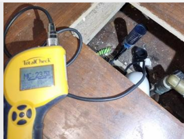
Shop 47 south floorboard of 23.5% indicate too high moisture condition
