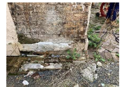
Evidence of salt attack on base course and also loss of mortar
