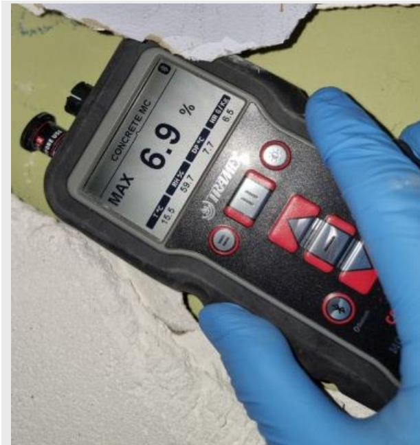
Shop 47, east wall, rendered brick wall - very high (6.9%) moisture content.
