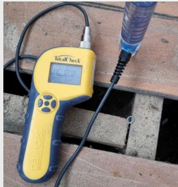
Shop 47 floorboard of 17.1% indicate high moisture condition
