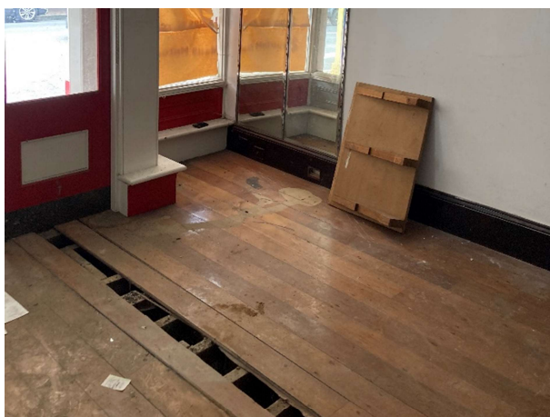
Figure 4-6: Detail view of floor in 47 George Street in 2024, showing damage associated with high moisture levels.
