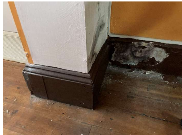
Figure 4-4: Efflorescing stone at base of walls, shop at 43 George Street.
