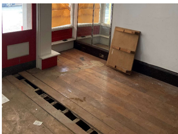
Figure 4-24: Area of damaged flooring, previously buckled owing to the effects of moisture,.
