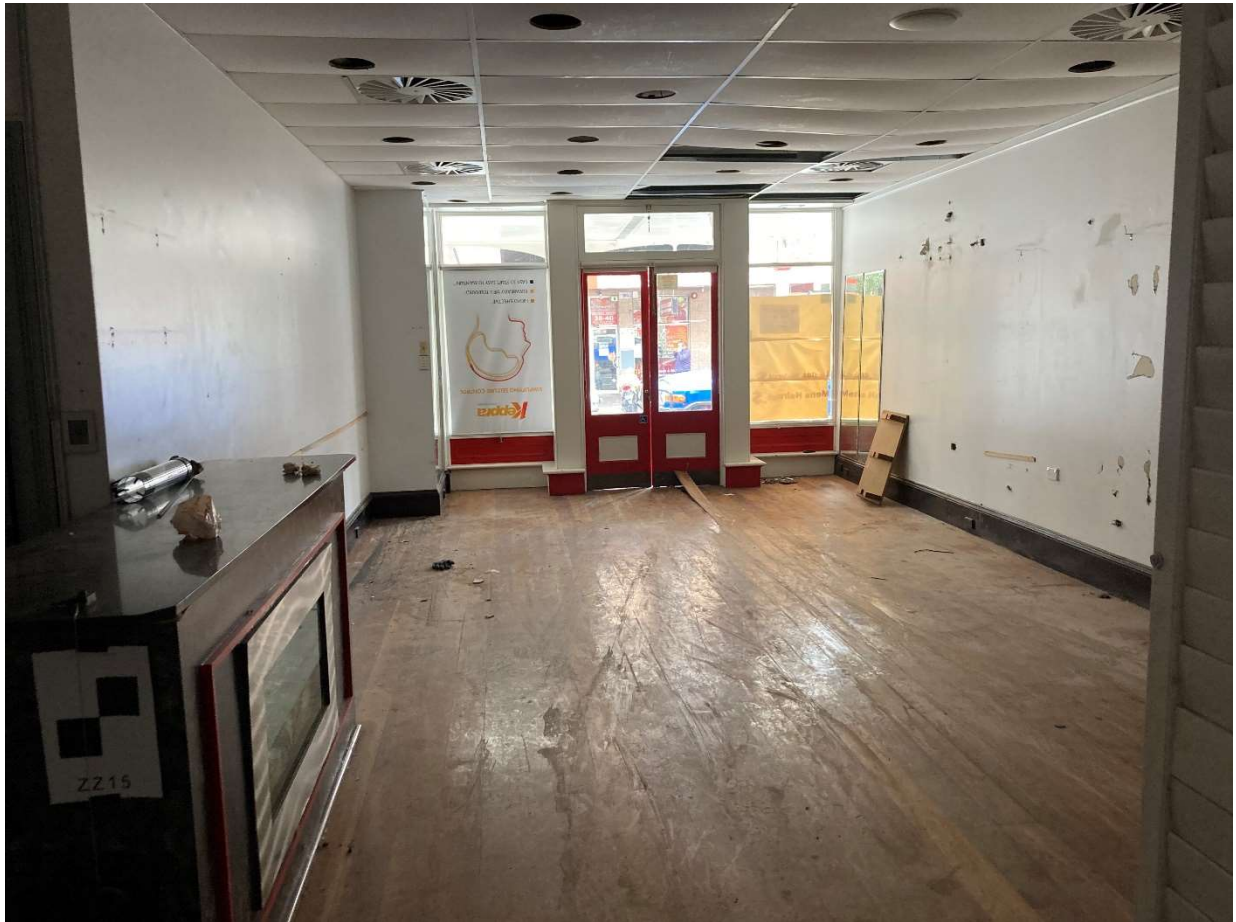
Figure 4-5: General view north in shop at 47 George Street (ground floor) in 2022. Note buckling floor, evidencing high moisture levels.
