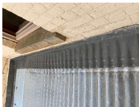
Figure 4-7: Synthetic abutment flashing recently installed on rear skillion roof.
