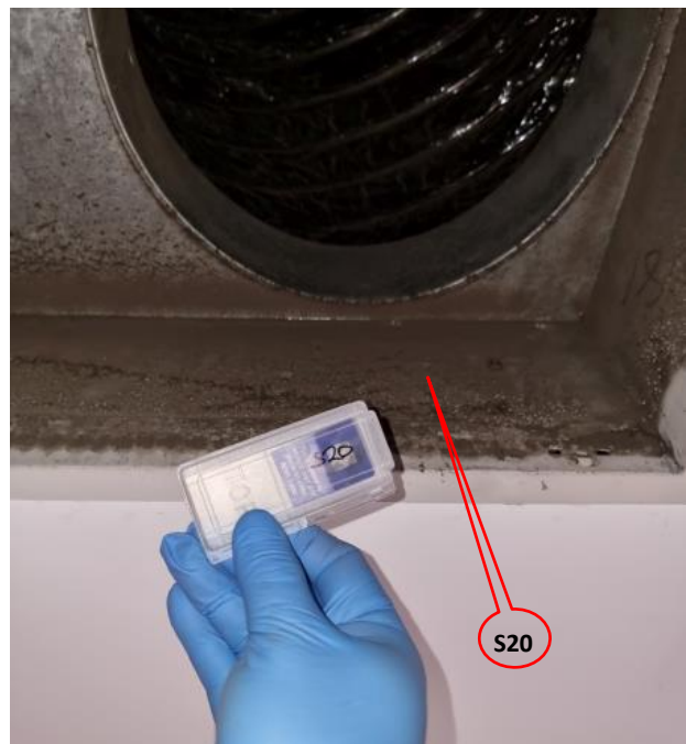
Photograph A.20: Level 1, Room 3, AC Return Air
