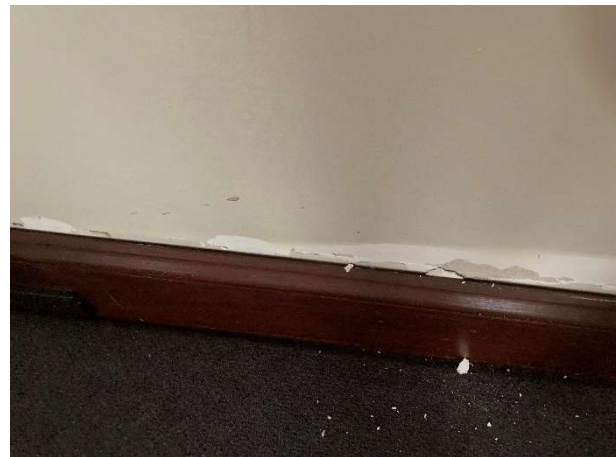
Figure 4-10: Evidence of moisture adversely affecting rendered masonry walls in 47 George Street.
