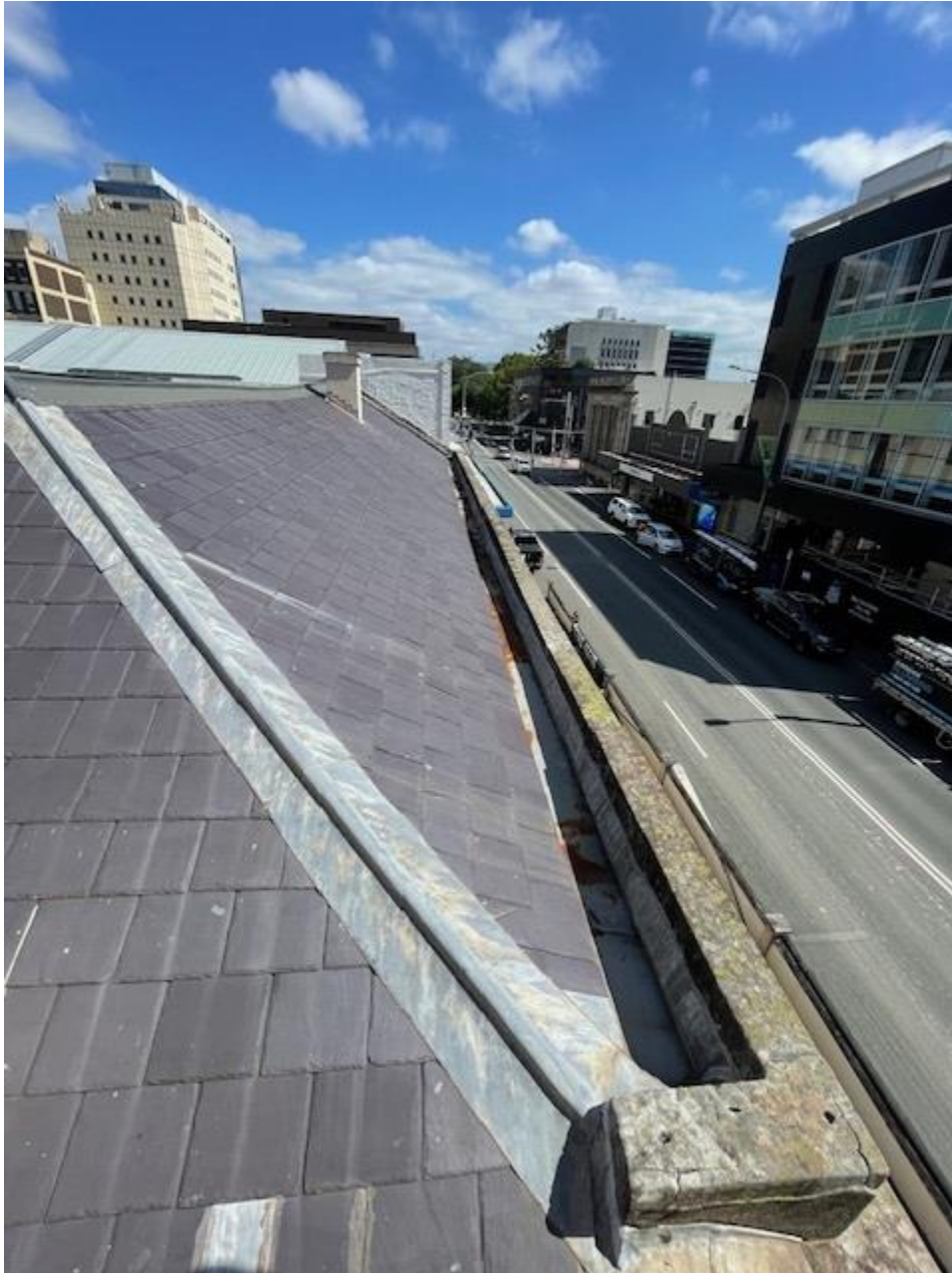
Figure 3: Front parapet internal box gutter
