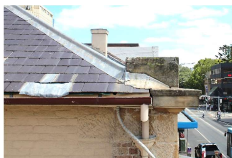
Figure 4-21: Extensive cracking through full section of north east parapet stone.
