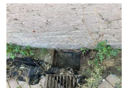
No visible DPC in external masonry walls
