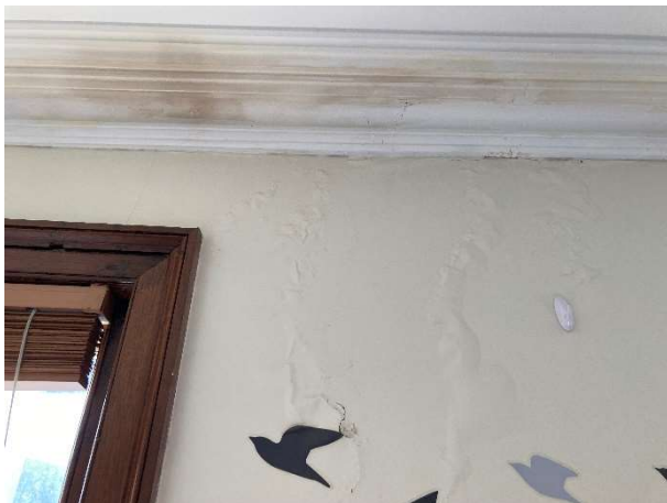
Figure 4-9: Detail view of water damage affecting north cornice and wall, 47 George Street.
