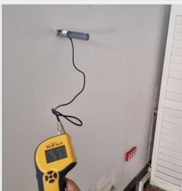
Shop 47 west wall at mid height, gypsum wall 0.9% indicate of wall too wet for painting which also have the potential for mould growth
