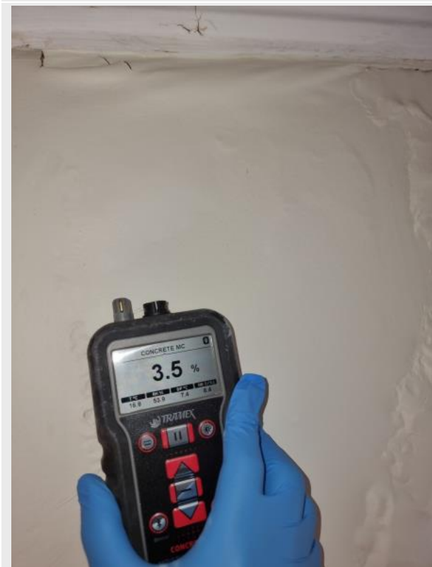
Level 1, Room 1, north wall above window - 3.5% on rendered wall, moisture level still too high.
