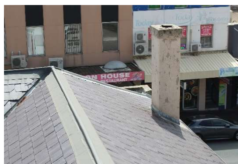
Figure 4-11: Capping of the north east chimney (Chimney 1) is damaged.
