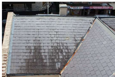
Figure 4-9: Example of galvanised steel roof valley, extensively corroded.
