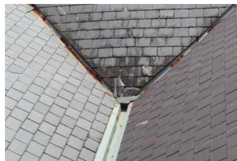
Figure 4-5: Detail view of rear face of main roof (over 45 & 47 George Street) showing slates in poor condition. Note also corroded galvanised steel valley gutters.
