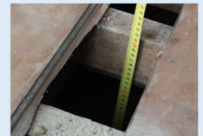
Clearance beneath joist is currently in the order of 300mm (Shop 47)
