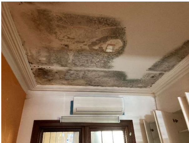
Figure 4-3: Detail view of mould affected ceiling at rear of shop at 43 George Street. Note set lines in plaster, indicating that the ceilings, and consequently cornices, are modern.
