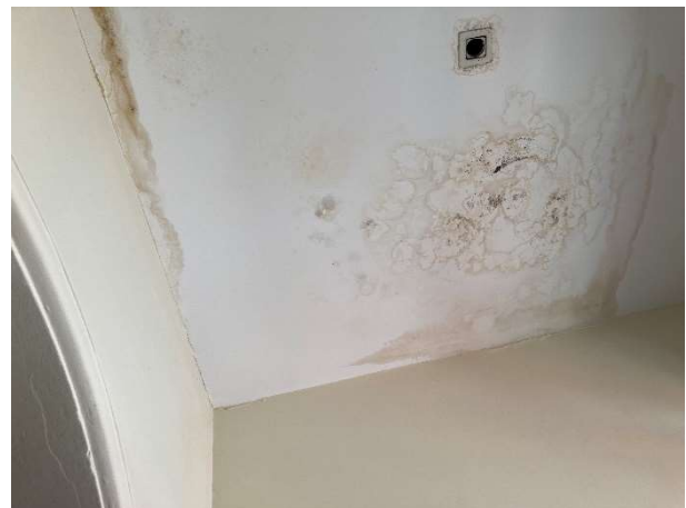
Figure 4-13: Water damage and mould affecting ceiling in first floor hallway.
