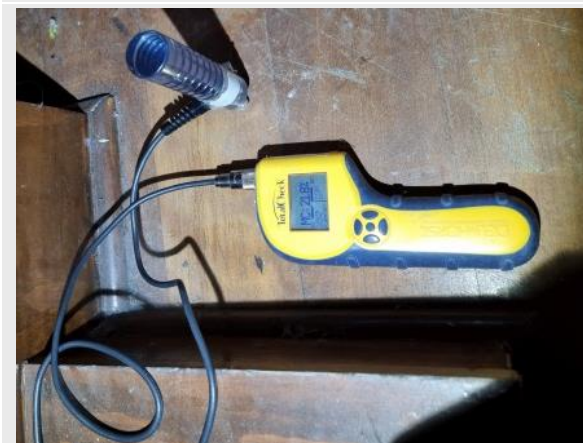
Shop 47 south floorboard of 21.8.1% indicate too high moisture condition
