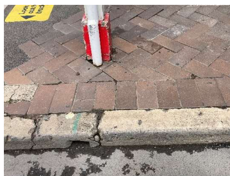
Figure 4-15: North verandah downpipe discharging to paving, also showing outlet in stone kerbing.
