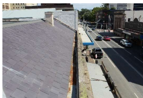
Figure 4-13: Corroded box gutter behind sandstone parapet of the north elevation.
