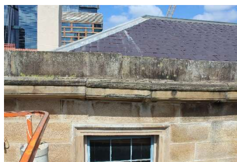
Figure 4-20: Open joints of parapet stones.
