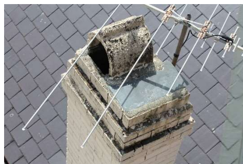
Figure 4-10: Extant cowl of south west chimney (Chimney 3). The adjacent cowl is missing.
