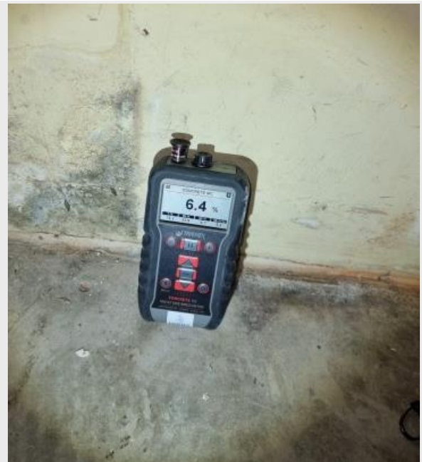
Shop 47, storeroom under stair, low west wall - very high (6.4%) moisture content.
