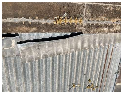
Figure 4-6: Dislocated abutment flashing at junction of sandstone north wall and verandah roof.
