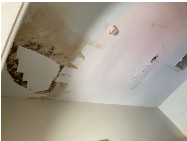
Figure 4-12: Water damage and mould affecting ceiling in first floor hallway.
