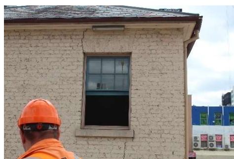
Figure 4-22: Cracking brickwork around rear first floor window of 47 George Street.
