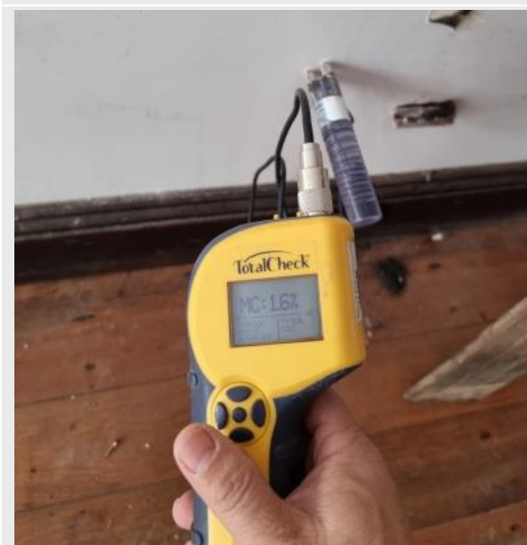
Shop 47 west wall at low height, gypsum wall 1.6% indicate of wall too wet for painting which also have the potential for mould growth
