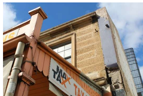
Figure 4-23: Western end of the timber verandah structure, showing evidence of rotting timber and peeling paint.
