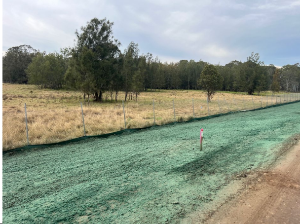
Defence - Hydromulch has been applied to the batters at the northern end of the Defence site.
