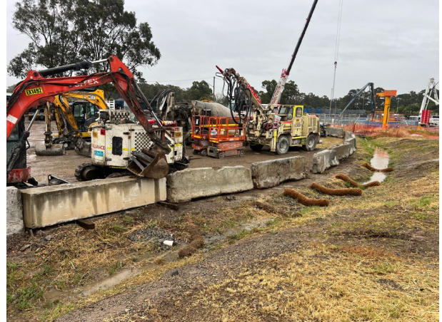
Claremont Meadows – The removal of the concrete washout adjacent to this drain has reduced the runoff risk.
