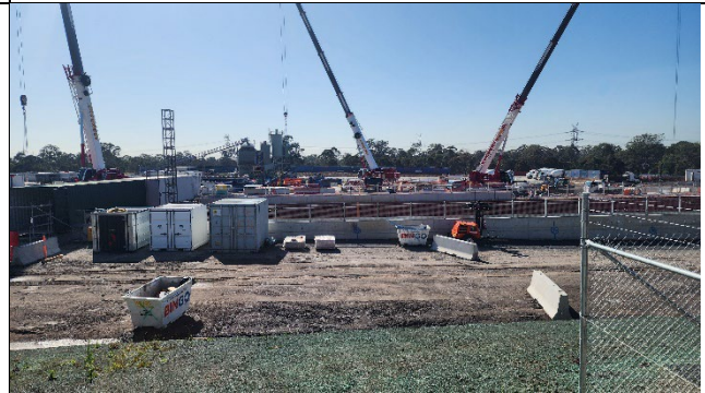
ORH – box and batch plant.
