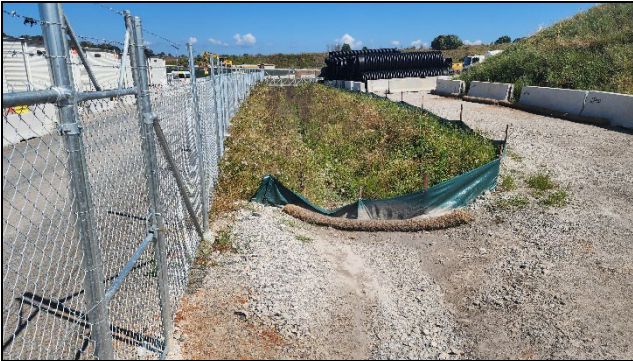
SMF – Weeds in swales and topsoil stockpile. Spraying was pending agreement of suitable herbicide.
