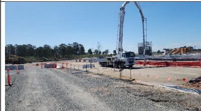
BFD – Concrete pumping on the northern side of the box had commenced.
