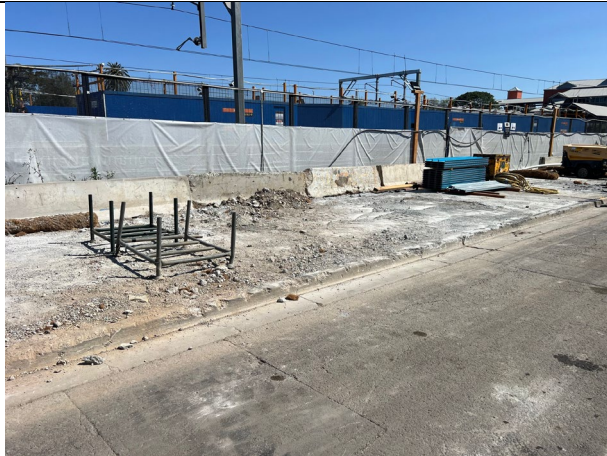
Compound - Waste concrete stockpiled in this location in the compound was sent off site for recycling.
