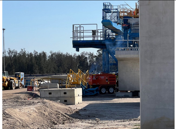
Luddenham North – Excessive smoke was seen from this diesel generator. ER was informed that this is part of the servicing process due to the particulate burn-off.
