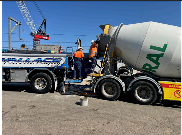
Compound – The concrete pump had a plastic catch tray underneath it, however the ER questioned its volume and recommended a tray with more capacity.
