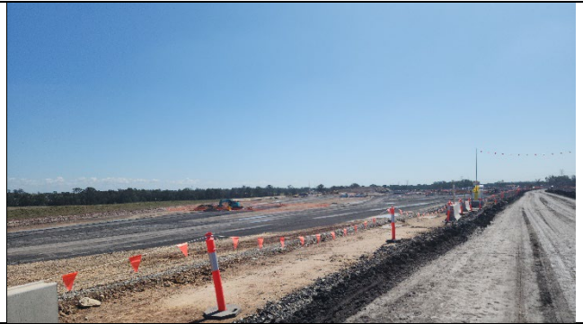
SMF – View of SMF facing north.
