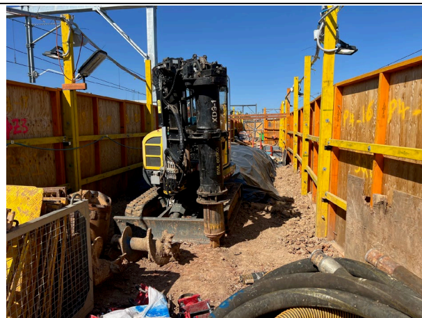
Platform 3/4 – Works were suspended prior to WE12 with all stockpiled material covered in plastic to reduce the ERSED risk.
