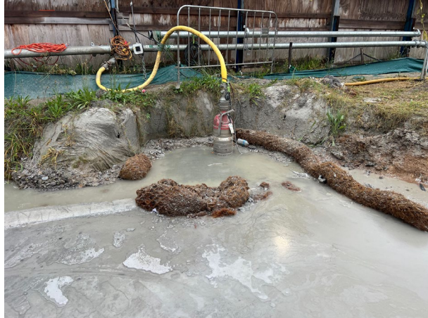
Claremont Meadows – All water in the NW corner is pumped from the sump to the WTP. Additional pumps are available in case of a breakdown.
