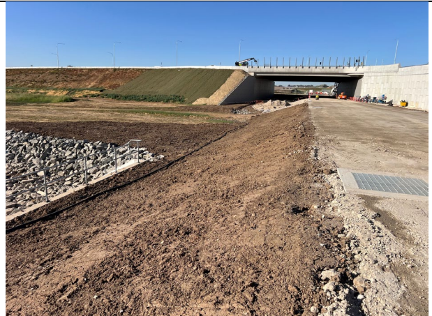
M12 Bridge - Batters have been topsoiled and are due to be hydromulched in late September / early October.
