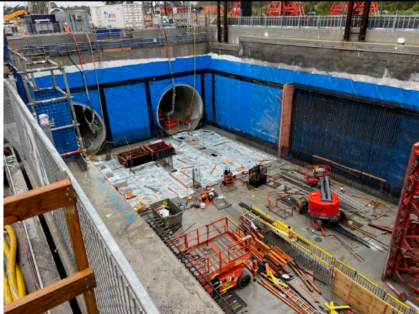
Orchard Hills – Works progress in the dive structure with low environmental risk.
