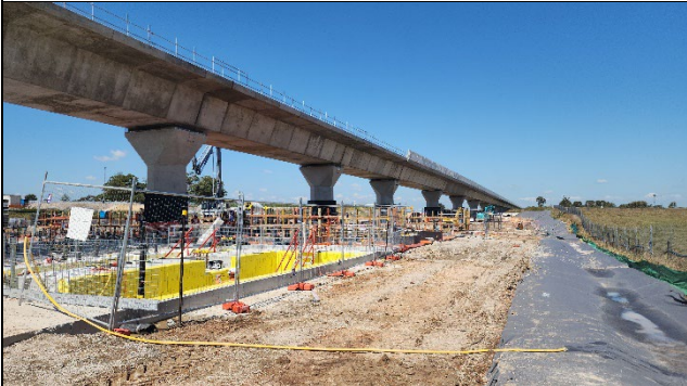
LUD – reshaping of the boundary swale had occurred, FRP and concrete pours had commenced. Lift shaft waterproofing works commenced.
