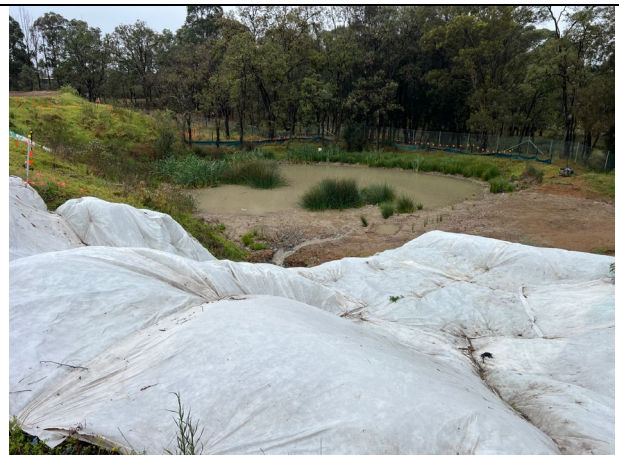
Orchard Hills – The sediment basin has significant freeboard despite 12.8mm of rain received prior to the inspection.
