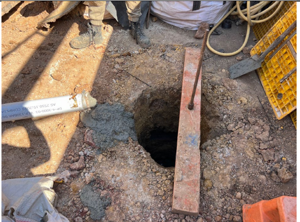
Platform 3/4 - Concrete was poured into piles, all concrete washout occurred in the compound and not on the platform.
