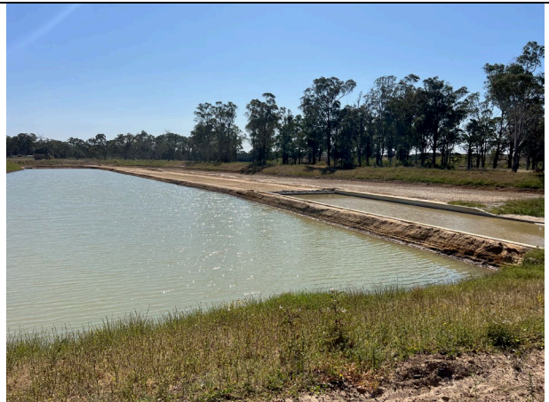
14ML Basin - The basin is still being used by SCAW as a water source for construction activities.
