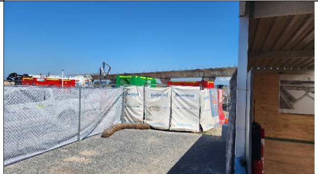
LUD - Hybrid generator installation (good practice).
