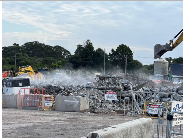
Claremont Meadows – Water cannons were in operation to control the dust during concrete breakup.
