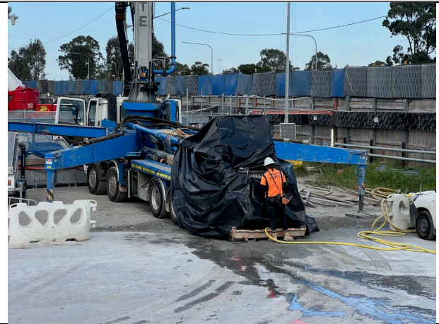
Claremont Meadows – Black plastic was placed around the concrete pump to capture any concrete splatter during pours.
