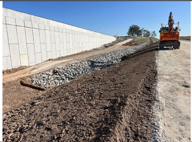
M12 Bridge – The rock lined channel adjacent to the M12 access track is being constructed.
