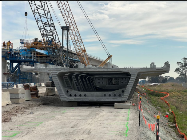
Luddenham North - Segments are stored in dedicated segment storage areas adjacent to the main alignment.
