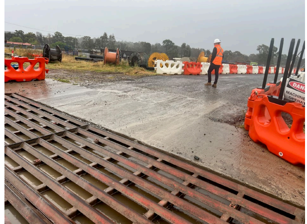
Claremont Meadows – The rumble grid at the site exit was working effectively.
