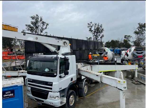
Bringelly – The noise wall has been installed prior to OOHW concrete pours.
