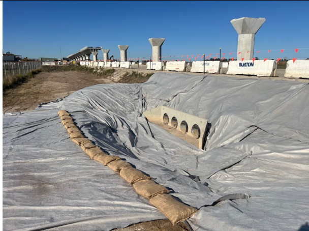
Luddenham North - A good drainage control has been installed on the access road cross drain.
