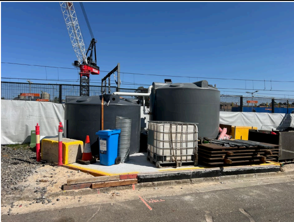
Compound - The water tanks to allow water recycling are setup, however do not have any water stored in them as of the last ER inspection on 23/09/24.
