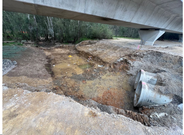
Defence - The headwall was about to be installed and the finalisation of the channel at Unnamed Creek.
