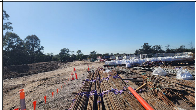
ORH – Batch plant generators and FRP prep area.
