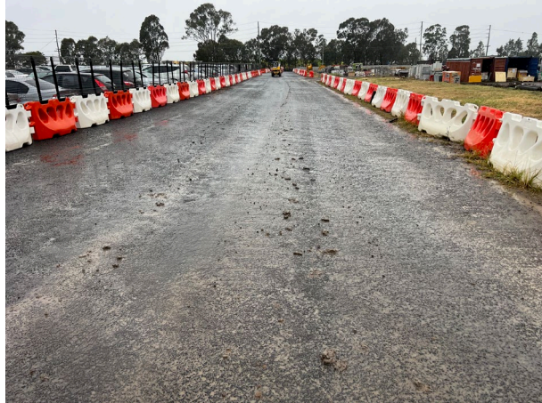
Claremont Meadows – Mud was noted on the internal sealed road, however the streetsweeper was present to continually remove this.
