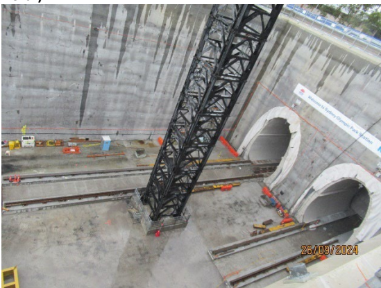
Figure 1.7 Tower crane in place and site being prepared for TBM arrival (SOP).
