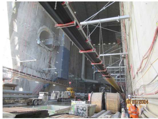
Figure 1.4 View of station box looking west with pedestrian adit evident (Burwood North).
