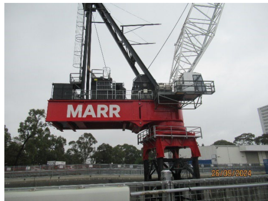
Figure 1.8 Tower crane installed with noise mitigation measures at SOP for removal of the TBM.
