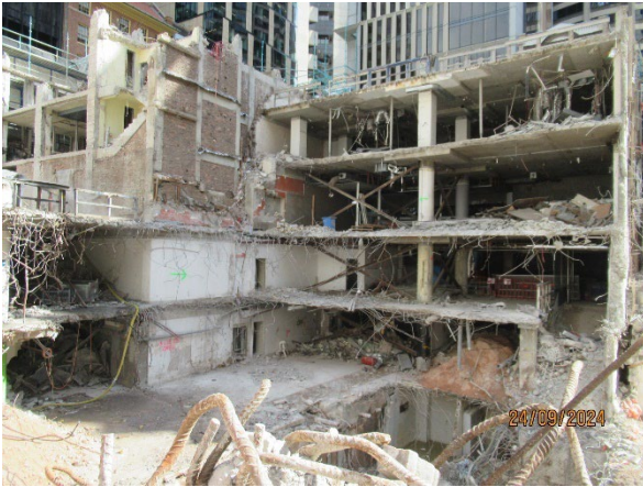
Figure 3.6 Hunter St West: Demolition of buildings ceased while supports designed for Skinner’s Hotel.
