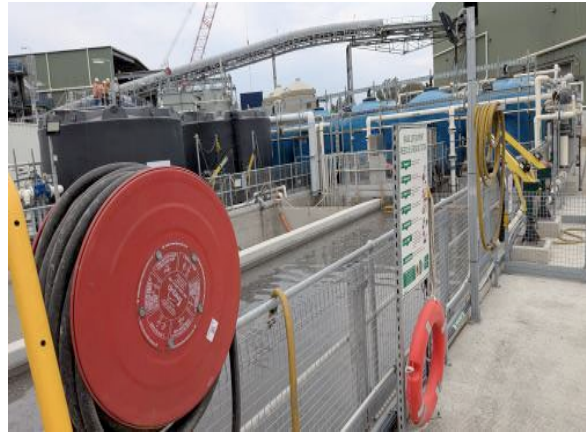
Figure 2.16: Rosehill site: Water Treatment Plant is operating with centrifuge installed and commissioned.
