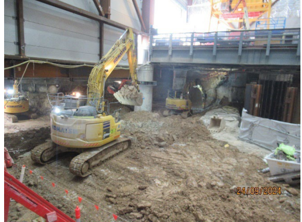
Figure 3.2 Pyrmont East: Excavation of the permanent shaft using multiple excavators with rock hammers.
