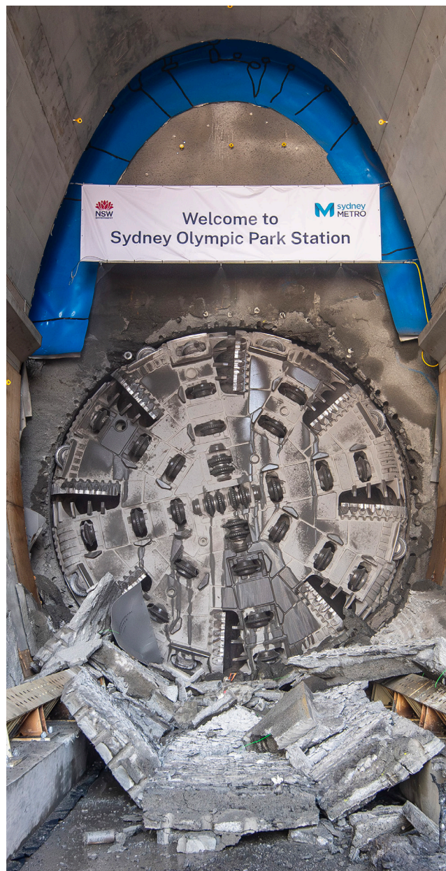
TBM Dorothy completes the first phase of tunnelling at Sydney Olympic Park.
