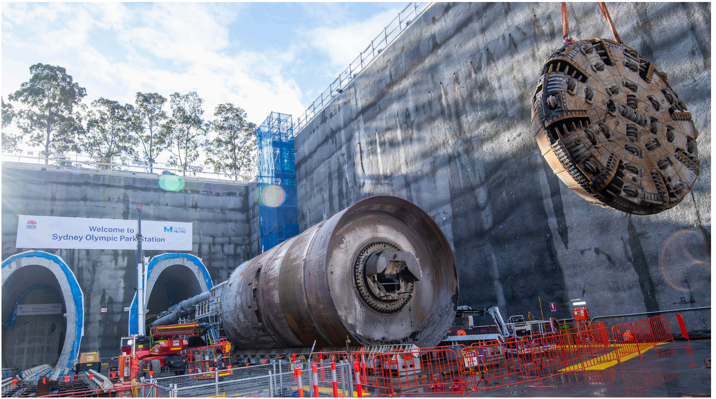
A different kind of face lift! TBM Betty's cutterhead has successfully been retrieved from Sydney Olympic Park metro station site.
