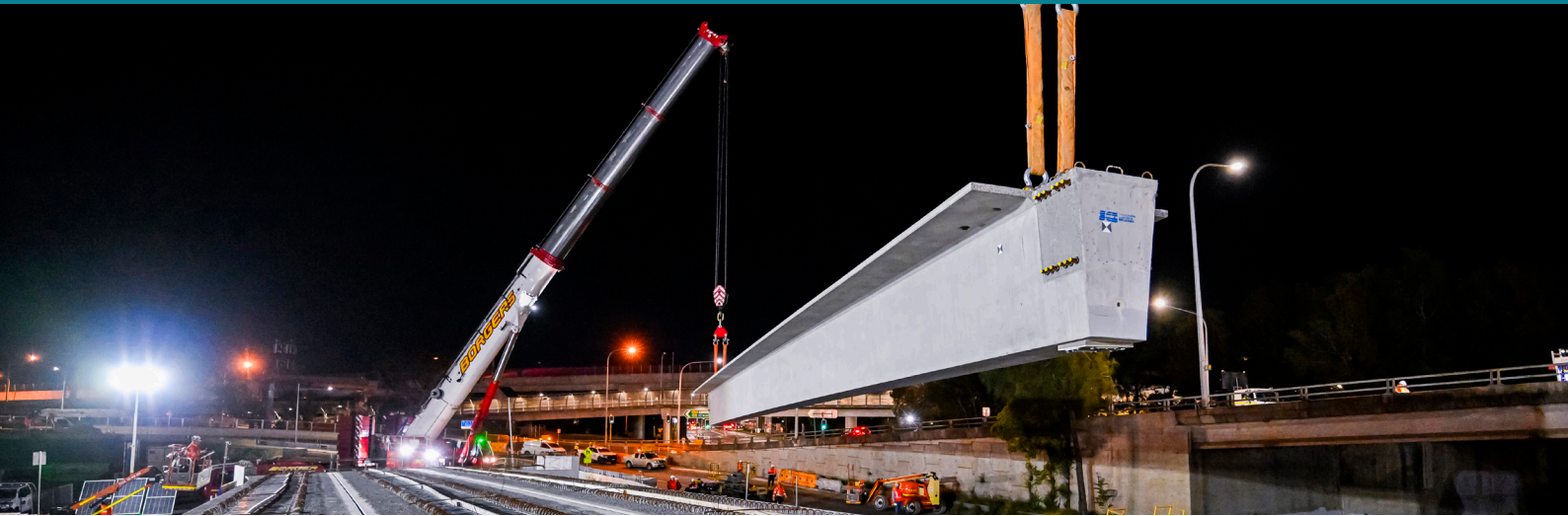
Dual crane lift positioning the girders into place for the A'Beckett's Creek bridge.
