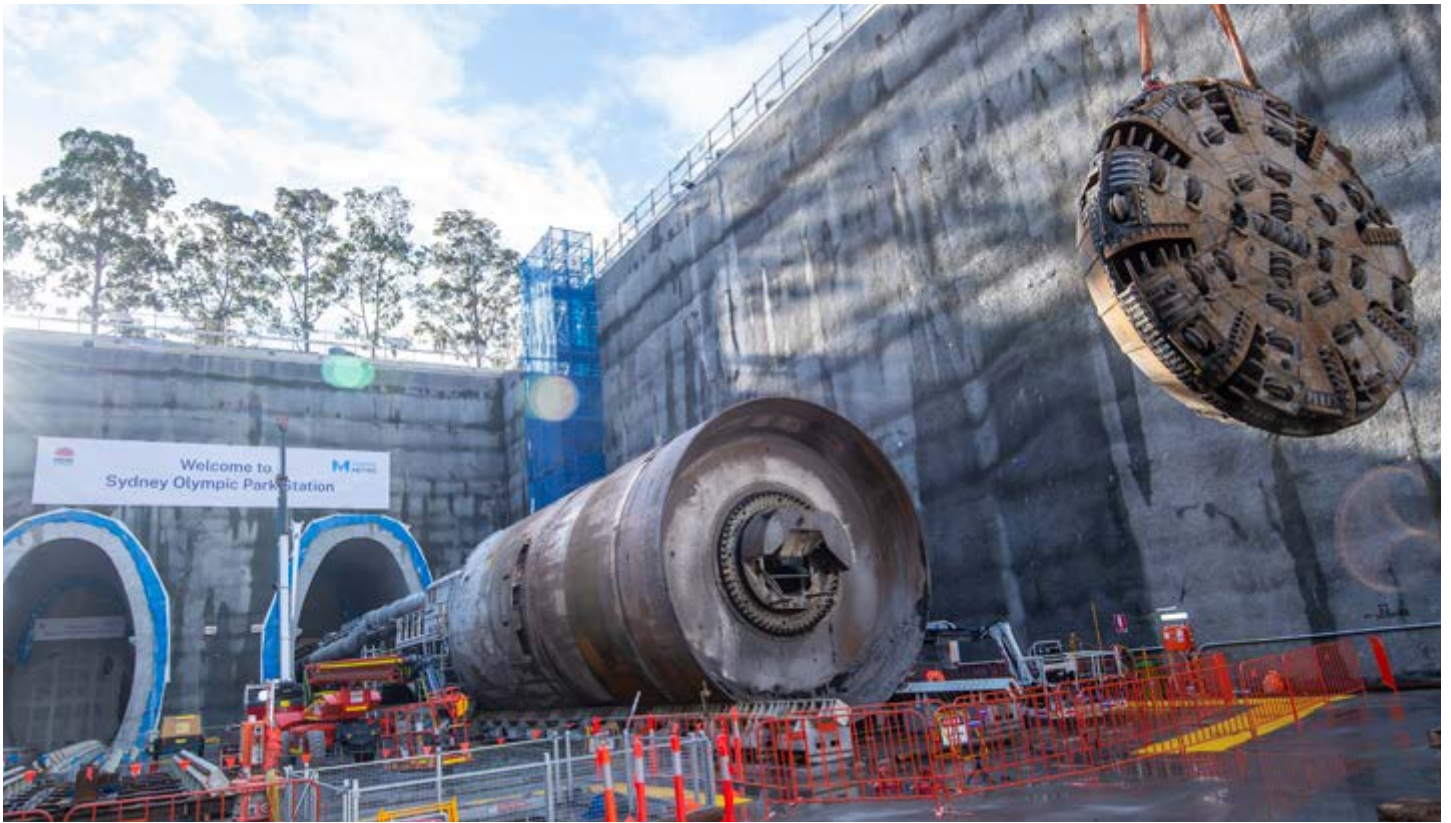
A different kind of face lift! TBM Betty's cutterhead has successfully been retrieved from Sydney Olympic Park metro station site.
