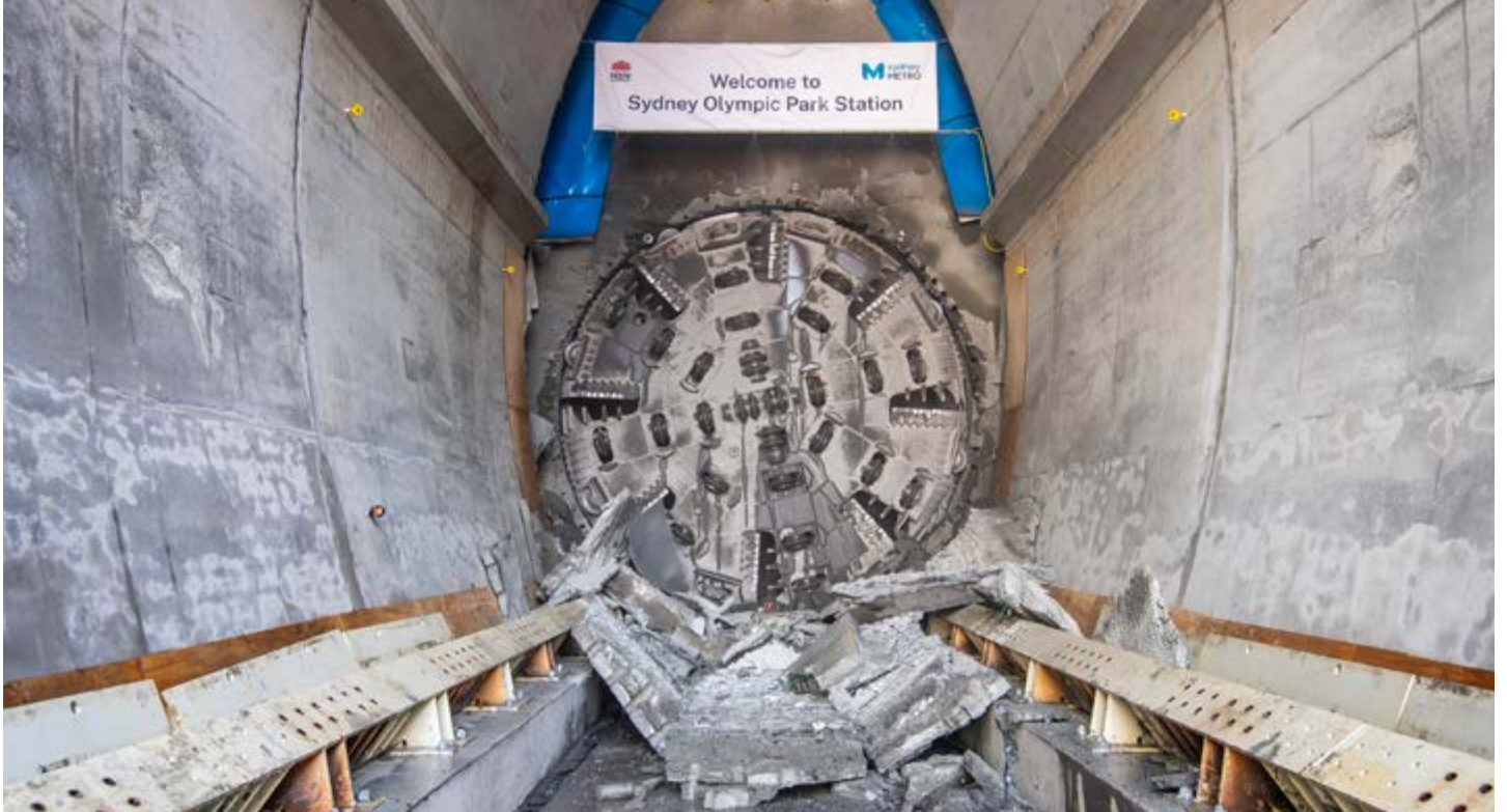
TBM Dorothy completes the first phase of tunnelling at Sydney Olympic Park.
