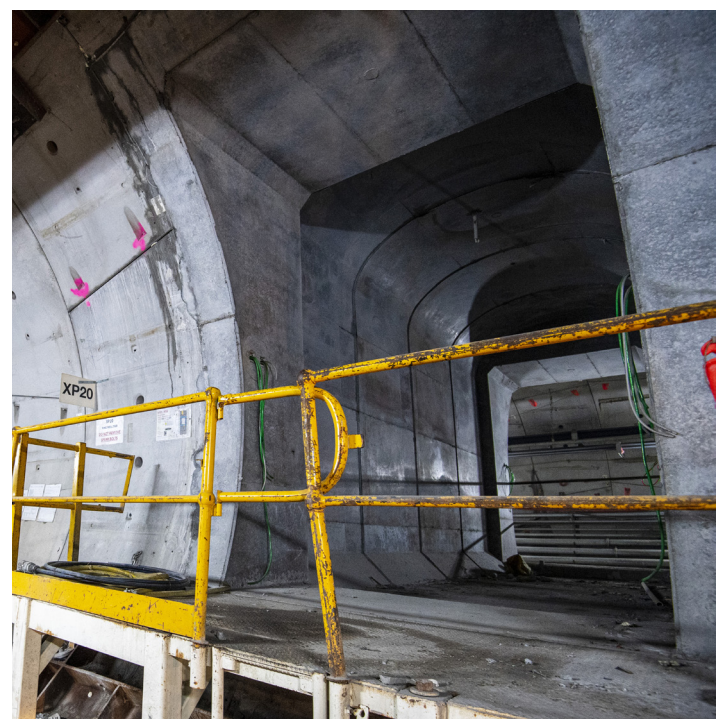
A completed cross passage on the Sydney Metro City and Southwest line.
