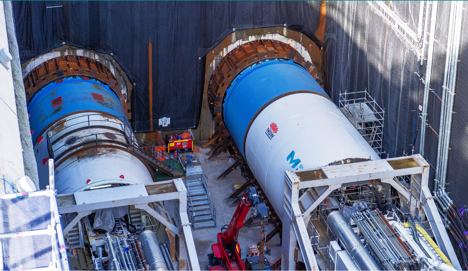
Two tunnel boring machines prepare for the start of their 2.3 kilometre journey from The Bays to Hunter Street.
