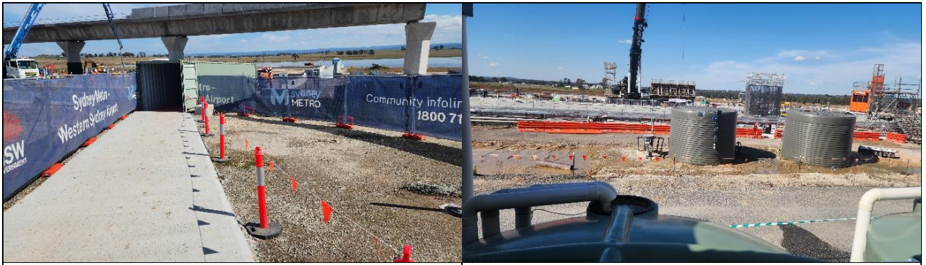
LUD – shipping container bridge installed and reduction of swale commenced AEC - box and laydown areas
