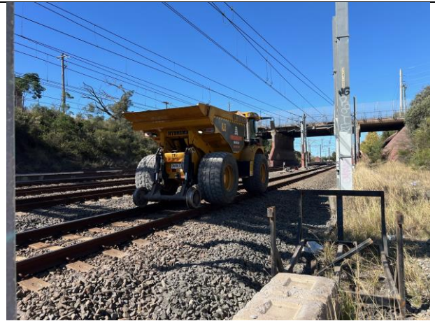
Hobart St Laydown - Moxy hydrexes were used to transfer spoil from platform 1/2 to the laydown areas at Hobart St
