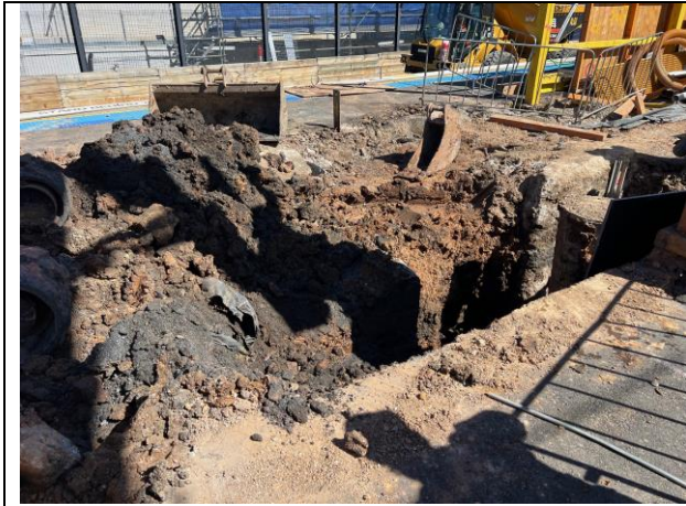
Platform 1/2 - An original brick footing was unearthed, the archaeologist was on site to assess the structure
