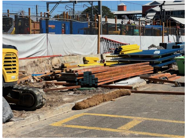
Compound - Previously stored spoil has been removed to allow material storage for WE09
