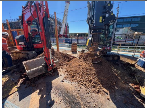
Platform 3/4 - Piling spoil was regularly removed, with no evidence of spillage beyond the platform
