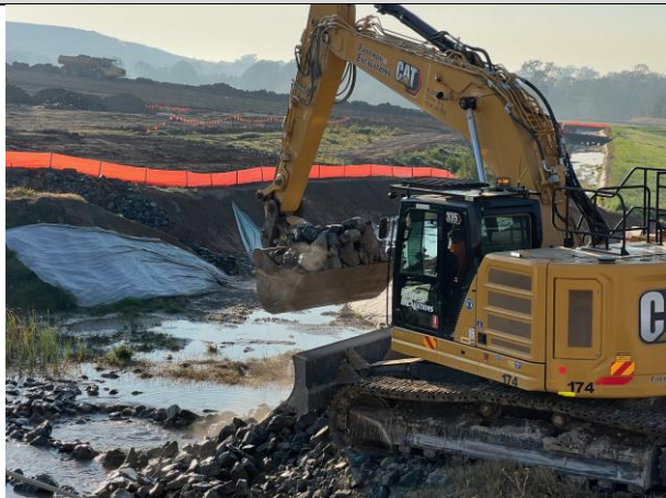
M12 Bridge - Rock in both the onsite and off-site drains was being removed and cleaned
