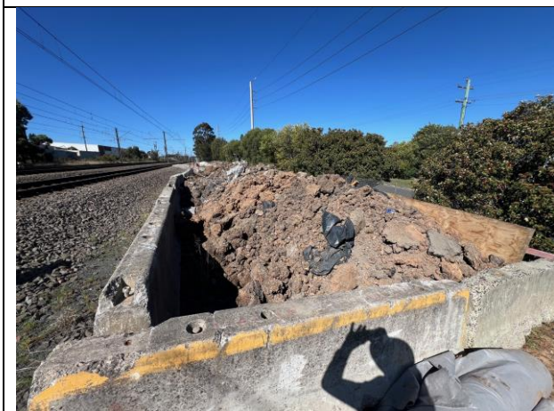
Hobart St Laydown - Spoil from platform 1/2 was loaded to specific areas bounded by jersey barriers with ERSED controls
