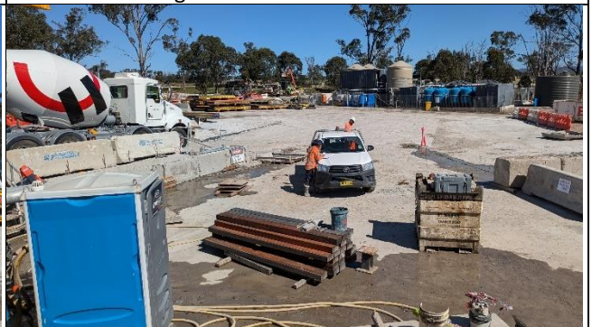
Bringelly view west from shaft – Concrete slab placed over loading/unloading and delivery areas.
