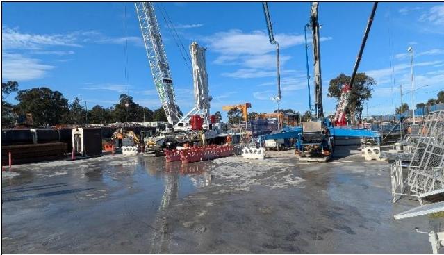
Claremont Meadows view north of shaft – Concrete delivery and washout well managed.
