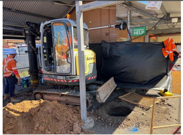
Platform 1/2 - Barriers were present to prevent works inadvertently impacting on the platform building
