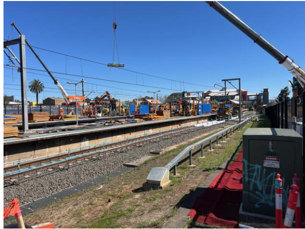
Compound - Cranes were setup in the compound to lift materials to and from platform 3/4
