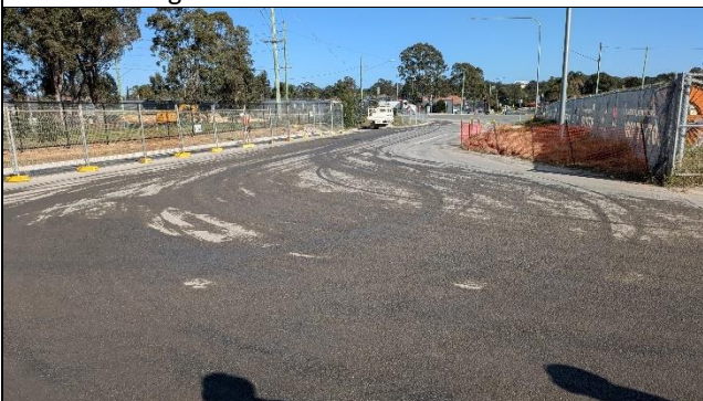
Claremont Meadows – Negligible tracking noted on Gipps Rd. at southern site access.
