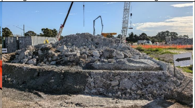
Claremont Meadows concrete washout area north of Shaft – Needs Improved design and management.
