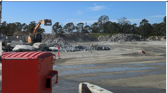
Orchard Hills view west – Former tunnel segment storage area used to store materials for haulage offsite.
