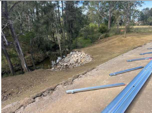
Blaxland's Creek - Final area of Blaxland's Crk bank has stabilised/hydromulched. Guard rails are being installed
