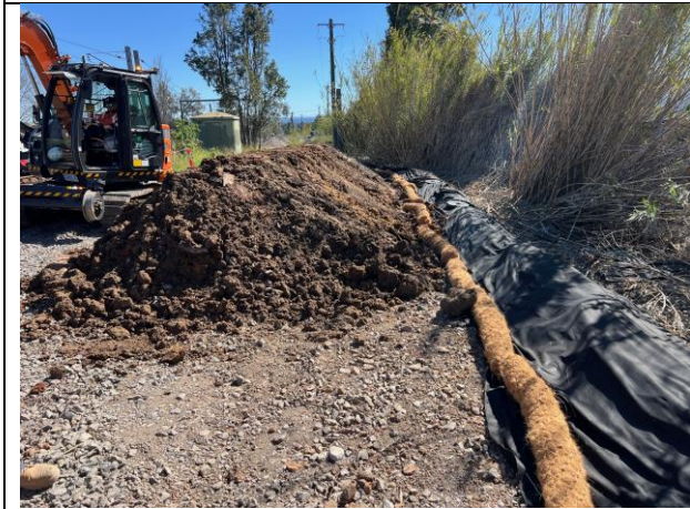
Stockpile area 1 - ERSED controls were of a good condition to control impacts from stockpiled material
