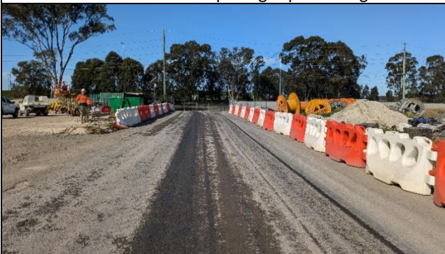
Claremont Meadows south, view to HV exit – Internal haul road in good condition.
