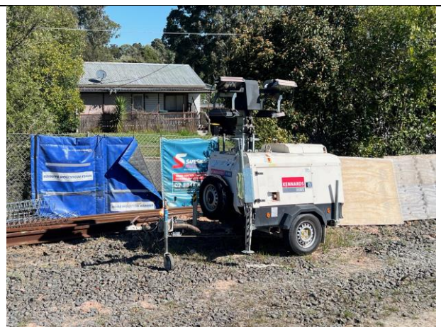
Hobart St Laydown - Hybrid lighting towers were utilised along Hobart St to minimise noise impacts
