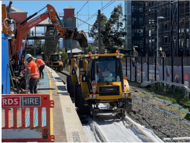
Platform 3/4 – Spoil was loaded out on the hydremas and taken to spoil location 1
