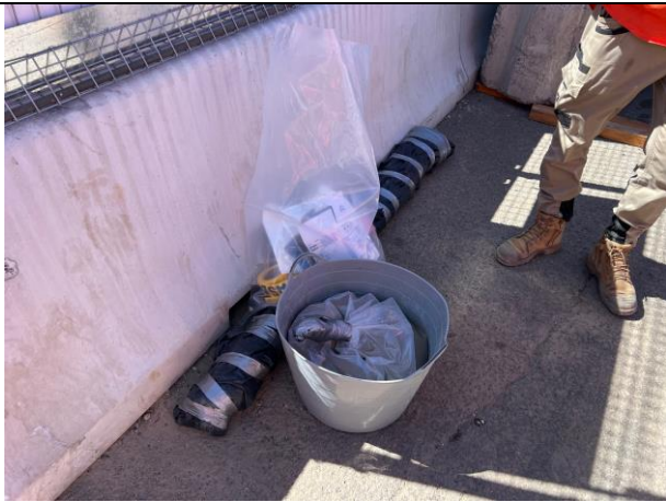
Compound - Asbestos pipe located on platform 3/4 was wrapped and clearance certificate has been given.
