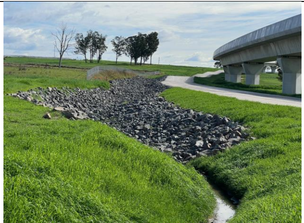
Cosgrove's Creek - Drainage channels north of Creek complete. Exposed areas revegetated in caretaker mode
