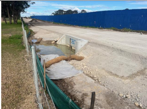
Lansdowne Road - The haul road is nearing completion, controls are of a good quality and appear to be effective
