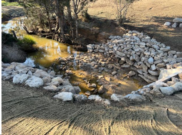
Blaxland's Creek - The downstream channel has been rehabilitated, with rubbish removed and areas stabilised
