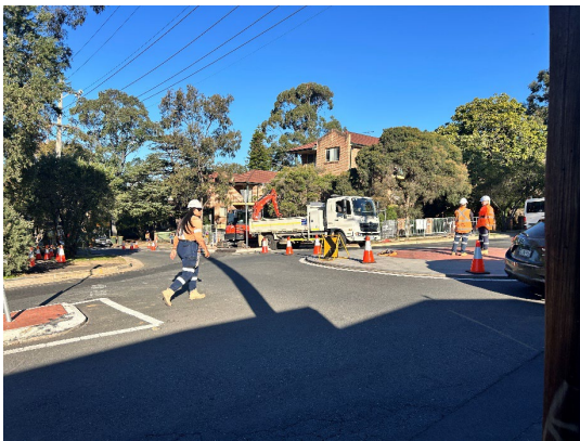
Figure 4.1: Westmead Utility Works – Telstra Pit backfill and footpath reinstatement Cnr Hassell and Bailey Streets
