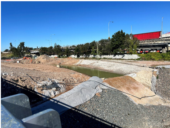
Figure 2.11: Clyde MSF Site – Cofferdam with minor erosion
