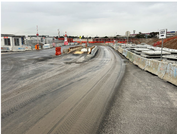
Figure 2.11: Clyde MSF Site – Internal Haul Roads with sediment
