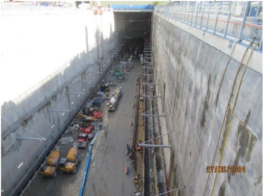
Figure 1 5 TBM support in the station box. Management of cross passage spoil (Burwood North).
