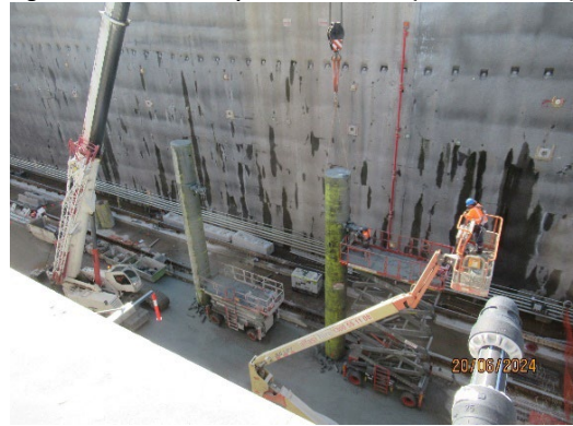
Figure 1 6 Removal of concrete pillar and steel decks completed during the reporting period (North Strathfield).
