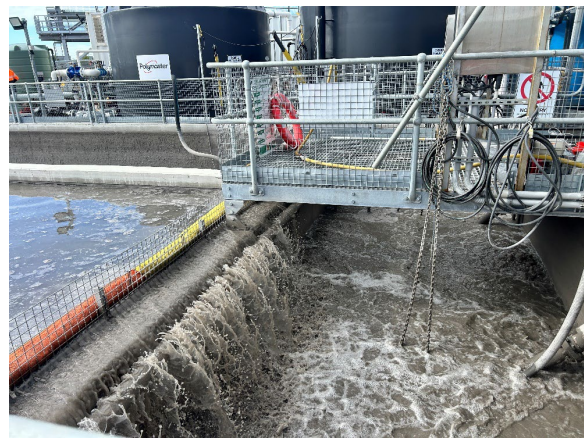
Figure 2.10: Rosehill Site – WTP operation
