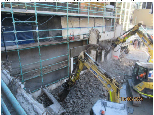
Figure 3.6 Hunter Street West: Demolition of buildings ongoing. Investigations to reduce impacts on Skinners Hotel ongoing.
