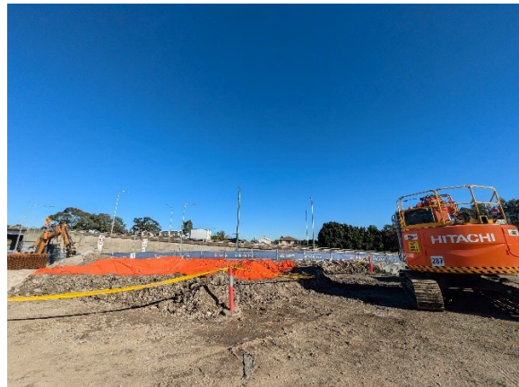
Figure 2.4: Clyde Site: Area set-up with geofabric lining for waste from HV Protection Slab investigation works.
