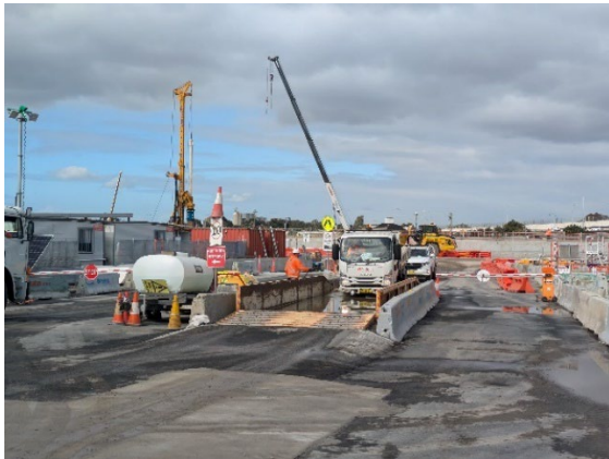
Figure 2.13: Clyde MSF West Site: Wheel wash and water cart with operator observed to manage tracking.
