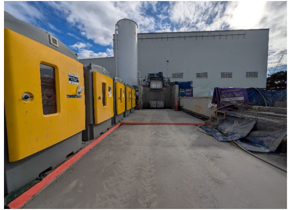
Figure 2.6: Westmead Site: Appropriate Chemical Storage -WTP.
