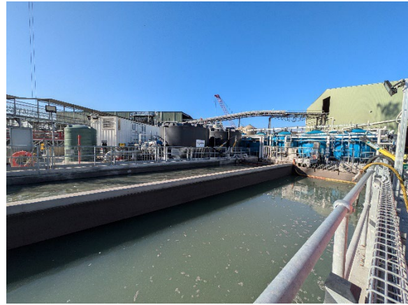
Figure 2.8: Rosehill Site: WTP operation.
