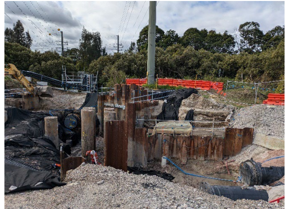
Figure 2.12: Clyde MSF East: North anchor block tie-in works; GLC Report Sydney Water Main works on hold.
