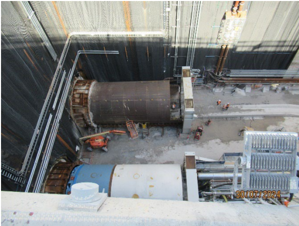
Figure 3.7 The Bays: Ongoing tunnelling of TBM Jessie. Temporary cessation of tunnelling to transition TBM support infrastructure.
