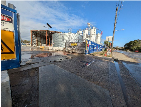
Figure 2.7: Rosehill Site: RH Gate 2 – evidence of sweeper mobilised and site egress maintained (no tracking).
