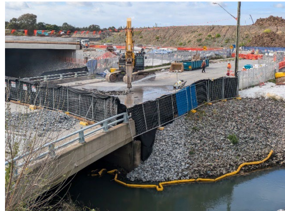
Figure 2.14: Clyde: Kay Street Bridge Demolition - controls noted (e.g. water mister, geofabric installed along ATF).
