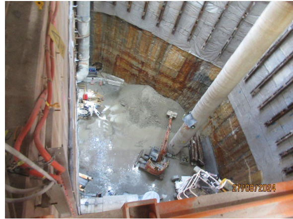
Figure 3.2 Pyrmont East: Tunnelling by two road headers with roof support and ventilation activities ongoing.
