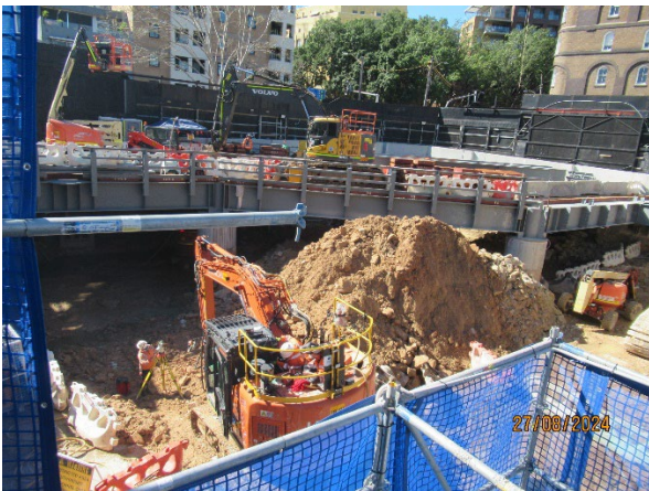
Figure 3.3 Pyrmont West: Ongoing construction of the steel deck. Removal of spoil. Excavation by rock hammer.
