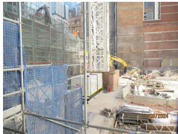
Figure 3.6 Hunter Street West: Building at 9 Hunter Street at or below ground level.
