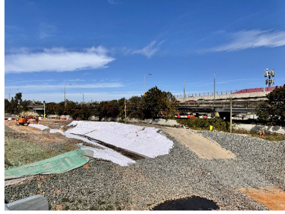
Figure 2.12: Clyde MSF West – Area 1 Swale Drain improvement and culvert installation works ongoing.
