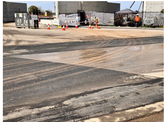
Figure 2.16: Clyde MSF West Site Gate 9: Mud tracking observed and raised as an action – refer ER Inspection section.
