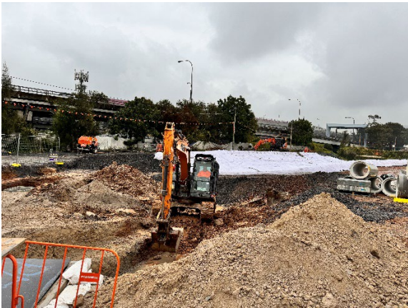
Figure 2.11 - Clyde MSF West – Area 1 Swale Drain improvement and culvert installation works ongoing.
