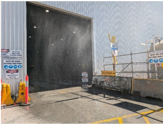
Figure 2.5 -Westmead Site: Acoustic Shed - Mister observed to operational.
