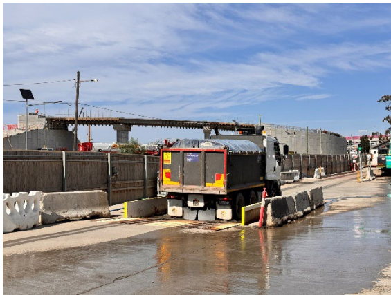
Figure 2.15: Clyde Dive: Wheel wash in use with no mud tracking observed on hardstand area leading up to exit.
