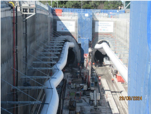
Figure 1.7 TBMs completed their traverse of the Station Box and were tunnelling towards SOP (North Strathfield).
