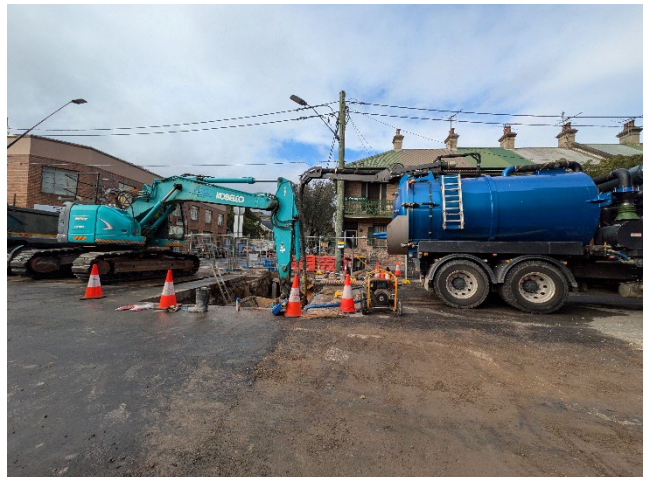
Wellington Street: Stormwater culvert works. Refer action raised under ER Inspection Section.
