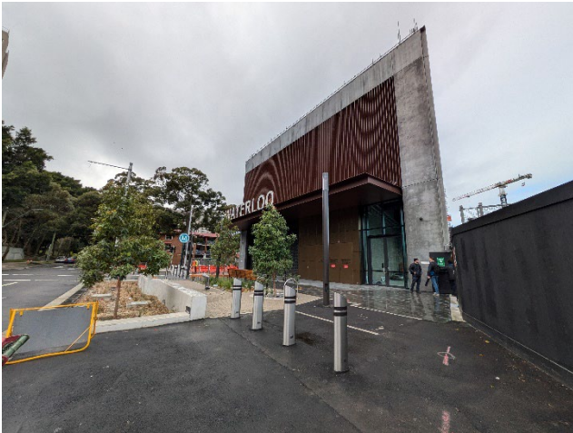
Northern Building and Station Entrance – Raglan St: Bollards, paving and raingarden installed.
