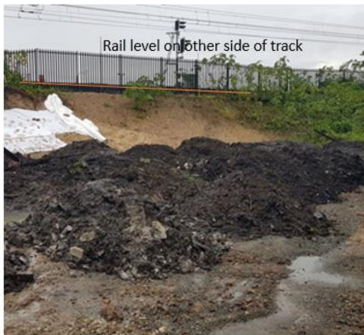
Figure 6: Image of rail line showing introduced fill to build up area of track.
