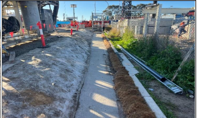
St Marys south side of Station St view east– Erosion and sediment control measures in good condition.
