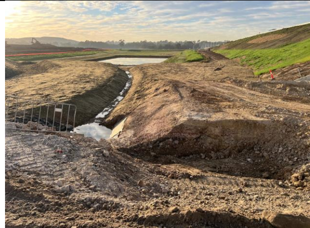
M 12 Bridge - The catchment leading to the basin has been sprayed with hydromulch
