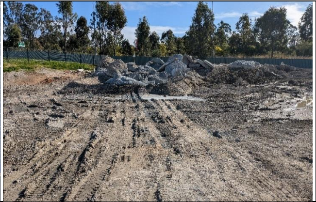
Orchard Hills Northern boundary– Concrete washout management improvements required.
