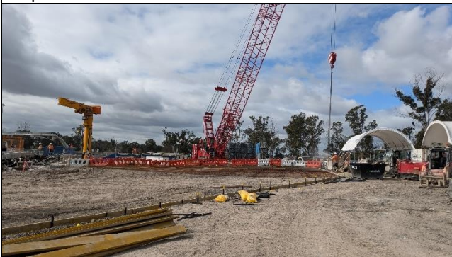
Bringelly view east to shaft– FRP underway for concrete slab over loading/unloading area.
