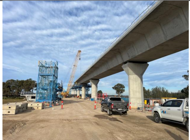
Defence - The viaduct is being constructed from the Defence site, over the Warragamba pipelines, towards Luddenham north
