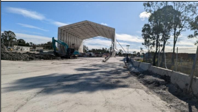
Orchard Hills south view north – Spoil management infrastructure demolition and shed removal.
