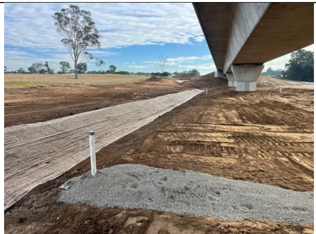
Blaxland's Creek – The catchment has been topsoiled and was due to be hydromulched the day following the ER inspection
