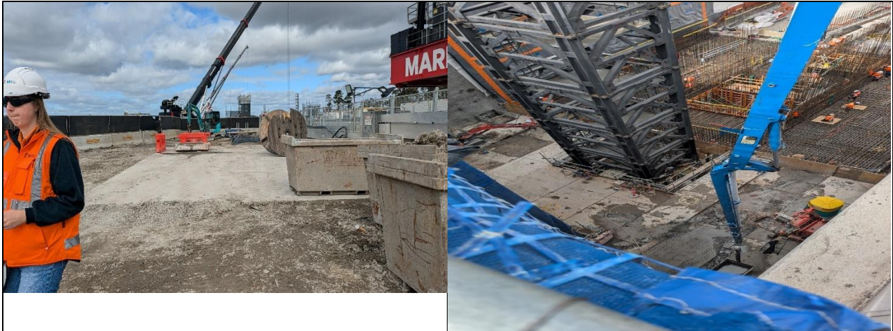
Aerotropolis view south of east side of station box– Demobilisation awaiting crane slab removal. Aerotropolis Station Box north– TBM retrieval finished with concrete delivery to portal. SSTOM FRP right
