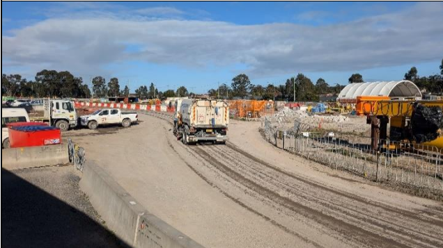
Claremont Meadows south, view to HV exit – Internal haul road in good condition.
