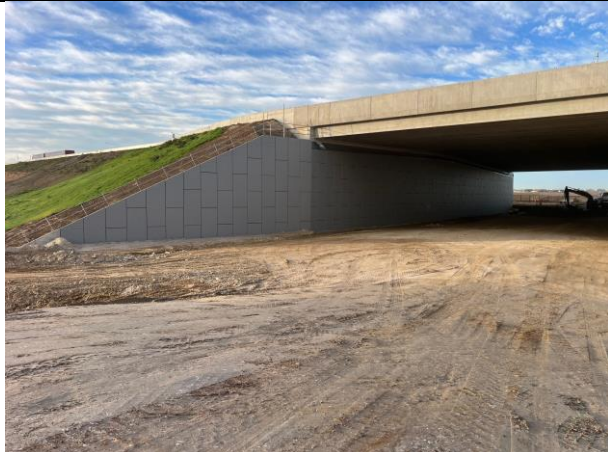
M12 Bridge - All water captured under the M12 bridge drains to the sediment basin adjacent to the bridge
