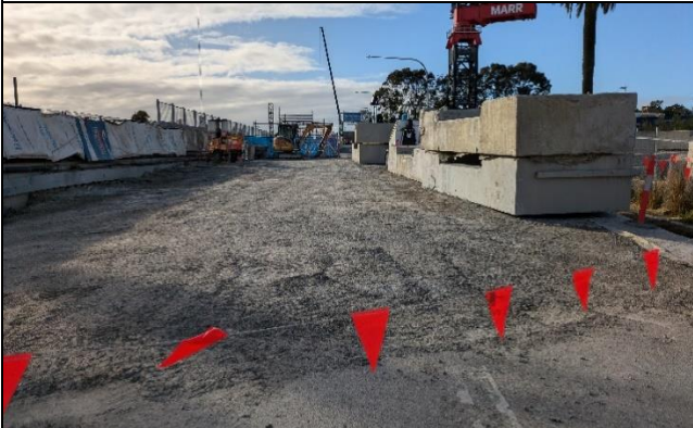
St Marys Station St view east – TBM precast support blocks ready for transport offsite.
