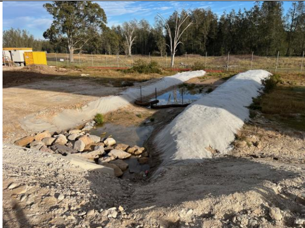
Defence - The downstream cross drainage structure is in generally good condition, however the coir logs required adjustment
