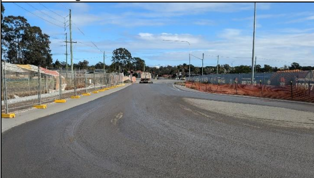
Claremont Meadows – Some tracking noted on Gipps Rd. at southern site access.
