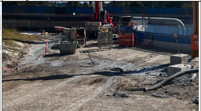
Claremont Meadows view south to shaft – Concrete washout management improvements required.
