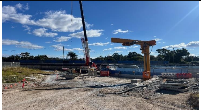
Claremont Meadows view northwest – Drop pipe at ramp abandoned, replaced by concrete pumps.
