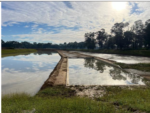
SMF - The 12ML basin is in good condition, both SCAW and SSTOM intend to discharge water at the licenced discharge point
