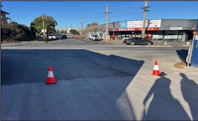
St Marys view south from Gidley St at Philip St – Negligible tracking observed from Gidley St access.
