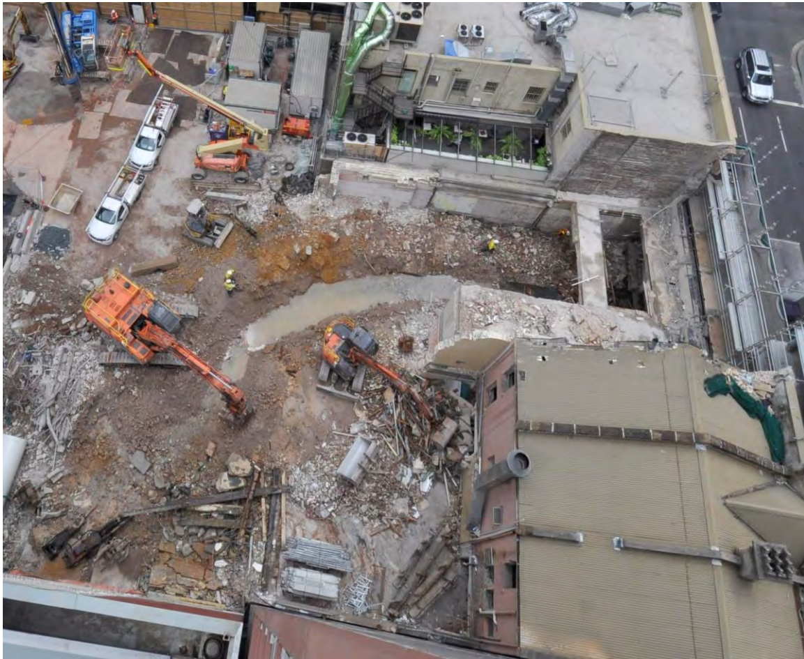
Figure 4.3 Aerial view of PS3 and PS4 on Bathurst Street and the trench excavated by Delta to drain the site (JHCPBG JV).
