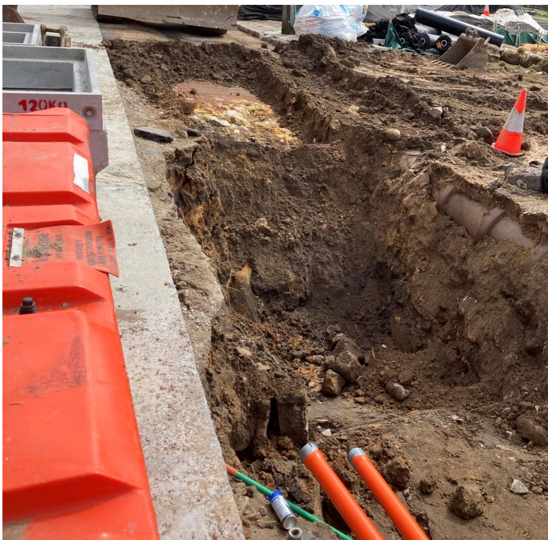
Figure 3.23: Trench for a garden bed in WZ3D showing the exposed bedrock at the top of the trench, a service pipe on the right and the steep natural benching of the bedrock.
