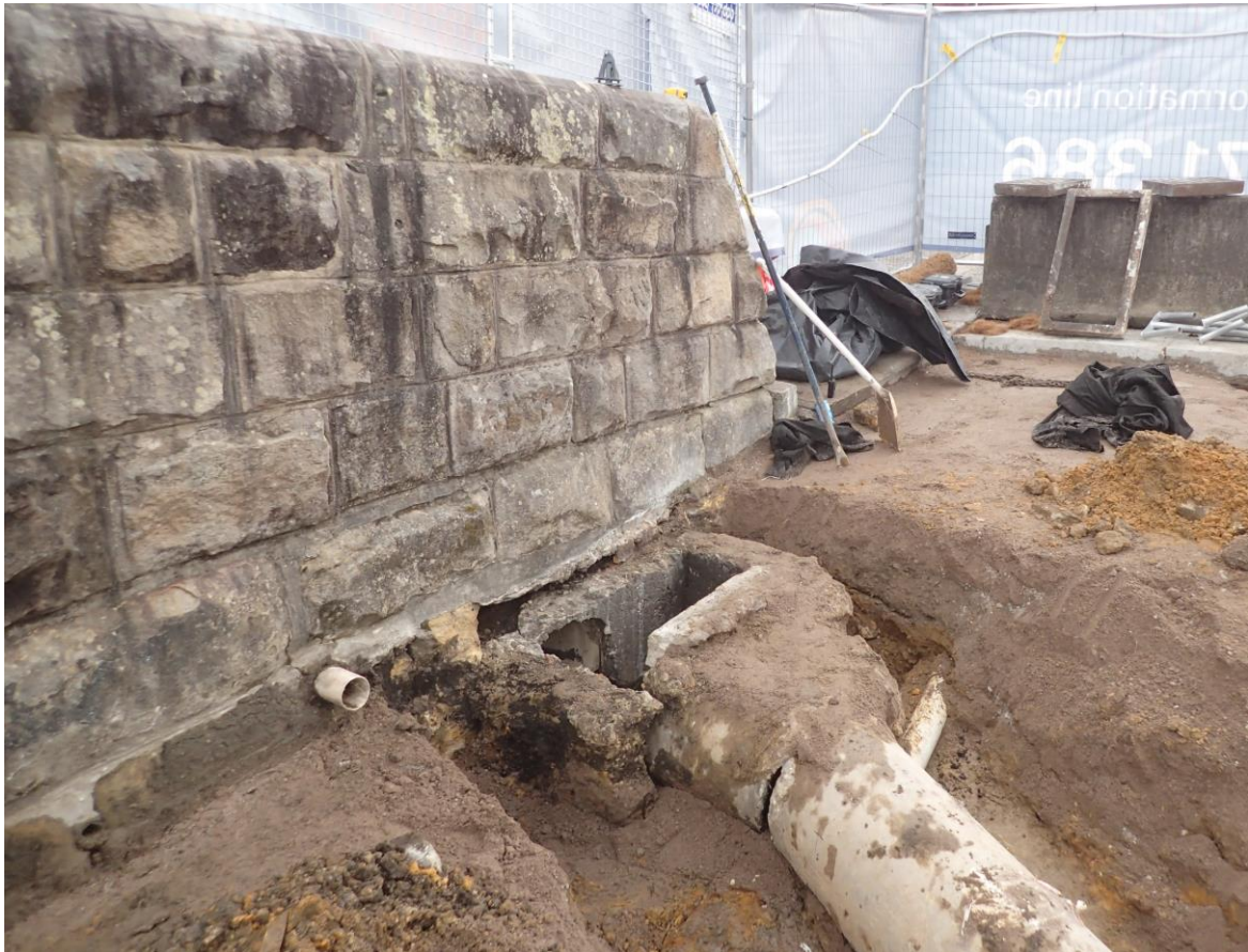
Figure 3.25: The concrete drain and connecting pipe laid under the northern most section of the heritage wall.
