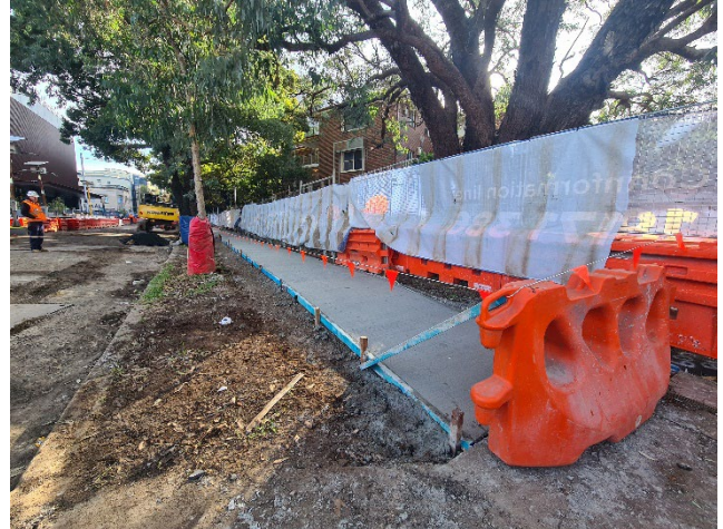
Cope St Site Compound: New concrete footpath pour completed on north-eastern end of Cope Street.
