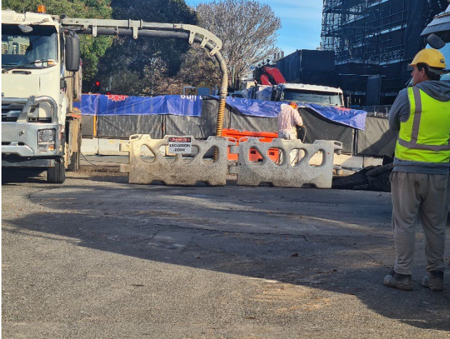
Wellington St/Cope St intersection: Investigation works underway. Full closure of Wellington St/Cope St intersection commenced on 19/06/2024 - 28/06/2024 for stormwater works (standard construction hours).
