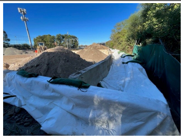
Improvements to stockpiling practices noted at Belmore Triangle.
