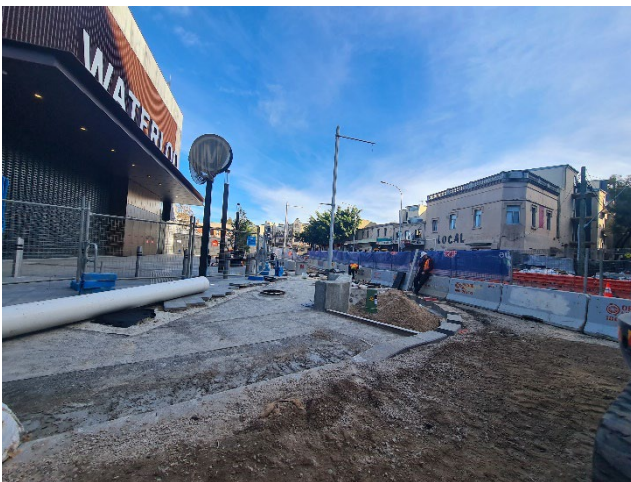
Cope St Site Compound: Kerb and gutter works underway; with grates being installed on drains. Refer action raised under ER Inspection Section of Report.
