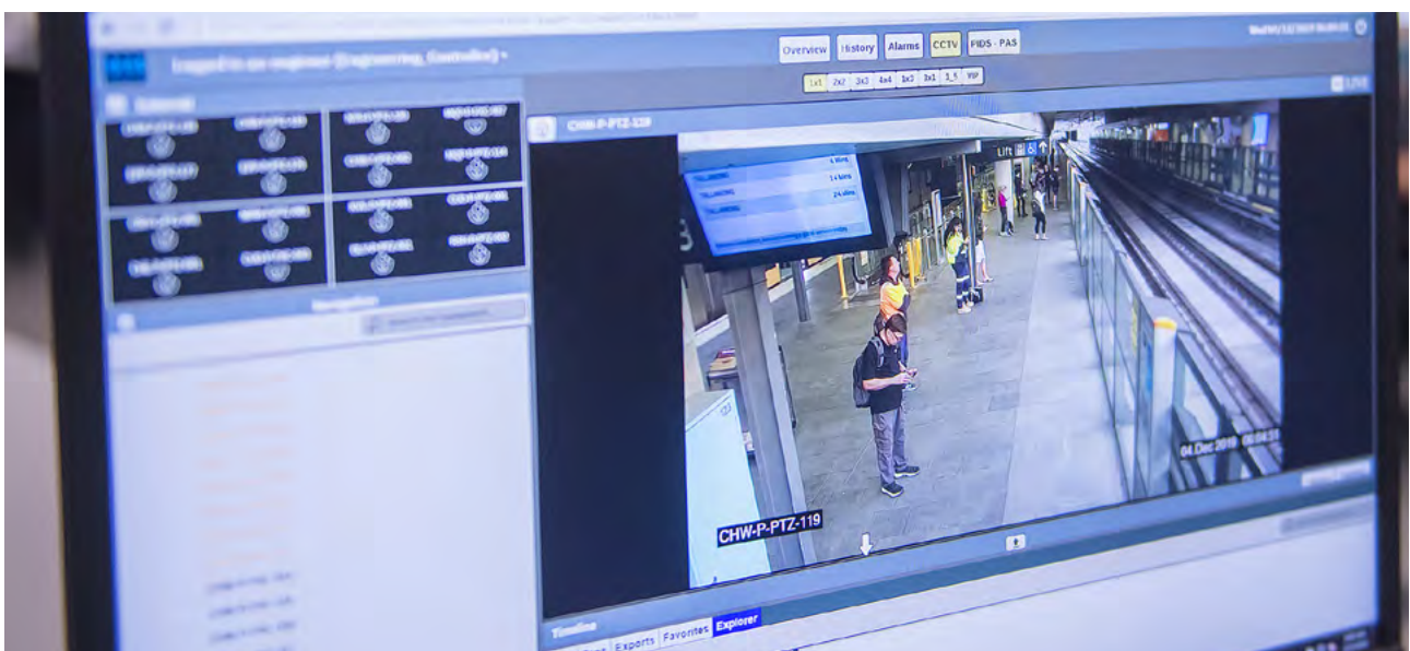
Expert train controllers work in a state-of-the-art Operations Control Centre at Tallawong.
