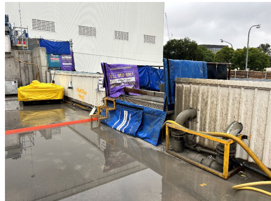
Figure 2.2: Westmead site – Acoustic shed with noise blankets over stairs and concrete shoot
