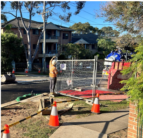
Figure 4.1: Westmead Utility Works – Open excavation on the Cnr Hassell and Bailey Streets
