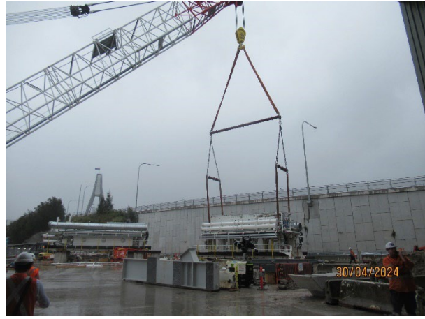
Figure 3.8 The Bays: Loading of new segments of the TBM into the station box.
