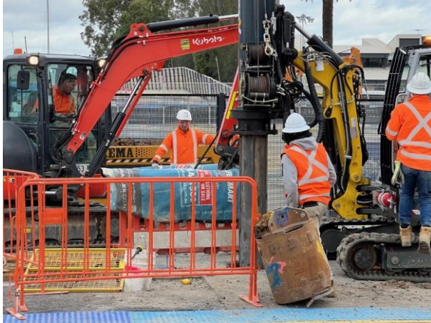
Platform 3/4 - Noise blankets were set up around the hammer to minimise noise
