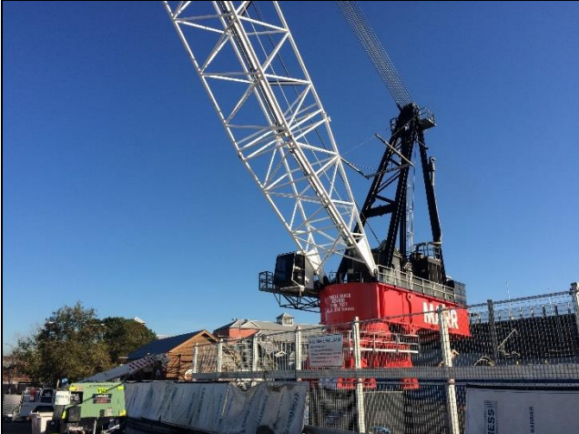
St Marys north west view north west – Erection of tower crane completed.
