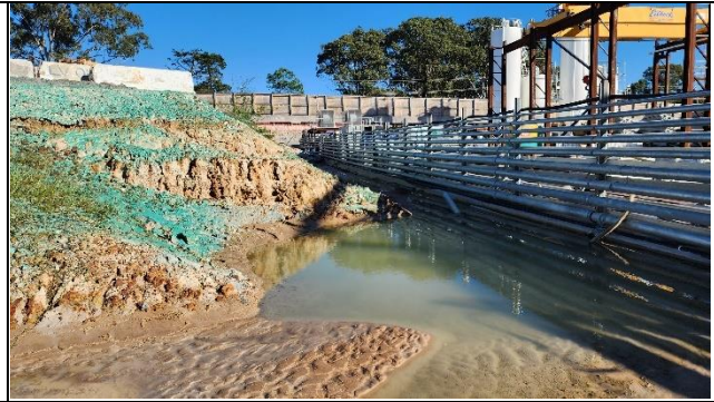
ORH –The ER re-emphasised that the removal of accumulated sediment was required on the SBT boundary as part of the site ERSED maintenance.
