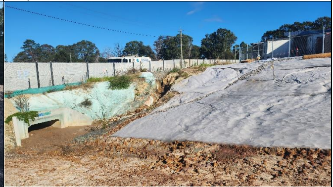
ORH – Maintenance of ESC and removal of sediment from internal swale was outstanding.
