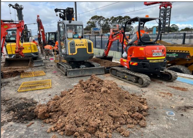
Platform 1/2 - Spoil was placed adjacent to the backfill location, with black plastic to be installed as a contingency if it should rain
