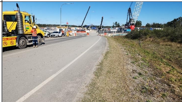
AEC – Site entrance shared with SBT, minor tracking was observed and organised the removal of tracked material.
