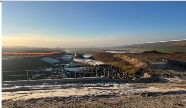
SCAW / M12 Interface - The large basin has been completed and revegetation is progressing well
