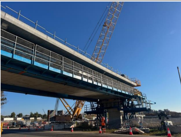
Patons Lane - The gantry has crossed Patons Lane and installed the precast elements out of hours under road closures
