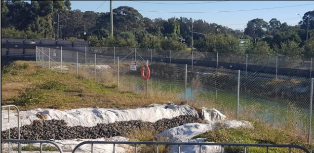
Claremont Meadows view north west – Northern basin and inlet swale well maintained.
