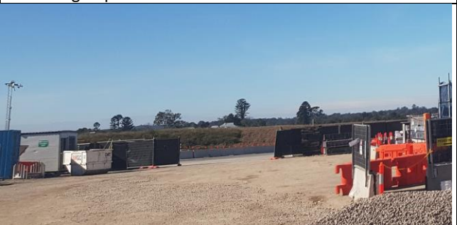
Aerotropolis view east to SBT access from SSTOM – TBM retrieval working/loading area.
