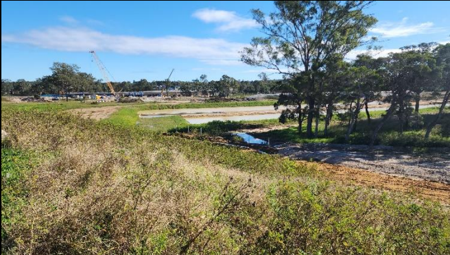
SMF – Tie in works with SCAW from the PLM sumps was discussed, noting that additional ERSED and stabilisation of the area was required.
