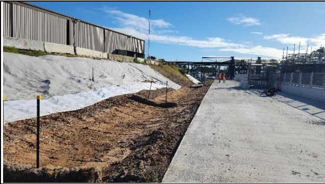
ORH – Maintenance of the ESC has been undertaken
