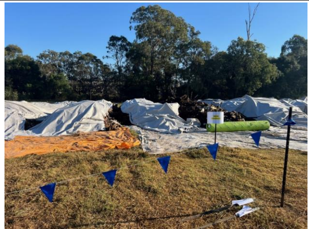
AEC 35 - Stockpiled material from AEC 35 is segregated awaiting testing results to determine disposal options
