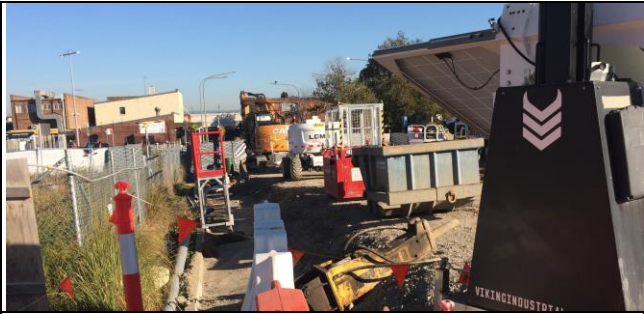
St Marys south side of Station St view west – road-base level working/loading area pad installed on Station St.
