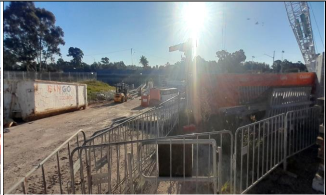
Claremont Meadows view west – Eastern noise blankets extended south for OOH concrete deliveries per DNVIS.
