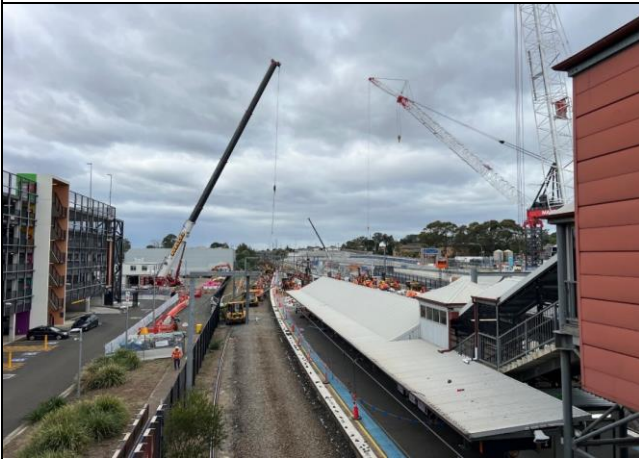
Overpass - Works were congested as Sydney Trains were operating adjacent to FSM
