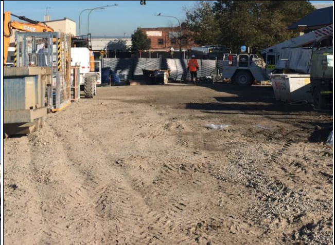
St Marys Station St view west – road-base level working/loading area pad installed on Station St.
