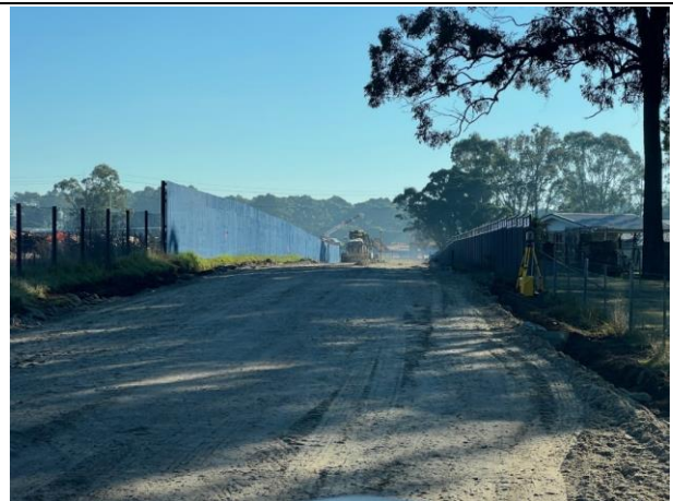
Lansdowne Rd - Work has commenced on the haul road, open communication has been maintained with the resident
