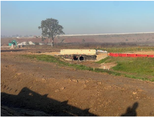
Main Haul Rd - A temporary crossing has been installed across the water channel
