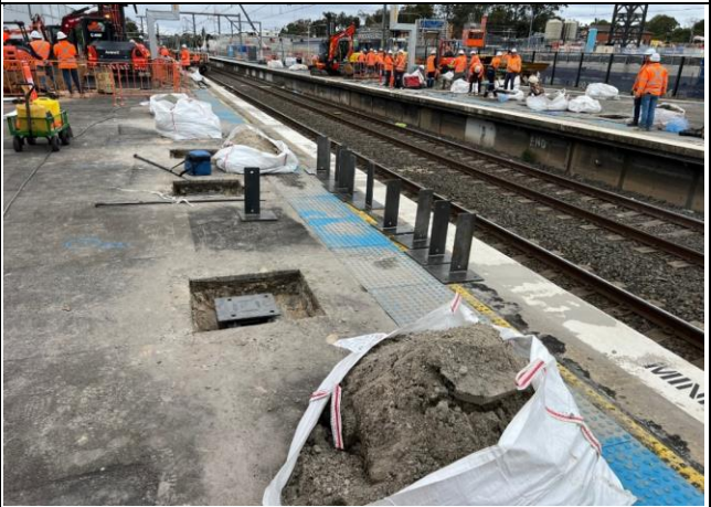
Platform 1/2 - Excavations were made to allow the installation of the hoarding brackets
