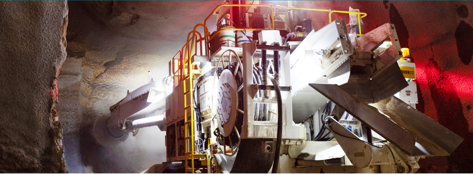
Roadheaders are being used to excavate the station cavern at Pymont Station.
