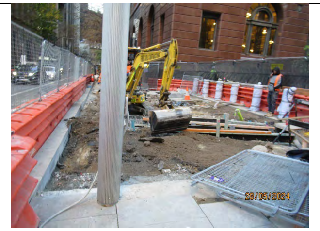
Martin Place: Ongoing works on utilities within water filled barriers adjacent Castlereagh Street.
