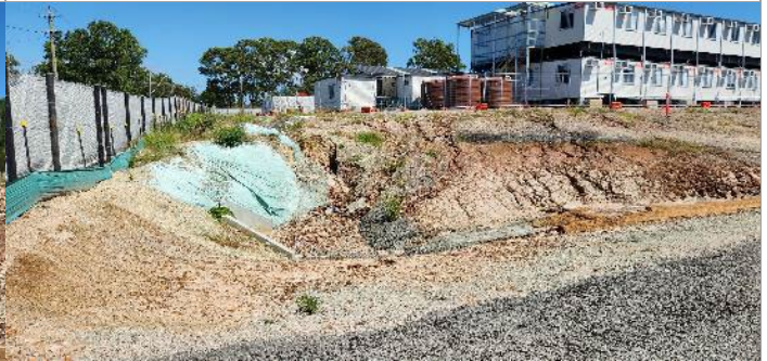
Photos 33-34: Localised scouring occurred due to recent heavy rains
