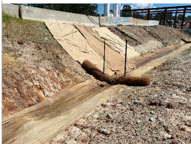
Photos 28-29: Erosion control devices in place
