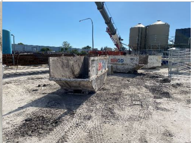
Photo 22: waste bin area found to have dirt/dust build up
