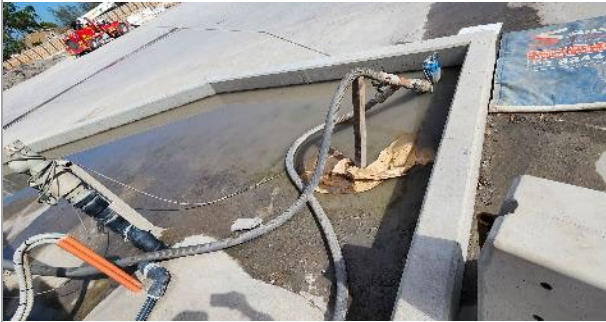
Photos 17-18: bunded areas with stormwater ponding
