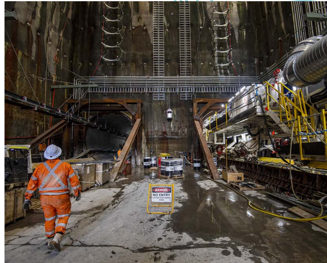
Tunnelling in progress: Part of the 11-kilometre twin tunnels from The Bays to Sydney Olympic Park.
