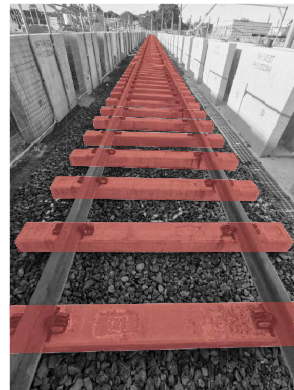
Geopolymer concrete sleepers with 60% lower carbon footprint than standard concrete sleepers at a Sydney Metro maintenance facility.
