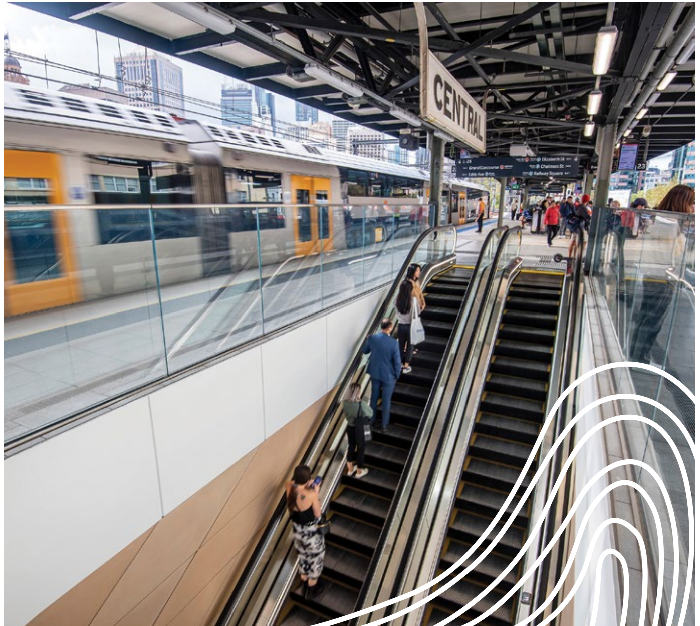
In preparation for Metro services at Central Station escalators have been installed to provide convenient access to suburban platforms.
