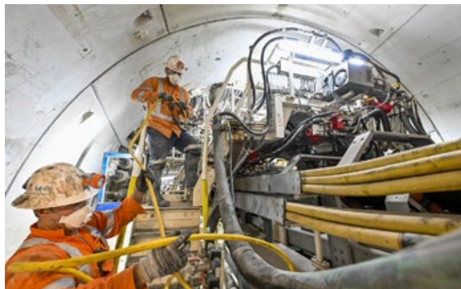
Segments are being installed in the Sydney Metro Airport Business Park tunnels.
