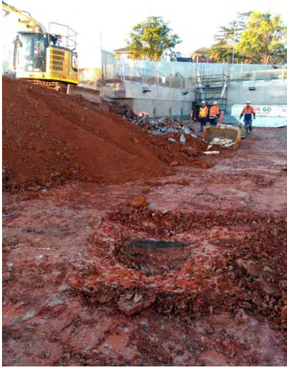
Figure 5.18 The base of the second well as exposed during excavation of the Dive.
