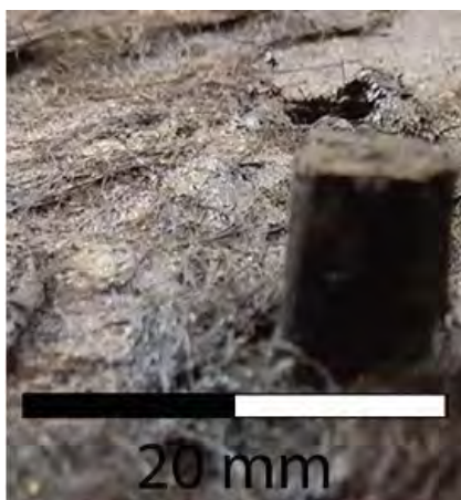
Figure 5.33: Old nail hole plugged with wooden plug. (Source: Fiedler, K., 2016)
