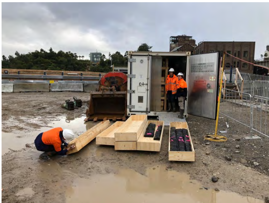
Figure 2.26: Crates for loose timbers prepared for being shelved inside the refrigerated container.
