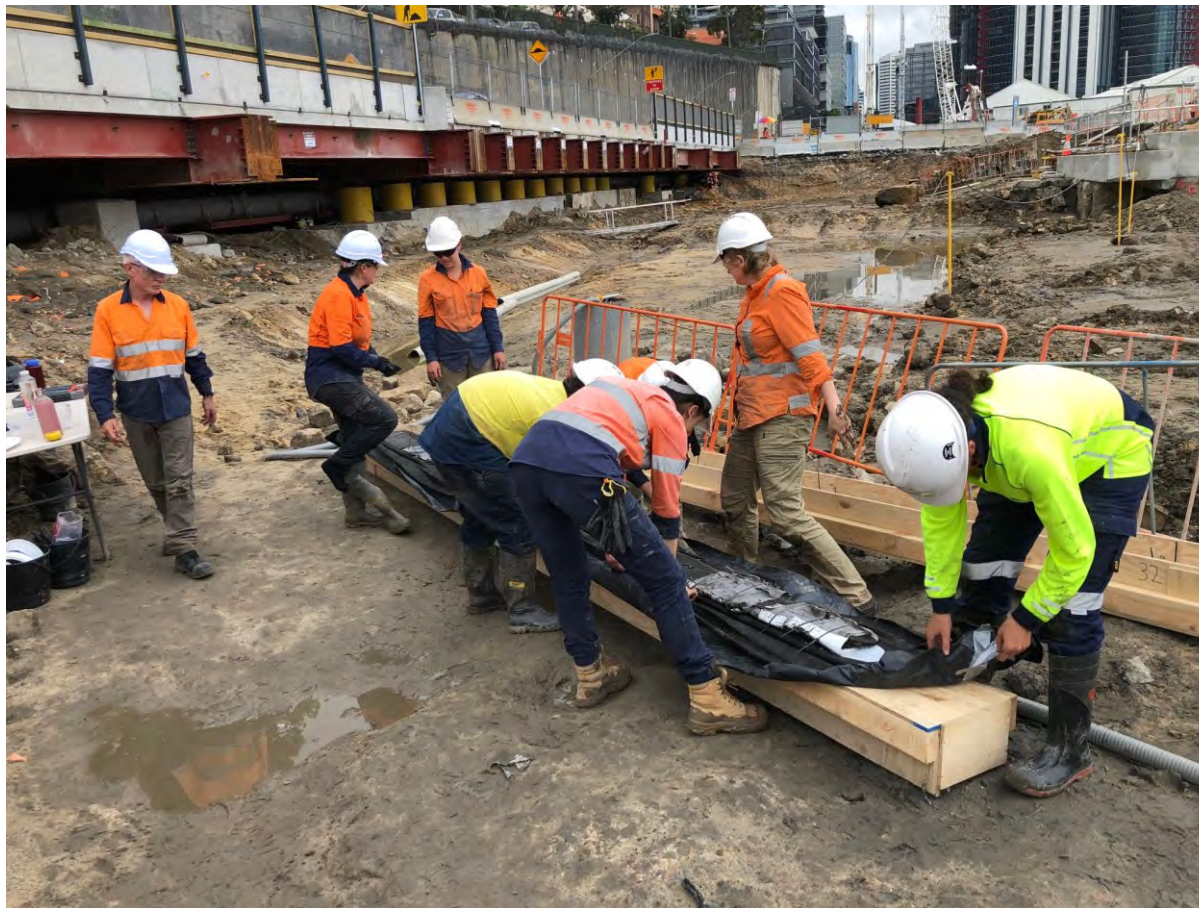
Figure 2.16: Ceiling planking being wrapped before being placed into a custom-made crate (in background) with upside down and unused crate being used as a work table. Note that a layer of geotextile and black plastic had already been placed onto the board before the plank was slid on. This allowed for the element to be wrapped without it being moved for a second time.
