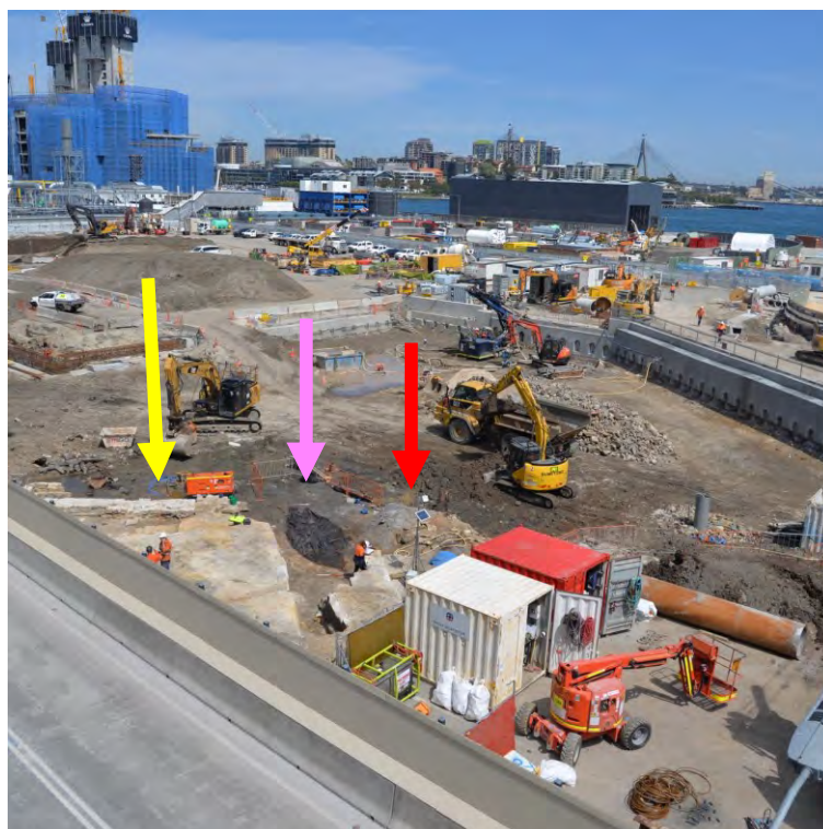
Figure 3.2: View of UDHB1 (pink arrow) looking to the south west. Hickson Road in foreground. Remains of Langford's house (yellow arrow) and location of Cuthbert's sawshed (red arrow). (Source: Casey & Lowe).
