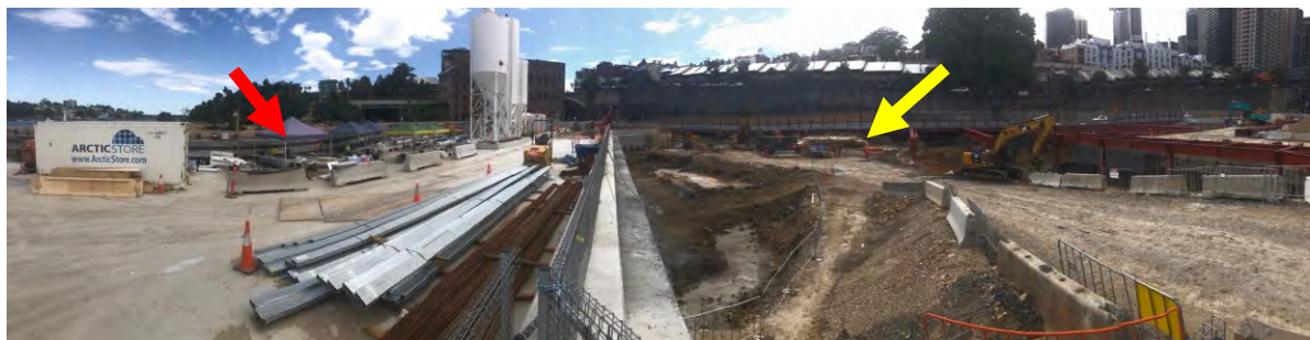
Figure 2.52: Relocated and larger processing area (red arrow) within the construction site which was around 100 m away from the boat (yellow arrow). Note the refrigerated container to the left of the image.
