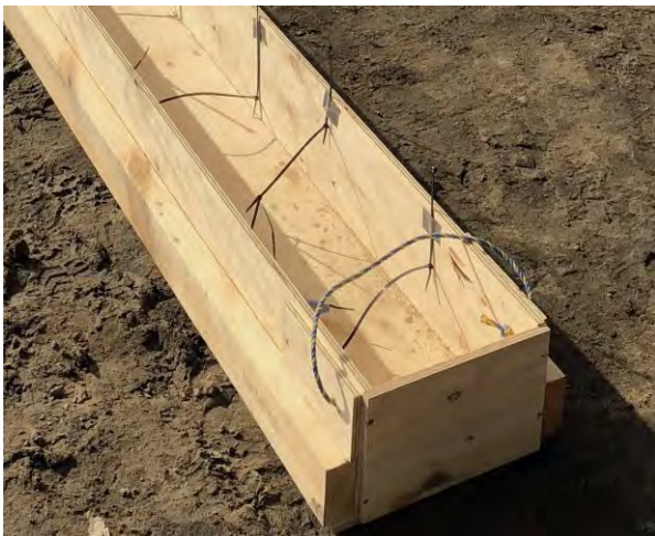
Figure 2.24: Crate made on site for the ceiling planking. Note the cable ties stuck to the inside of the crate to better secure the contents.
