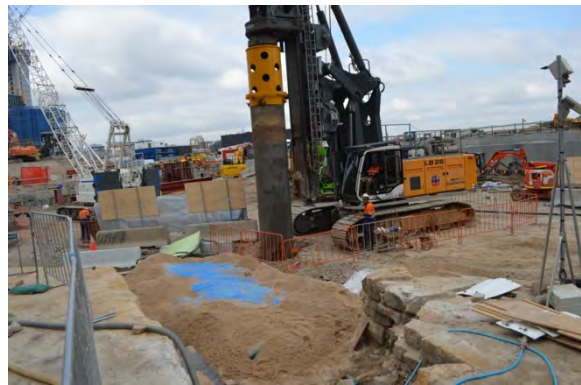
Figure 2.44: Construction works adjacent to wreck during temporary in situ protection. (Source: ICS).
