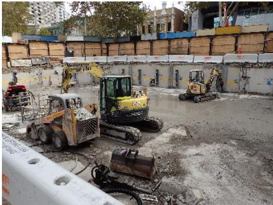
Figure 4.11 View north-west to the corner of Miller and Berry Streets of the basement to the north of 187 Miller Street.
