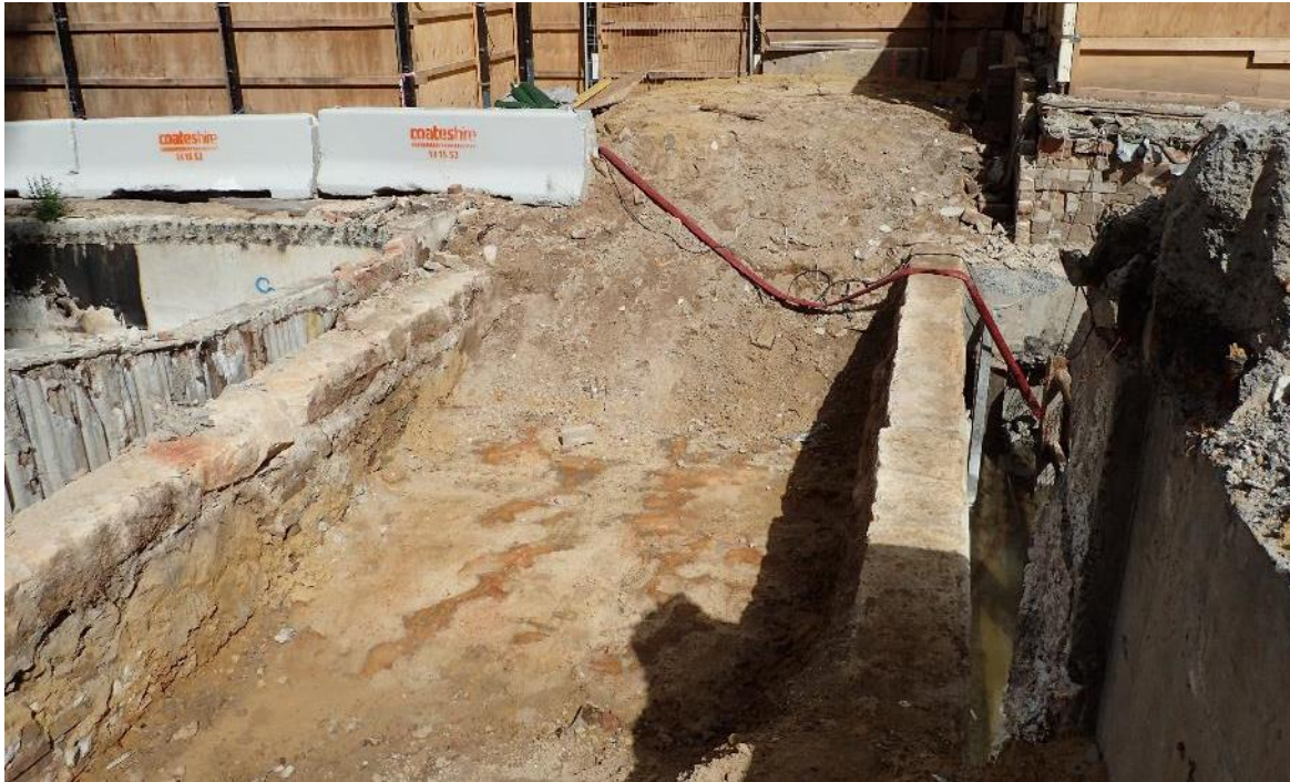
Figure 4.15 View west along the narrow 'land bridge' that was 187 Miller Street. Note that the 187 property is protected from collapse into the basements to each side by a supporting wall.
