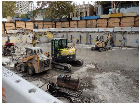
Figure 4.12 View south from 187 Miller Street. The depth of the basements descending to three levels and 8m below street level was such that no evidence of wells survived.
