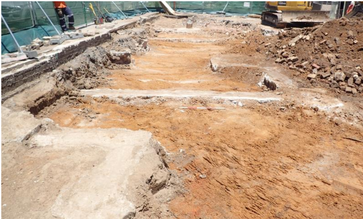
Figure 3.15 View west, showing the twentieth century foundations retained in the B Horizon, post-removal of nineteenth century foundations (13 December 2017).
