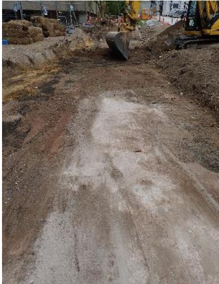
Figure 4.3 View north along the eastern section of the site showing a concrete surface and introduced fills, perhaps dating to the 1970s. Note the depth below pre-existing ground level.
