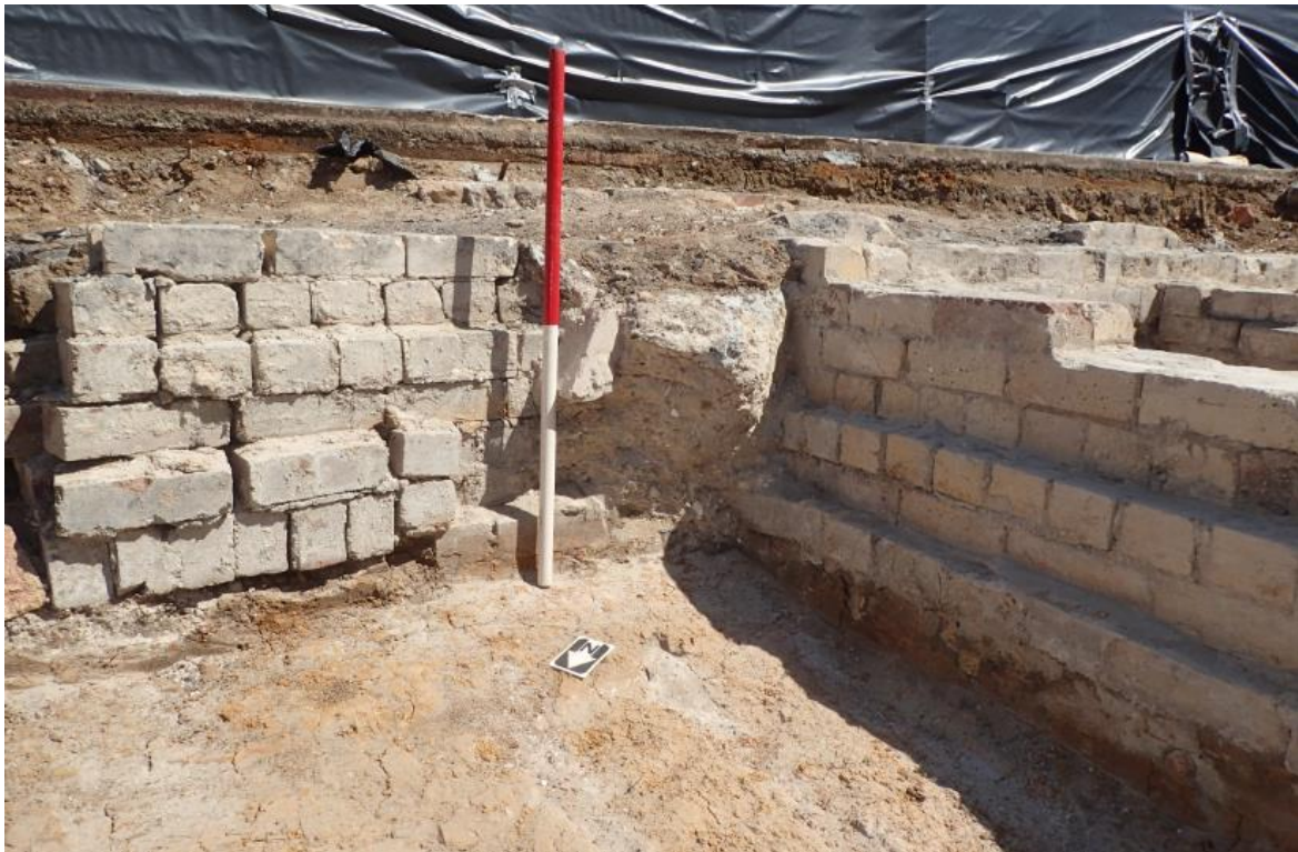
Figure 3.12 Northern elevation of nineteenth century brick walls [0012] and [0014] truncated by concrete foundations [0017] (11 December 2017).
