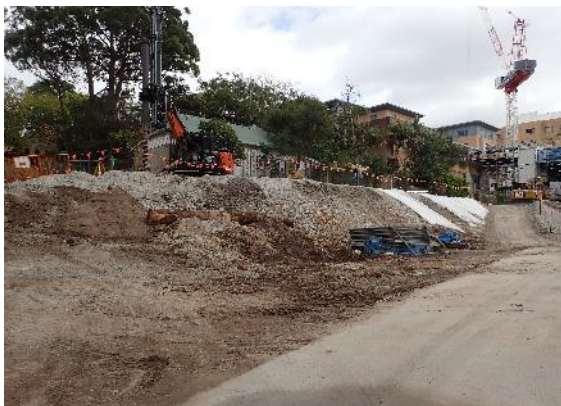
Figure 4.5 The Victoria Cross north site from the haul road to McLaren Street which has removed a substantial depth of soil as a part of works undertaken prior to the Sydney Metro project.
