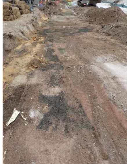
Figure 4.4 Second view north along the eastern section of the site showing a concrete surface and introduced fills, perhaps dating to the 1970s. Note the depth below pre-existing ground level.
