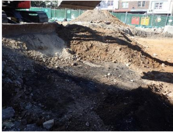
Figure 3.18 View south of contaminated coal tar deposit.
