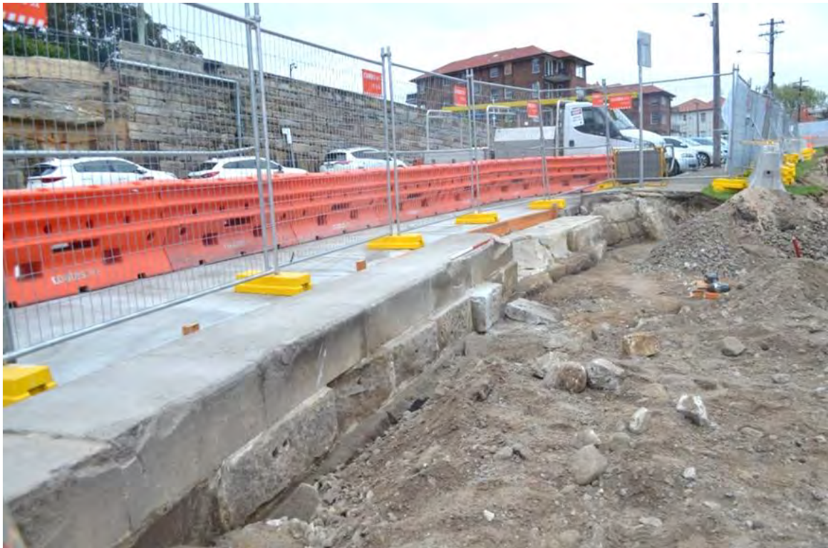
Figure 4.115: Different phases of sandstone seawall along the edge of Blues Point Road. The upper row of dressed blocks formed the edging of the present-day footpath and was bonded with concrete to the lower courses. The grey sandy rubble fill abutting the wall to the east is context (329). View to northwest, 1m scale. DSC_4921.
