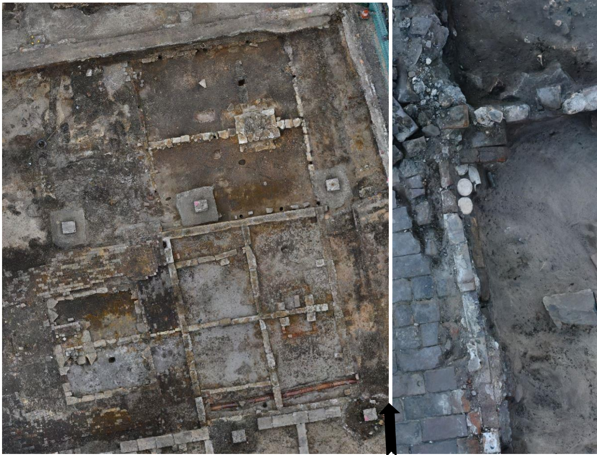
Figure 3.4 Houses at 53–59 Botany Street illustrating variations in the quality of the foundations (left). Detail of the stout bottles forming part of the foundations for 79 Botany Street.
