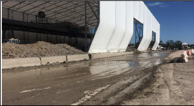
Orchard Hills view north: Internal spoil haul road in poor condition and requiring repairs.
