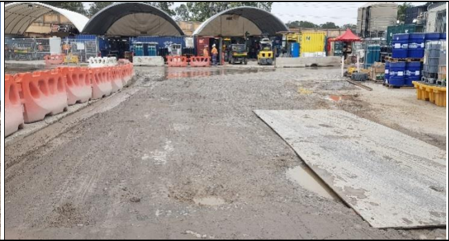
Orchard Hills view west: Internal spoil haul road in poor condition and requiring repairs.
