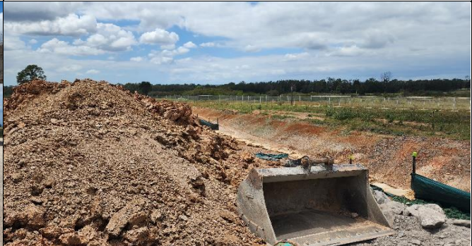
AEC – Preparation for the diversion of the clean water swale. Noted that damming of the swale would occur while the diversion works occurred.
