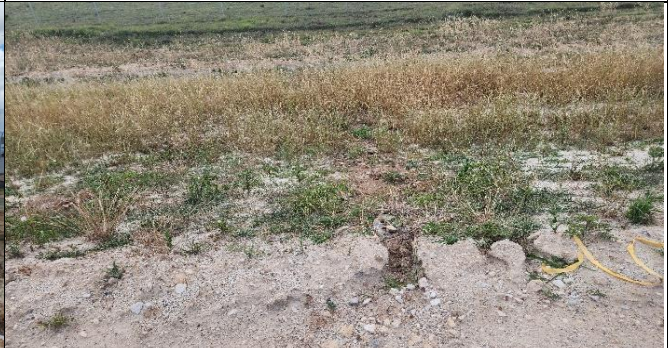
SMF – Minor scouring of the batter was noted and weed maintenance was discussed with PLM.
