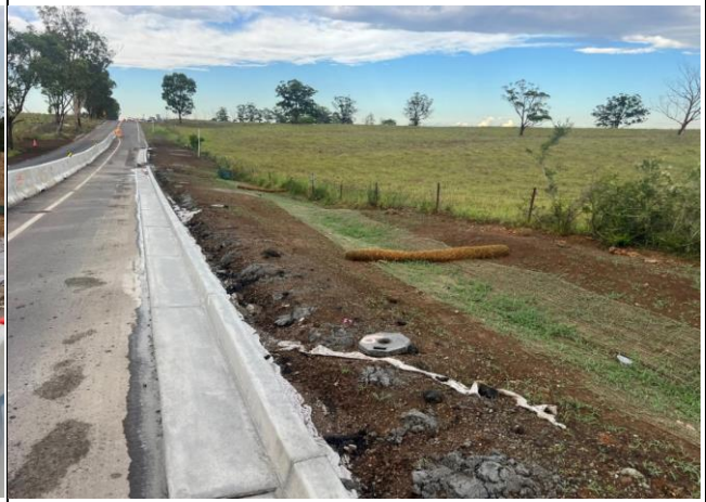
Roundabout - The drainage lines have been jute matted and seed applied, this is good practice
