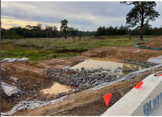
Elizabeth Drive Haul Road - The culvert is being worked and a small retaining area has been left for water to collect
