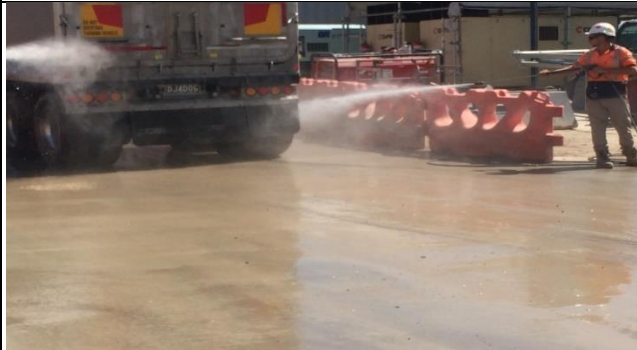
Orchard Hills south: Manual wheel washing prior to, and supplementing, automated wheel wash.
