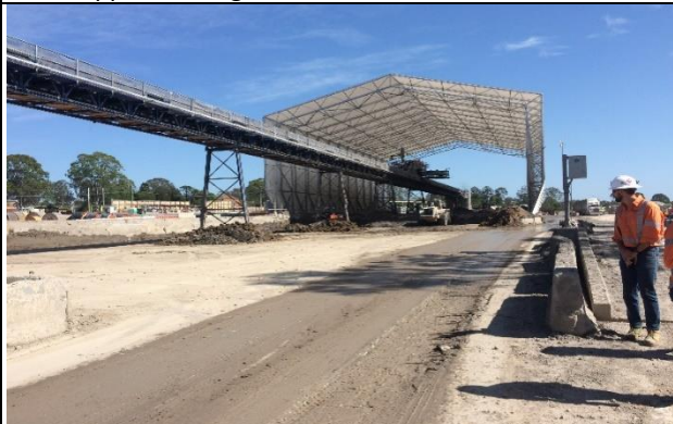
Orchard Hills view northwest: Management of tunnel spoil storage area significantly improved.
