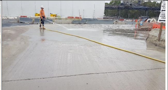
Orchard Hills exit: Greater frequency of washdown needed to minimise tracking onto Kent Rd.
